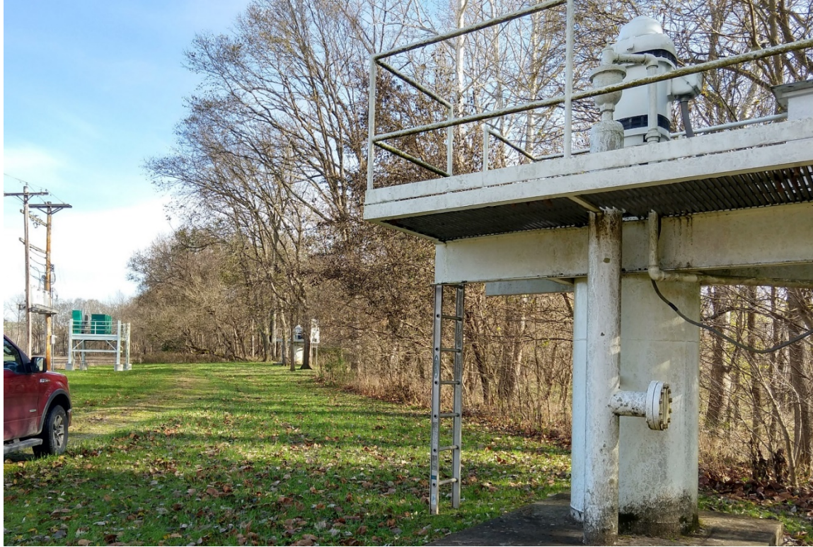
Wells located along Whitewater River, standby generator on platform at left
