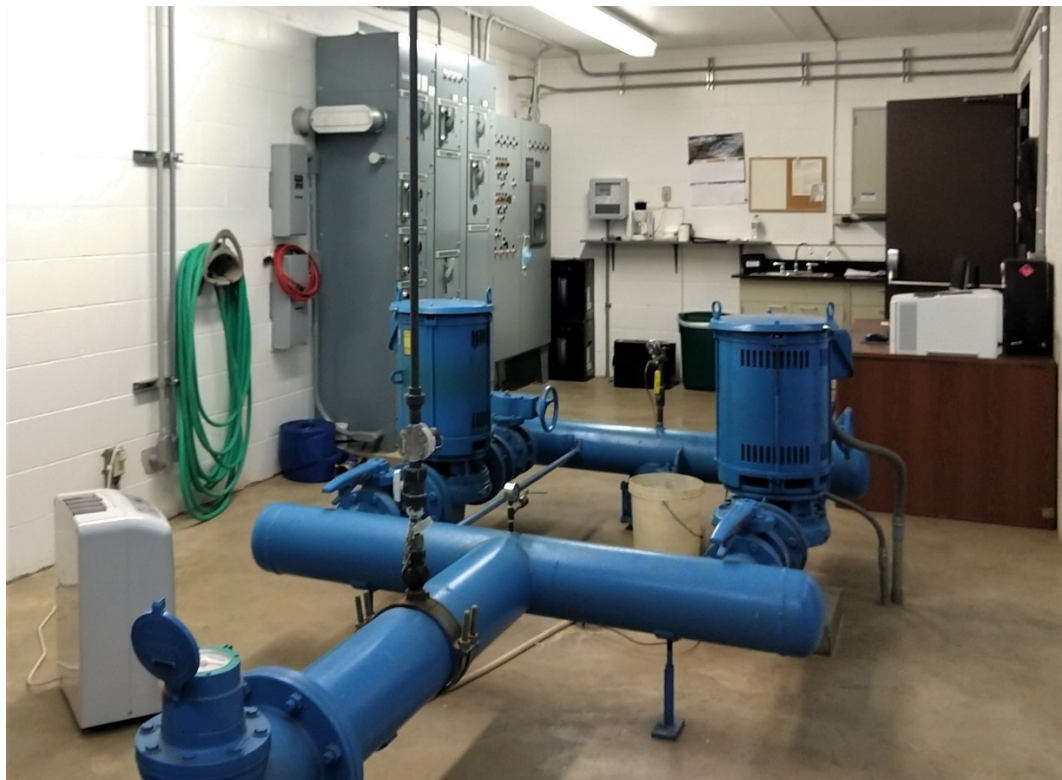
Plant interior showing high service pumps, control panel
