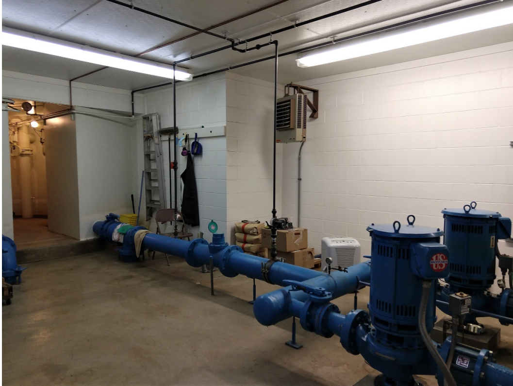
Plant interior, high service pumps on right, Aeralater on left
