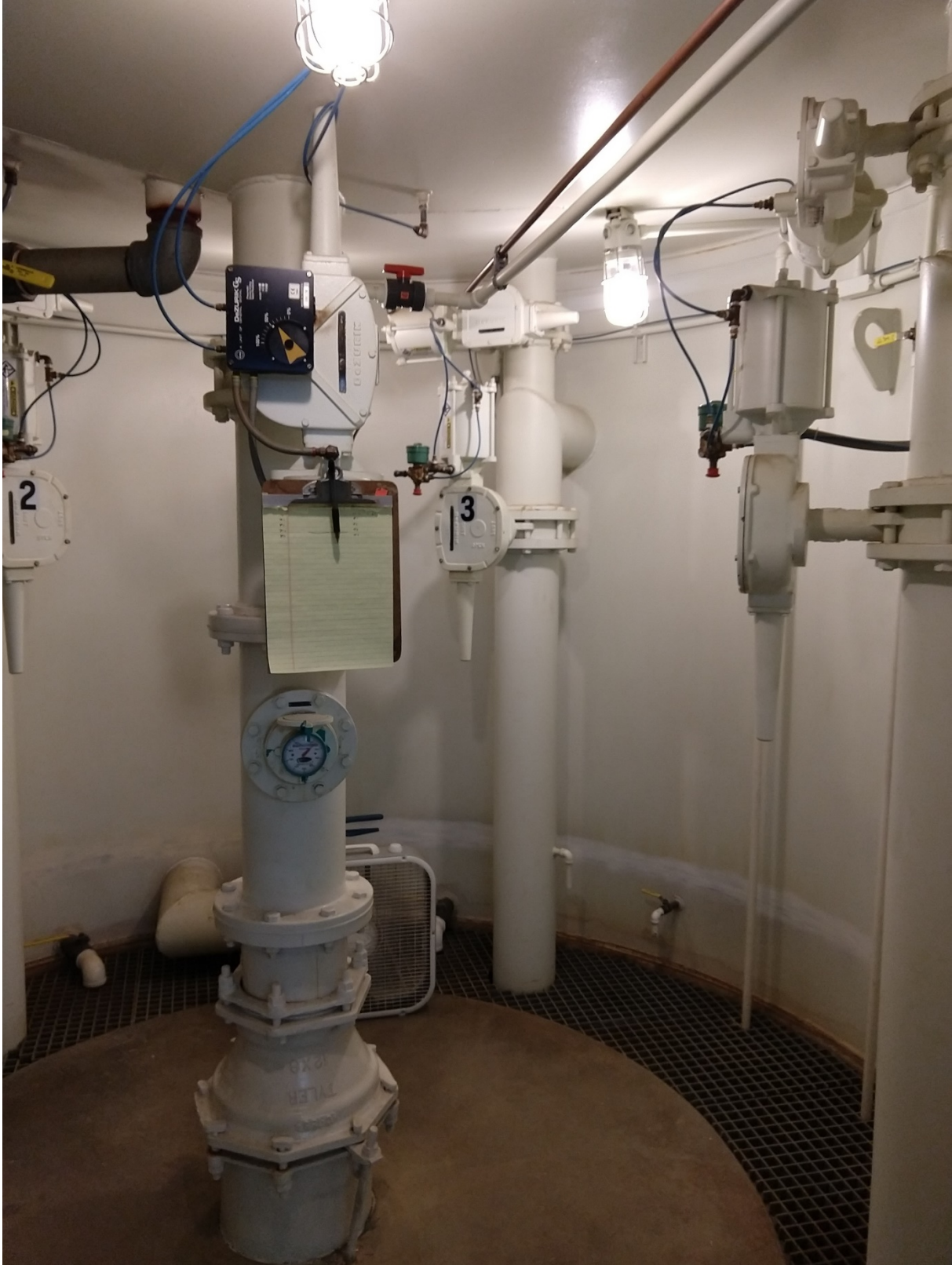
Aeralater interior, note lighter-colored repair seam towards bottom
