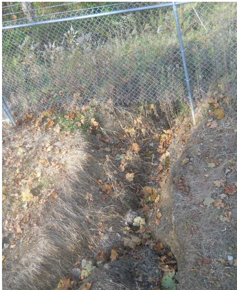
Figure 2 – Erosion under the property fence
