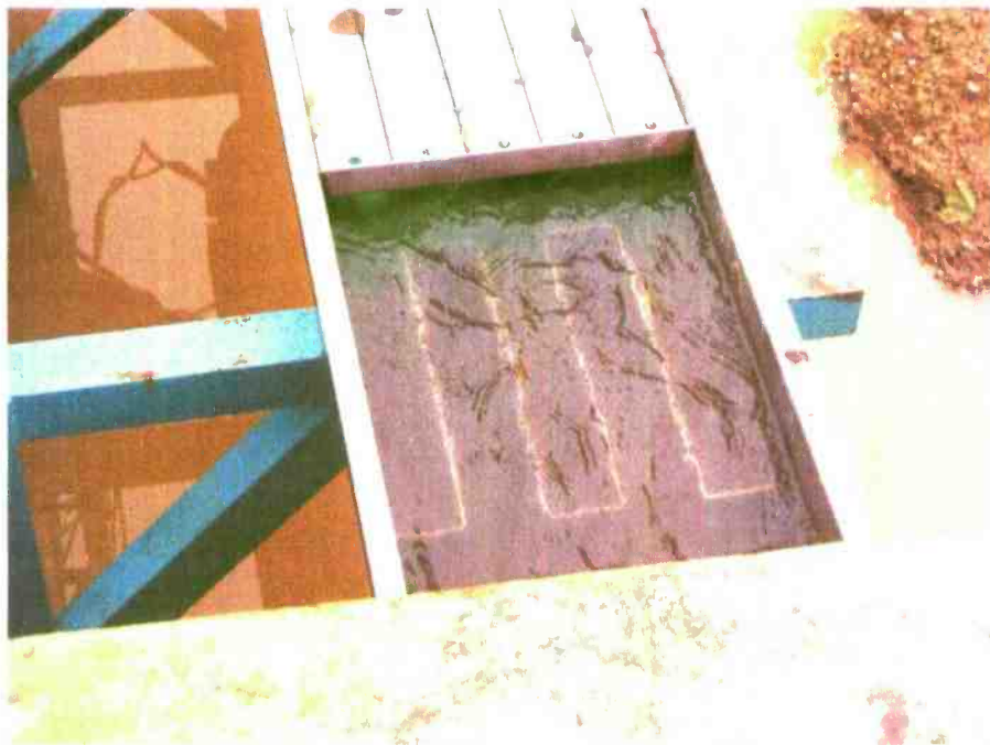
UV unit. Note the weirs are submerged 06
