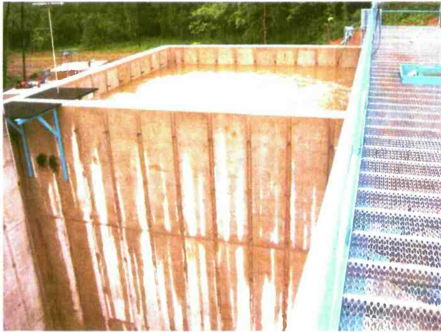
Digester (used for both north and south trains). See EQ/raw tank behind (2 pics) 05
