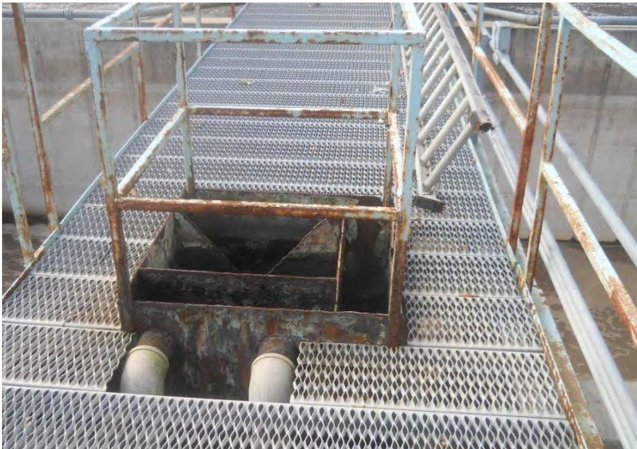
Figure 1 – Coating failure and metal corrosion on the Flow Splitter Structure
