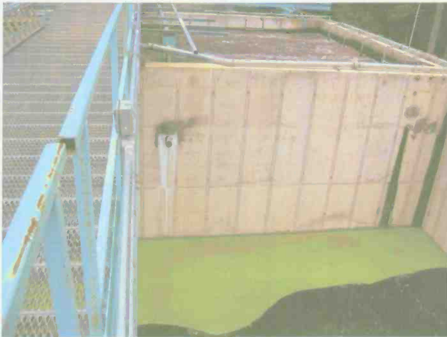
Sludge holding tank (bottom of pic). Note scum line (top center of pic)
