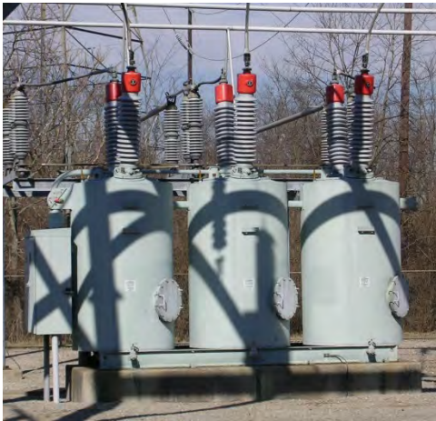
Typical Transmission Oil Circuit Breaker
