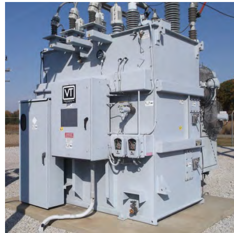
Typical Distribution Transformer
