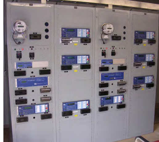
Typical Digital Relays
