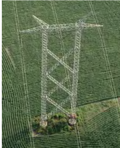
345 kV Aluminum H-Structure
