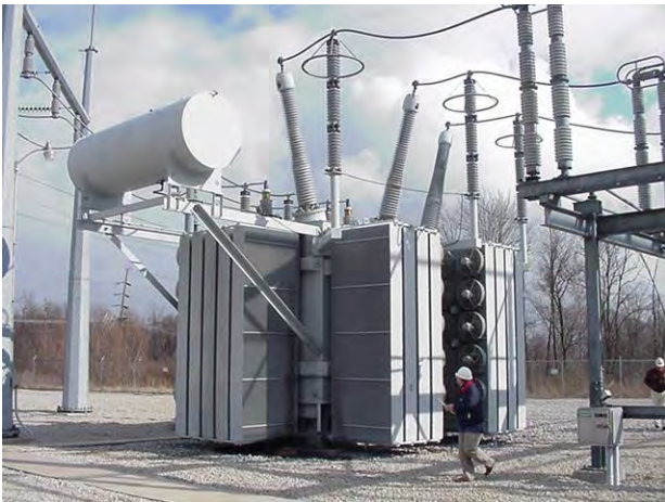
Typical Transmission Transformer
