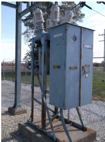
Typical Distribution Oil Circuit Breaker
