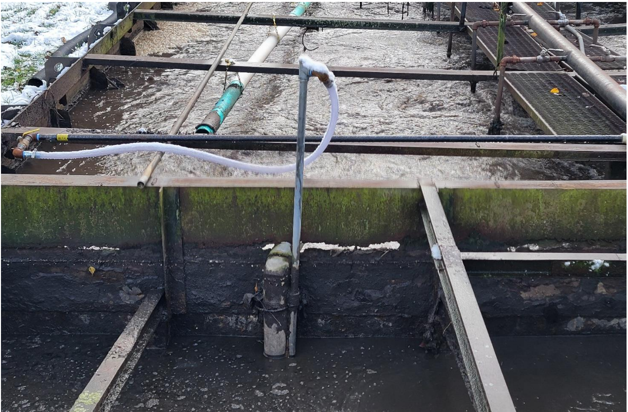
Fig. 6 – 2024 Photo - View SE of the corroded steel wall between the sludge tank (foreground) and aeration basins beyond. Applicant has inserted replacement pipe through the wall crack.
