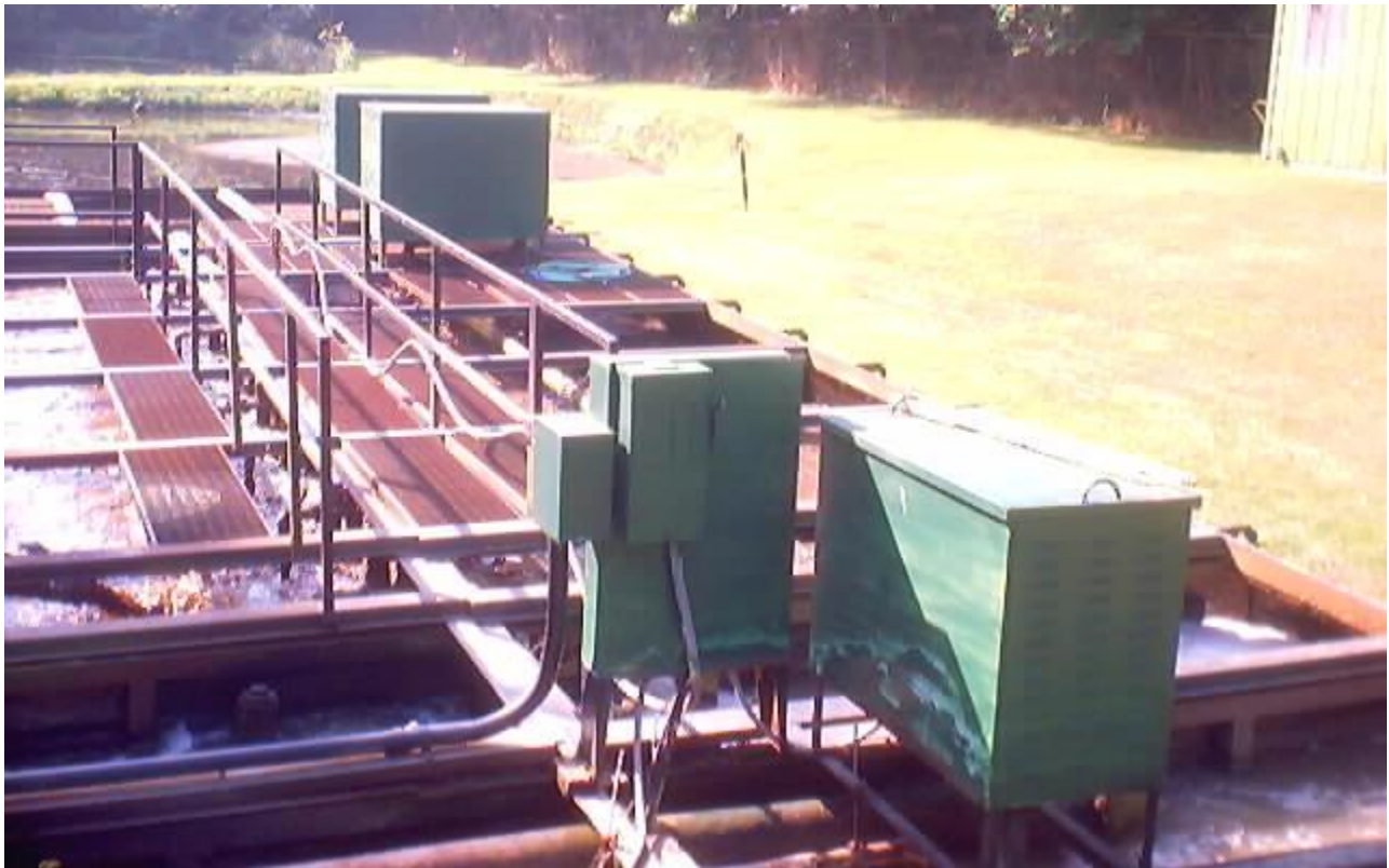
Fig. 9 – 2002 Photo – View looking south of the 1974 Package Plant of the surge tank, sludge tank, aeration basins (middle left), blowers and polishing ponds beyond.
