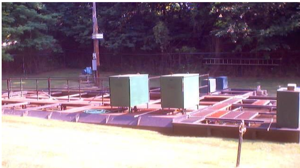
Fig. 11 – 2002 Photo – View N of the 1974 Package Plant aeration basins and blowers (center) and clarifiers (at right)
