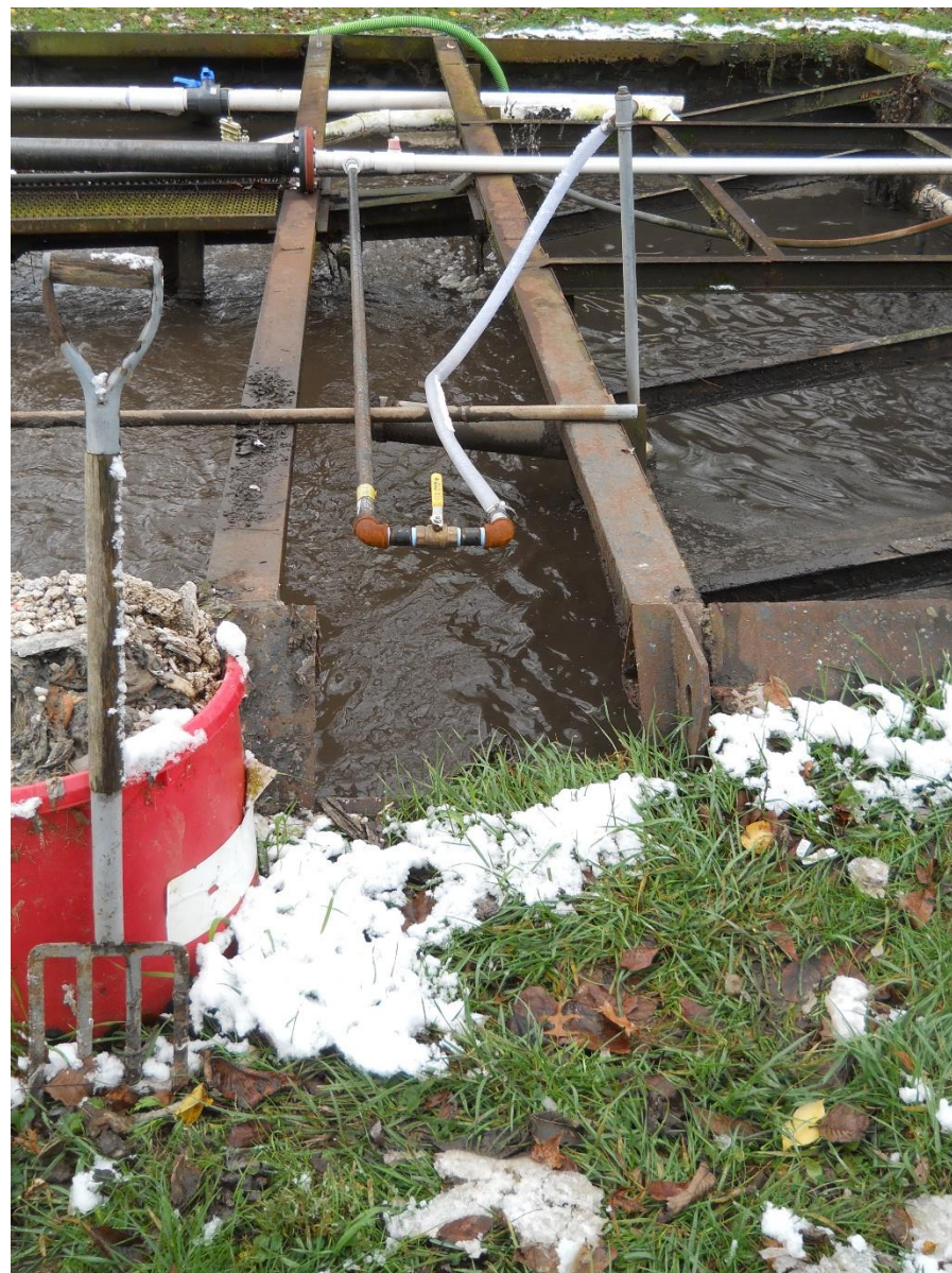
Fig. 18 – 2024 Photo View SW of notch cut out of the wall which allows overflows to exit the aeration basin and flow to the pond.
