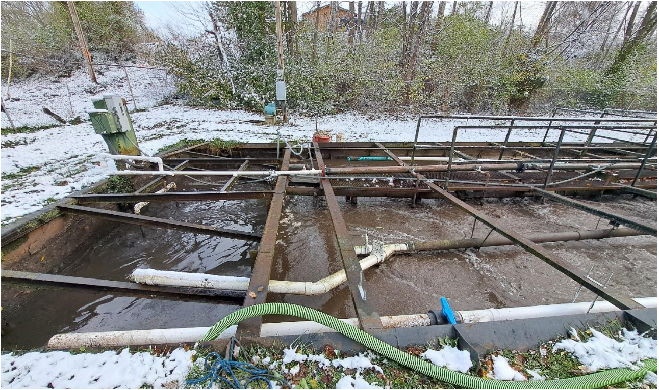
Fig. 5 – 2024 Photo - View NE of the 15,000 gal. sludge tank (left) and aeration basins (right)
