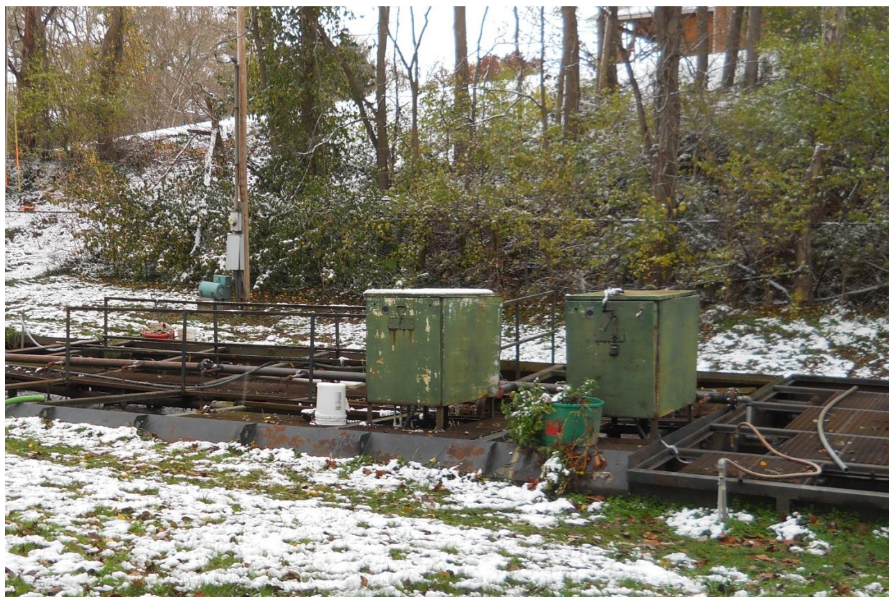
Fig. 12 – 2024 Photo – View N of the 1974 Package Plant aeration basins and blowers (center) and clarifiers (at right). Note the rust on the tank walls and grating.
