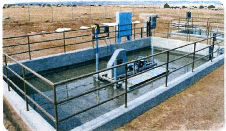
Overview of the AquaCAM-D ® unit in a SBR reactor.
