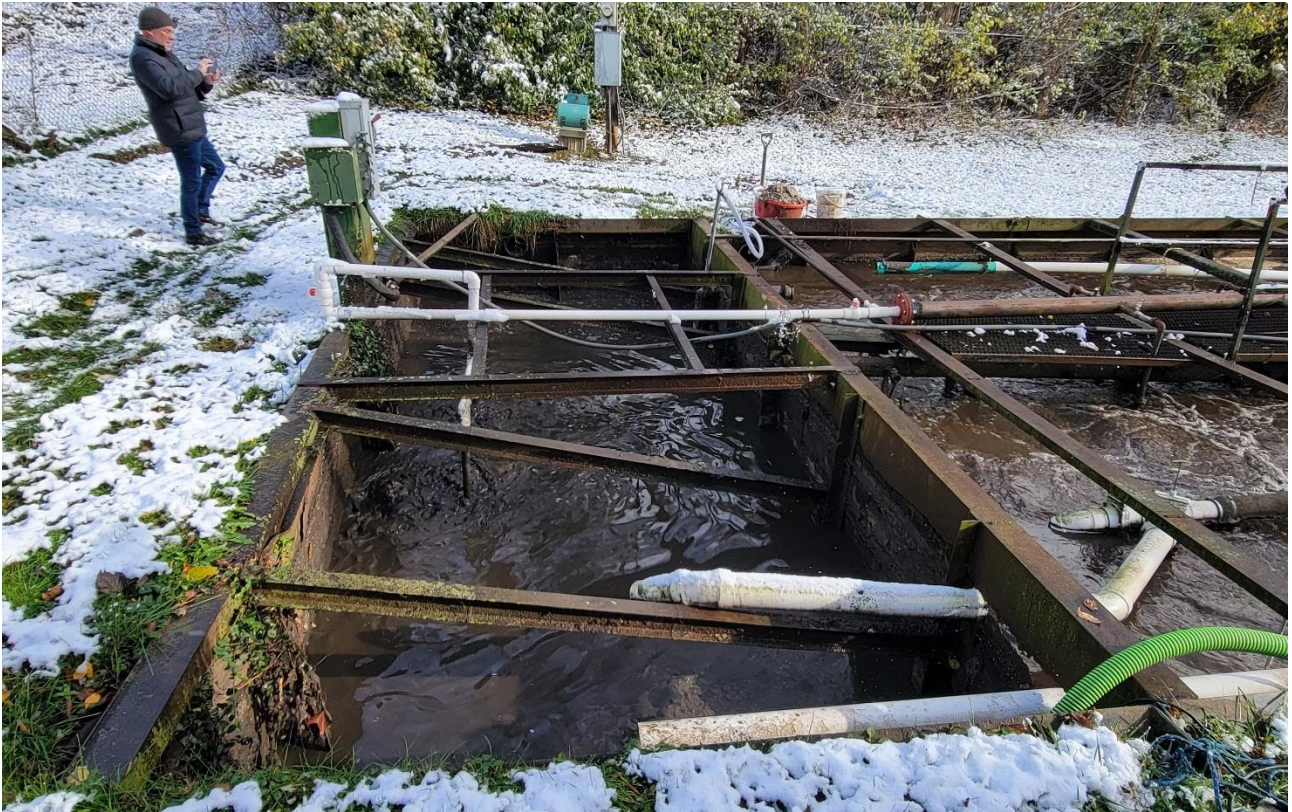
Fig. 7 – 2024 Photo - View of sludge holding tank showing rusted walls, piping through corroded wall cracks and bowed wall (at left).
