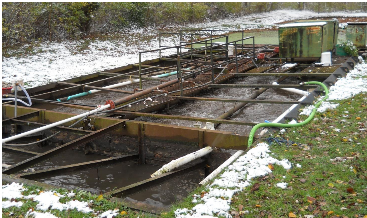
Fig. 4 – 2024 Photo of the 15,000 gal. sludge tank in front with two aeration basins (30,000 gallons each-center right) and blowers in upper right.
