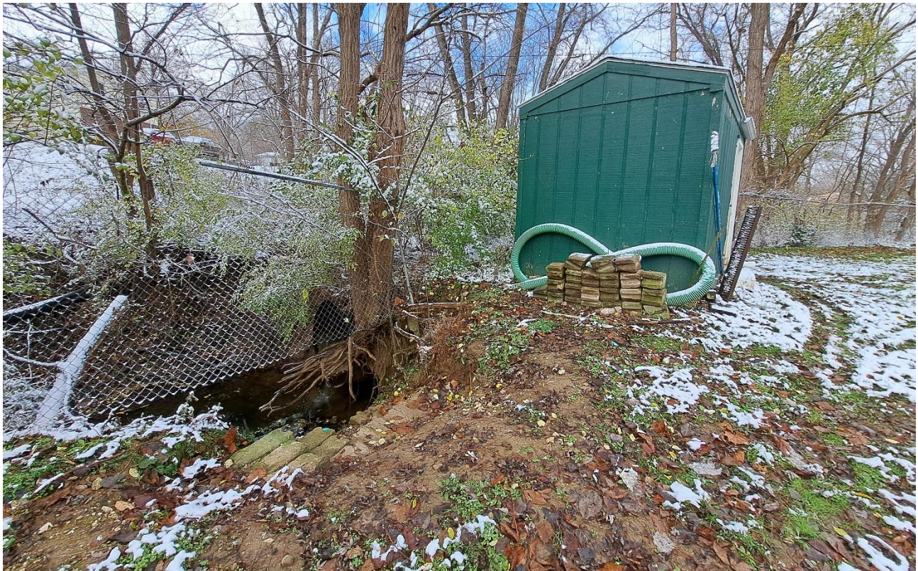
Fig. 22 – 2024 Photo – Outfall location with ground eroded at fence line.
