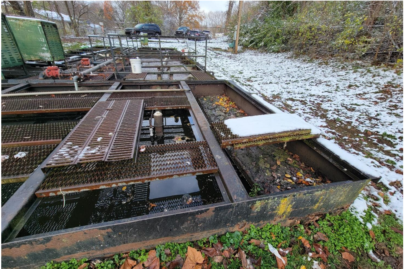
Fig. 15 – 2024 Photo - View NW of floating sludge along clarifier weirs and holes in wall at right.
