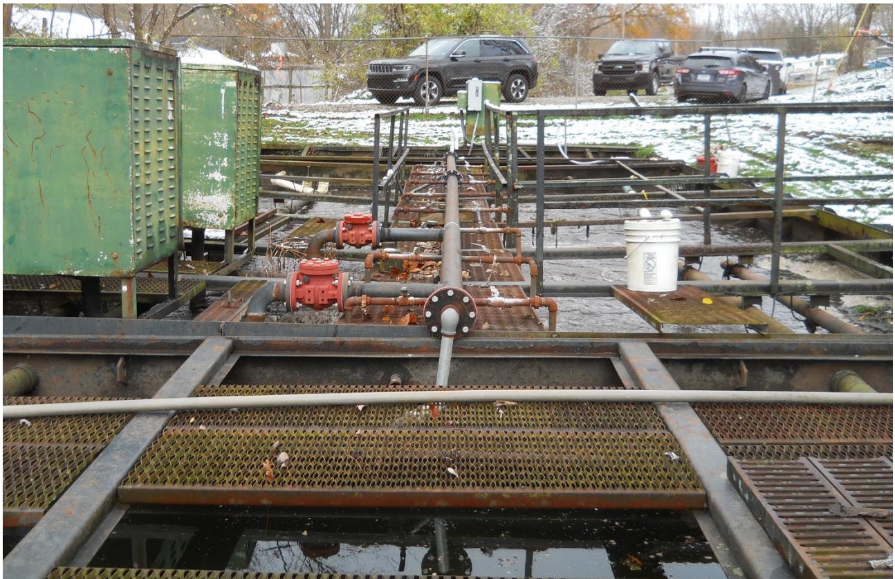
Fig. 10 – 2024 Photo – View NW showing the sagging center walkway and air header trip hazard.
