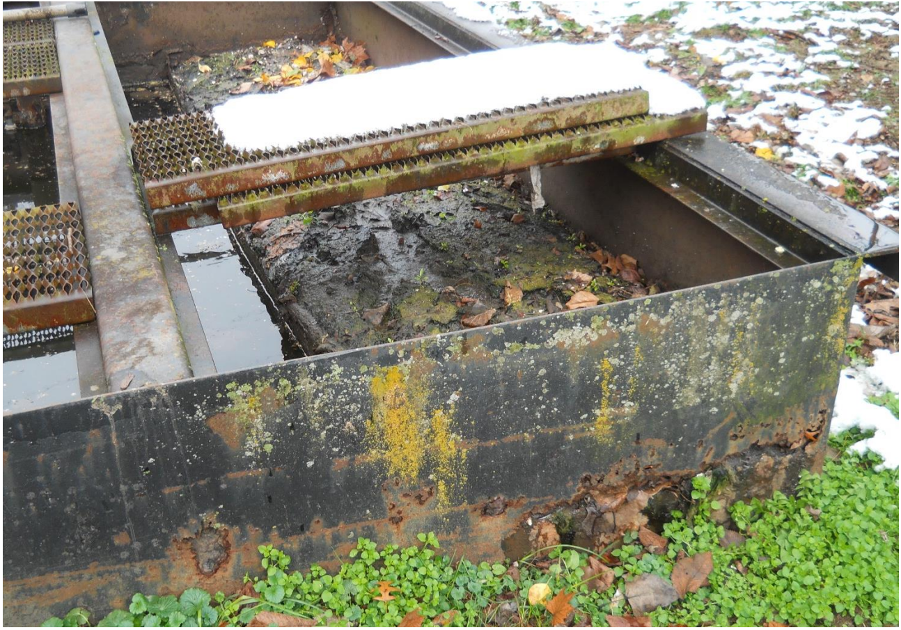
Fig. 21 – 2024 Photo - View of holes through tank wall at clarifiers.
