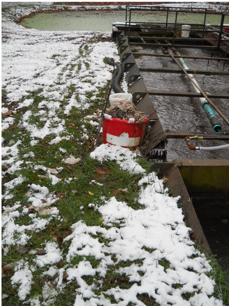
Fig. 17 – 2024 Photo View SE of notch cut out of the wall which allows overflows to exit the aeration basin and flow to the pond.
