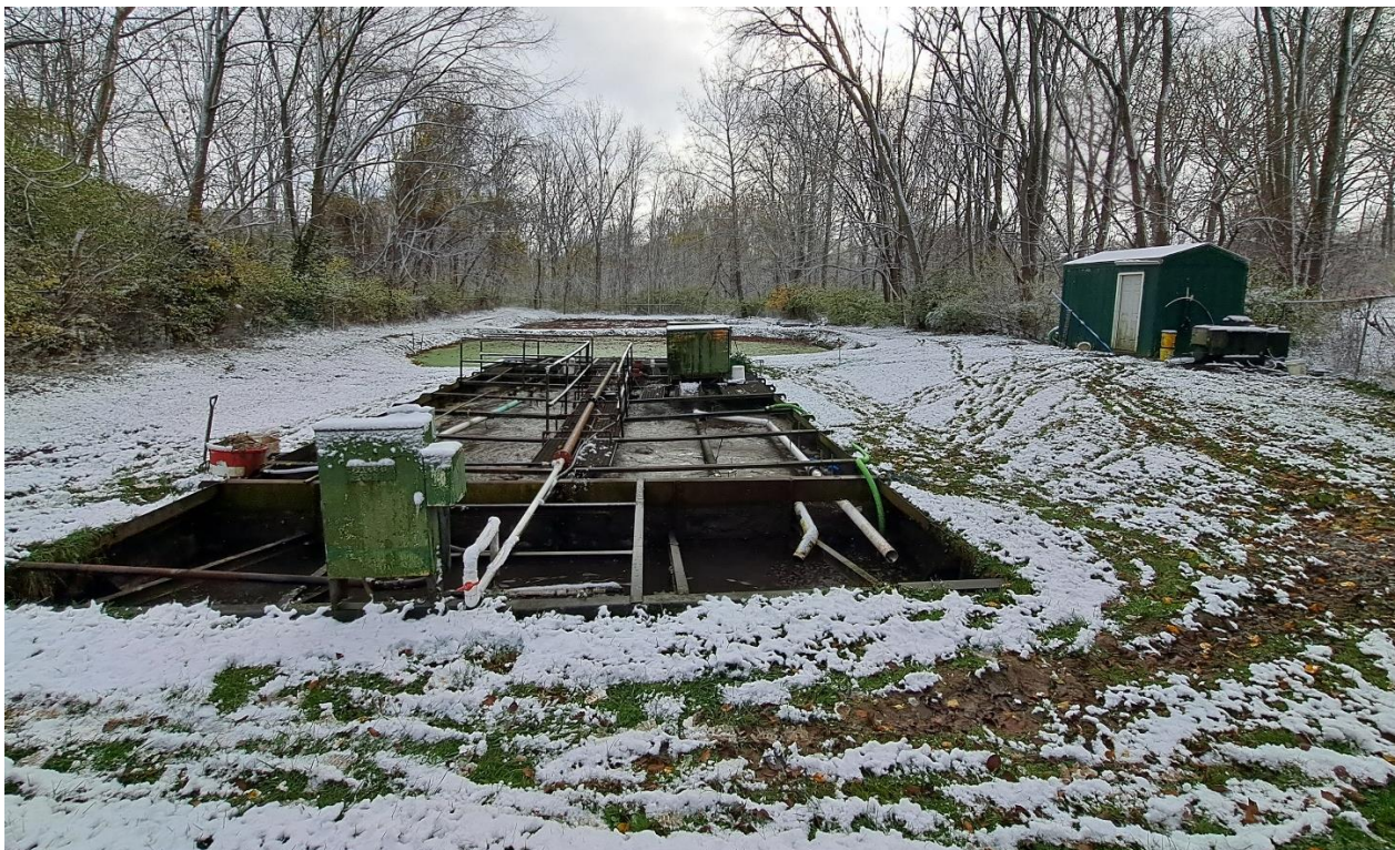
Fig. 2 – 2024 Photo View SE of the 1974, 60,000 gpd steel package plant with polishing ponds beyond. Note replacement air header pipe is a tripping hazard above the center walkway grating.
