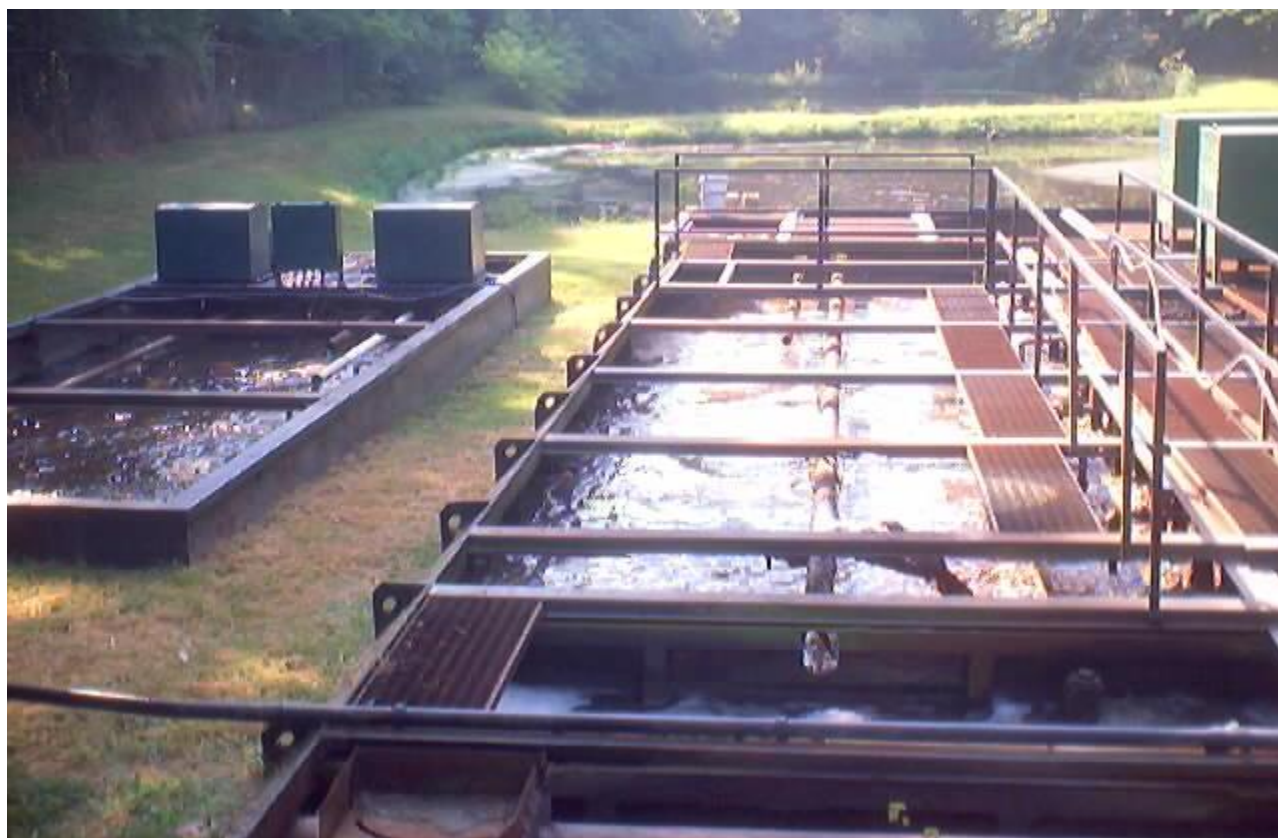
Fig. 3 – 2002 Photo of the 1974 Package Plant tankage and the original Package Plant at left. Note the grated walkway is free of tripping hazards.
