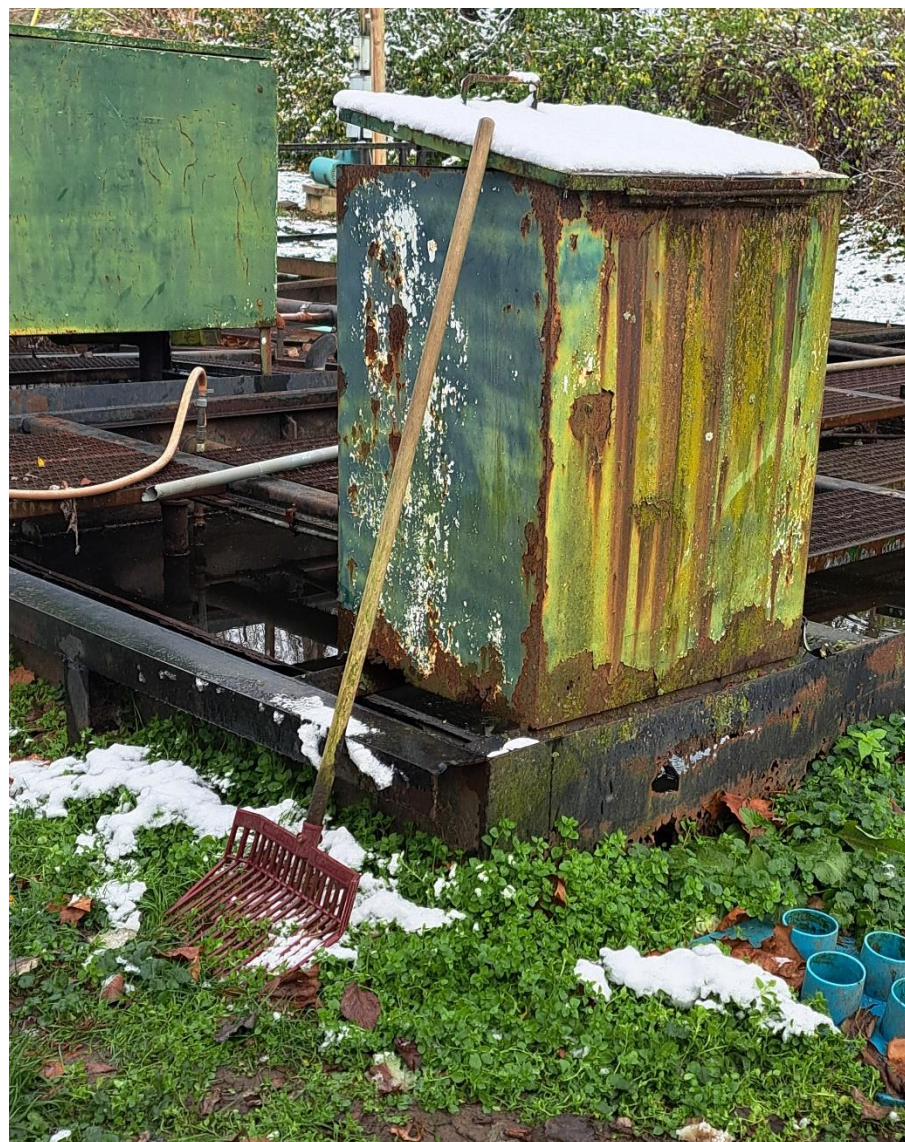
Fig. 19 – 2024 Photo - View of holes thru tank wall at clarifiers
