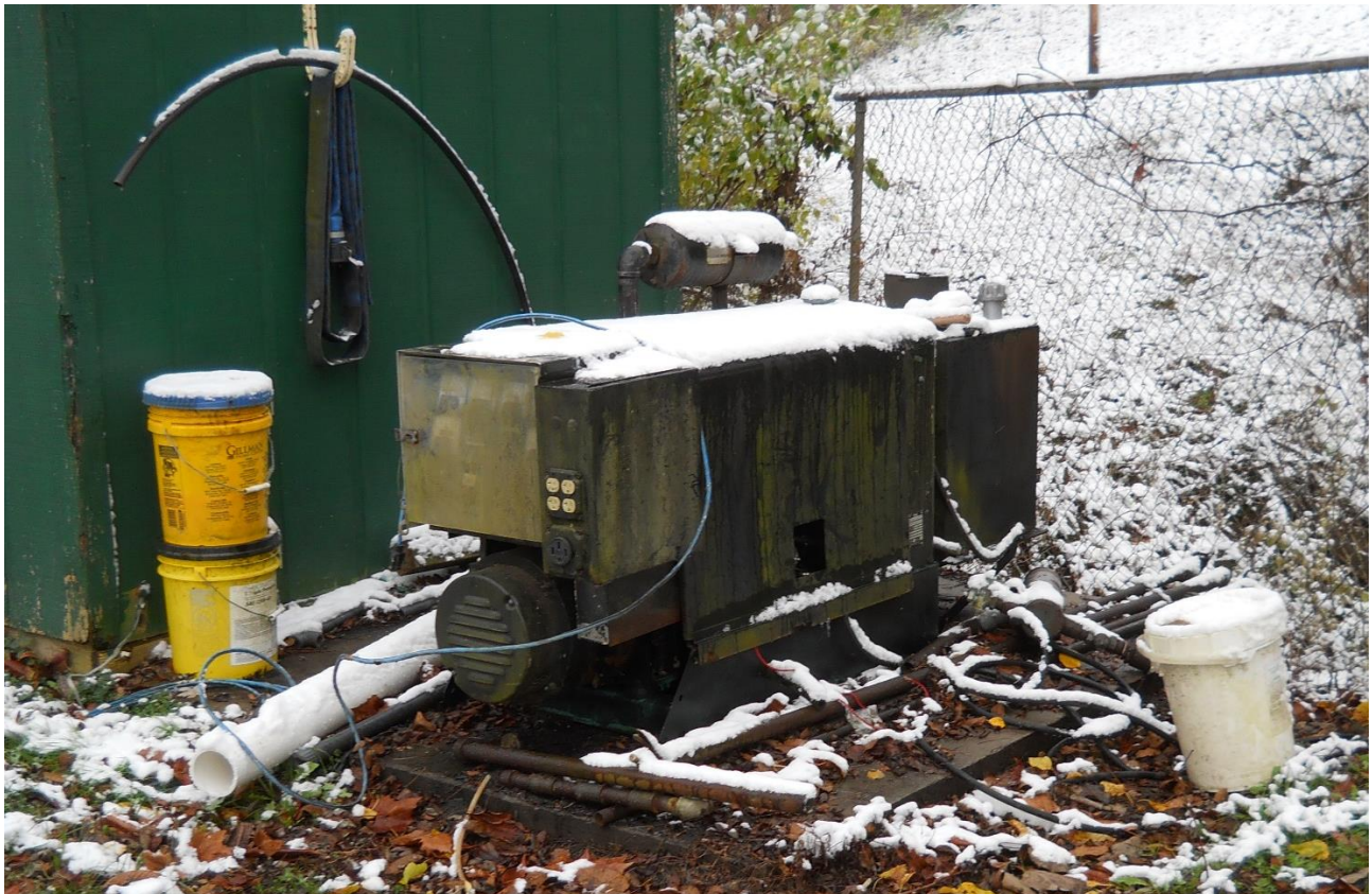
Fig. 16 – 2024 Photo of the emergency generator next to the shed.
