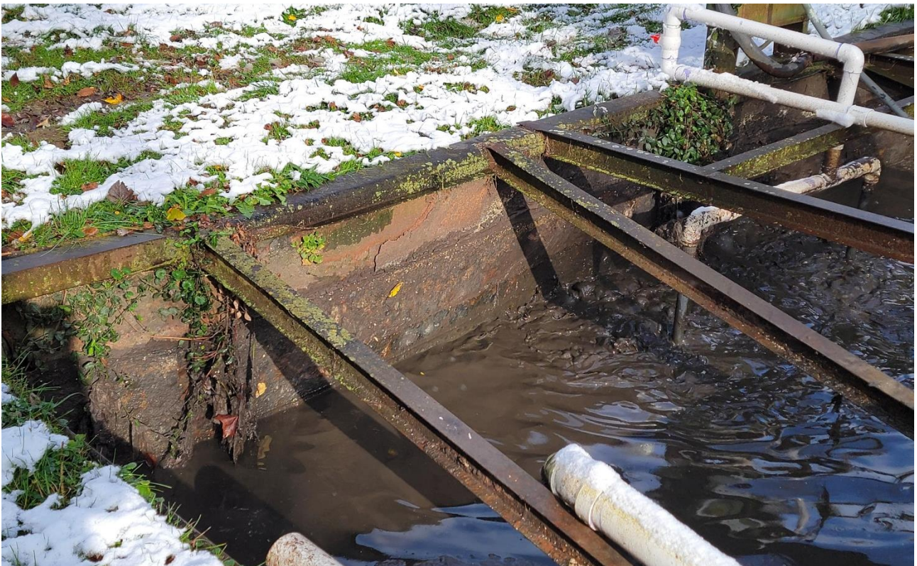
Fig. 8 – 2024 Photo -Close-up view of the bowed NW wall showing loss of paint coating, flaking steel rust, and vegetation. Additional beams (angled) appear added to retain the bowed wall.
