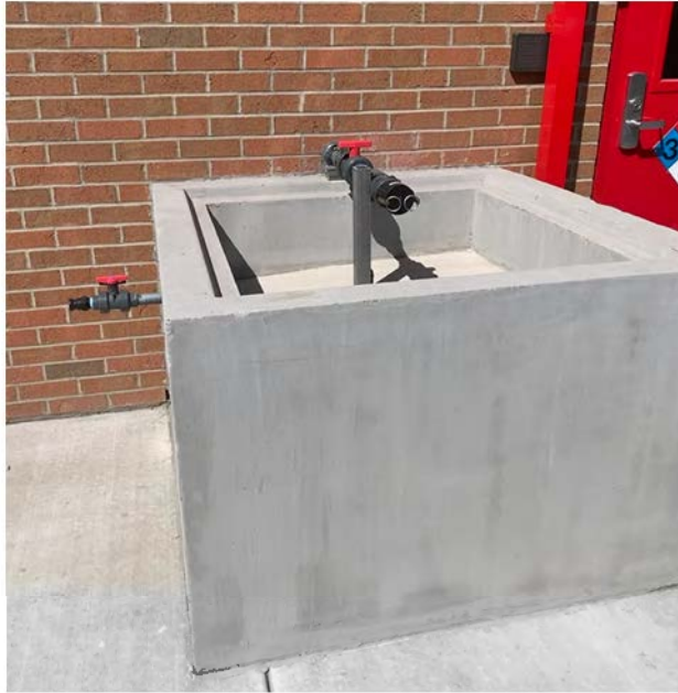
Figure 5-22: Example Chemical Fill Station
