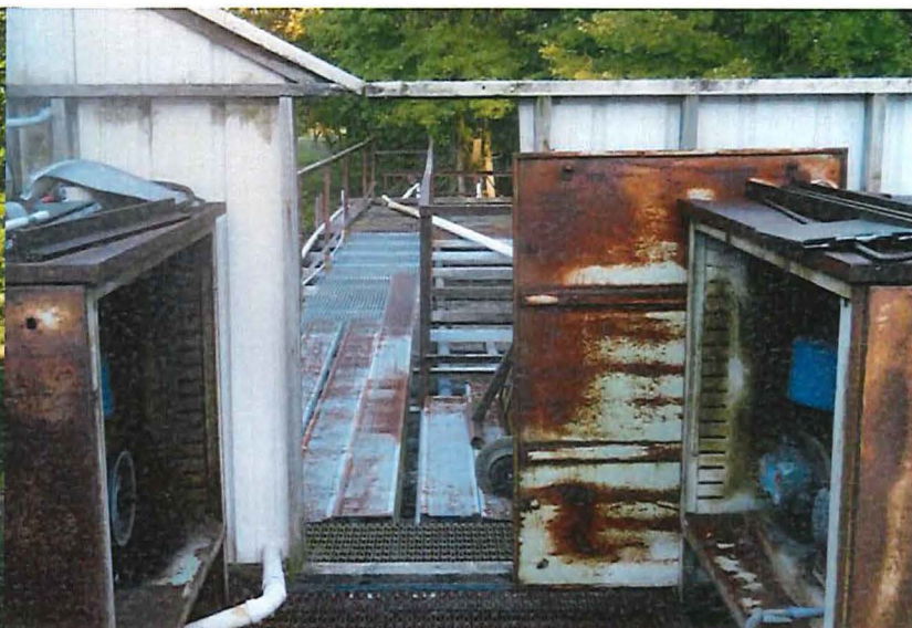
Fig. 8 View west on top of tanks showing blowers (in foreground).
