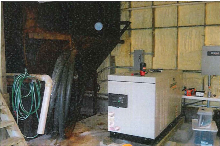
Fig. 11 View of clarifier (left) and new standby power generator.
