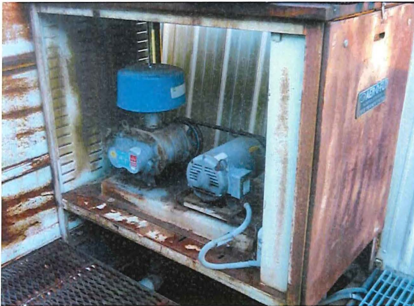
Fig. 15 View of aeration blower (one of two blowers).
