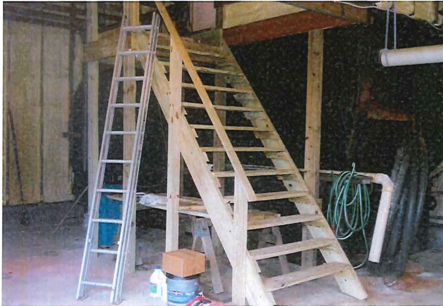
Fig. 9 View of new access stairs inside Control Bldg. (to top of tanks)
