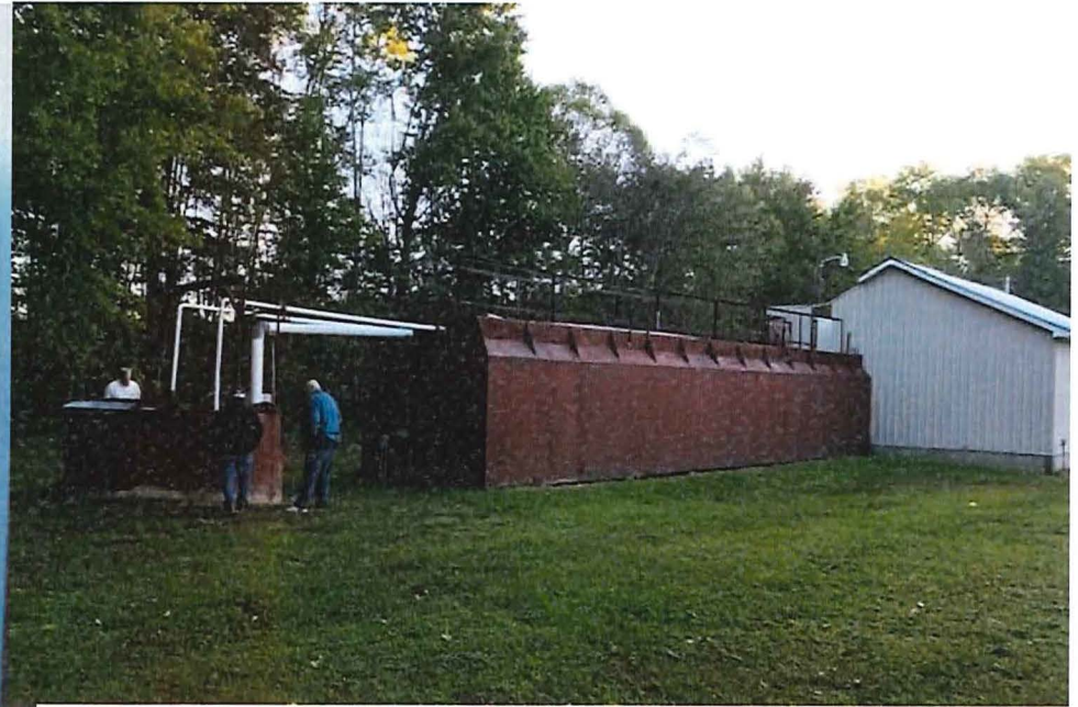
Fig. 4 View of Raw Sewage Pump Station (left), Sludge Digester and Aeration Basin (large brown tank), and Control Building (right).
