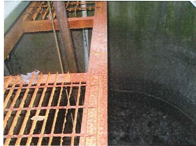
Fig. 2 Inside of Raw Sewage Pump Station showing rusted steel.
