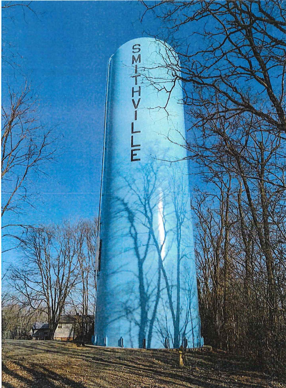
Smithville tank – 300,000 gallons
