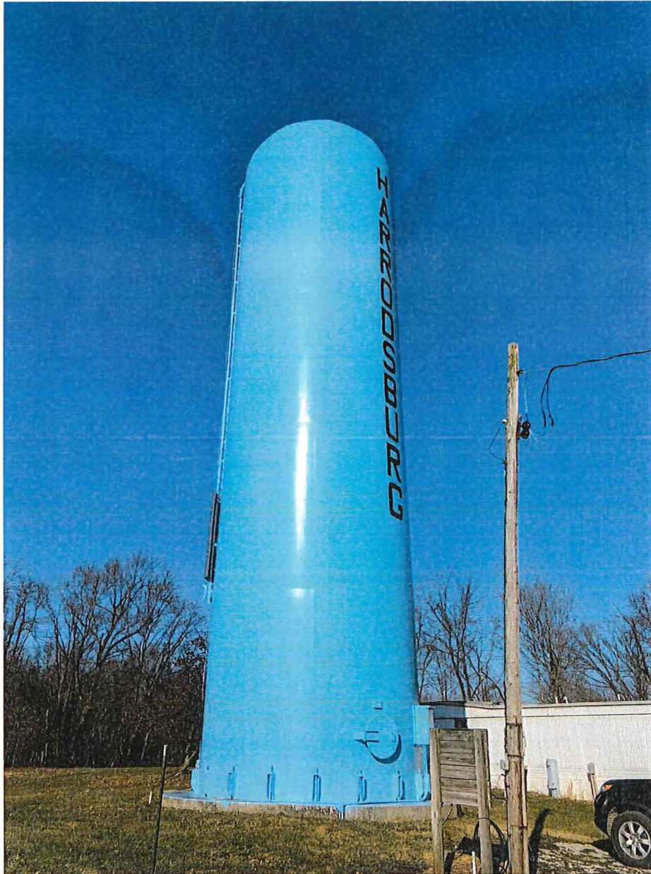
Harrodsburg tank – 100,000 gallons
