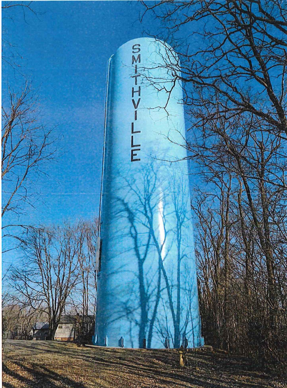
Smithville tank – 300,000 gallons
