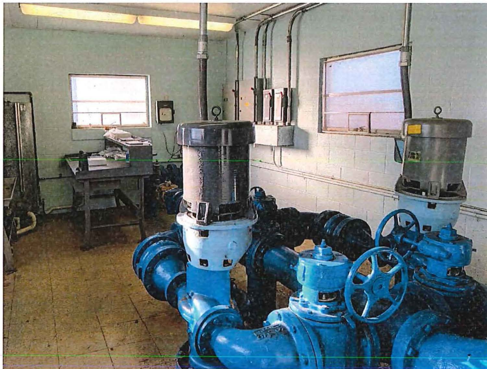
North (office) booster – interior
