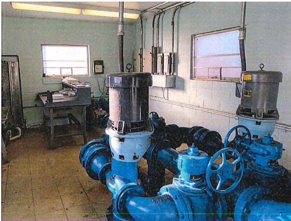
North (office) booster – interior
