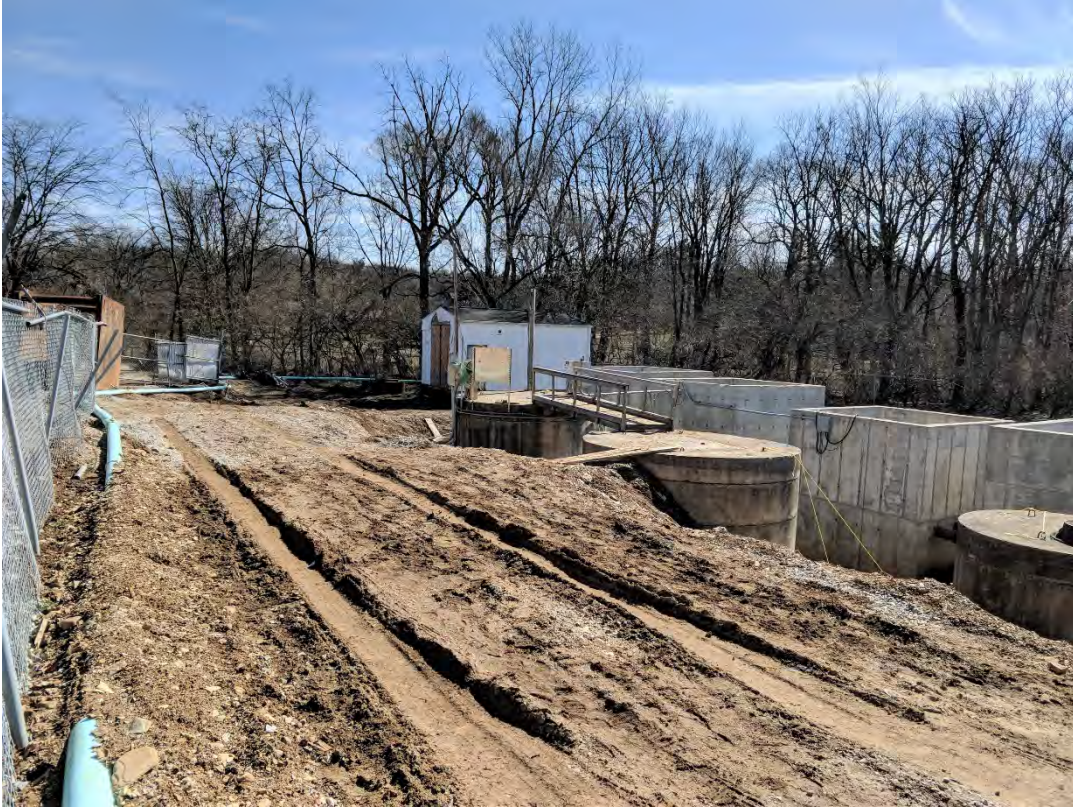
03/05/2020 Rough site grading, final grading, final pavement, sidewalks, fencing (Status: Not Complete)
