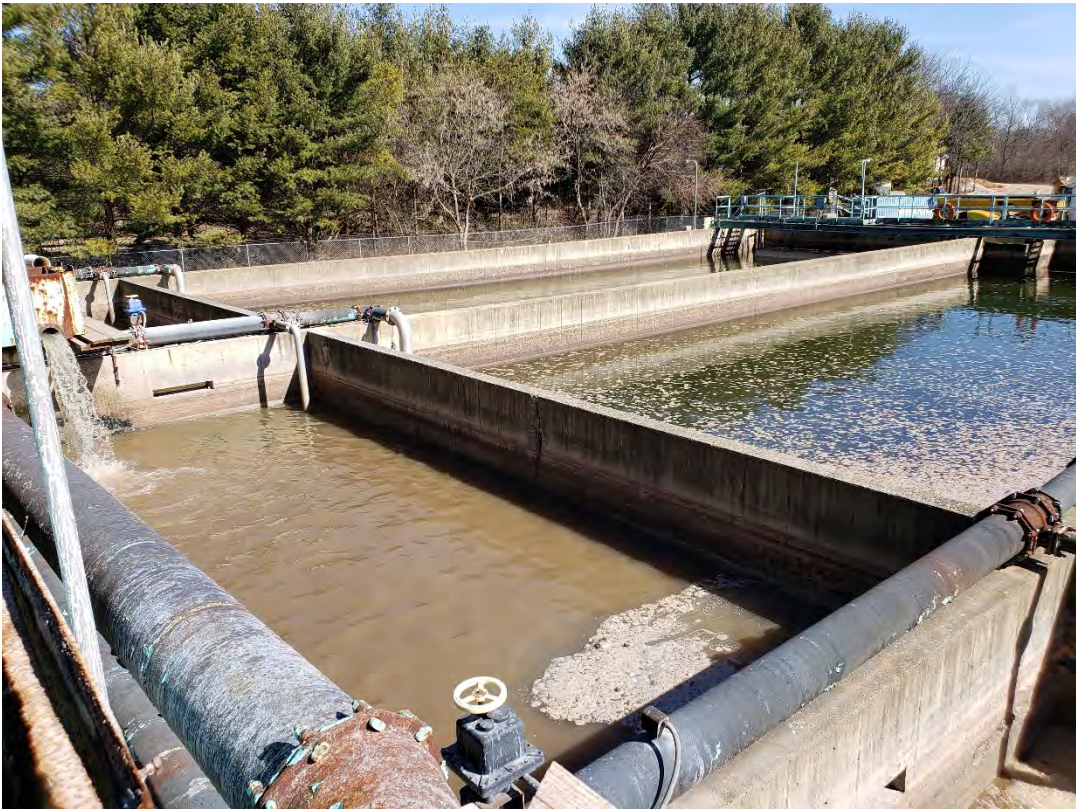
03/05/2020: CSBR tanks not rehabilitated
