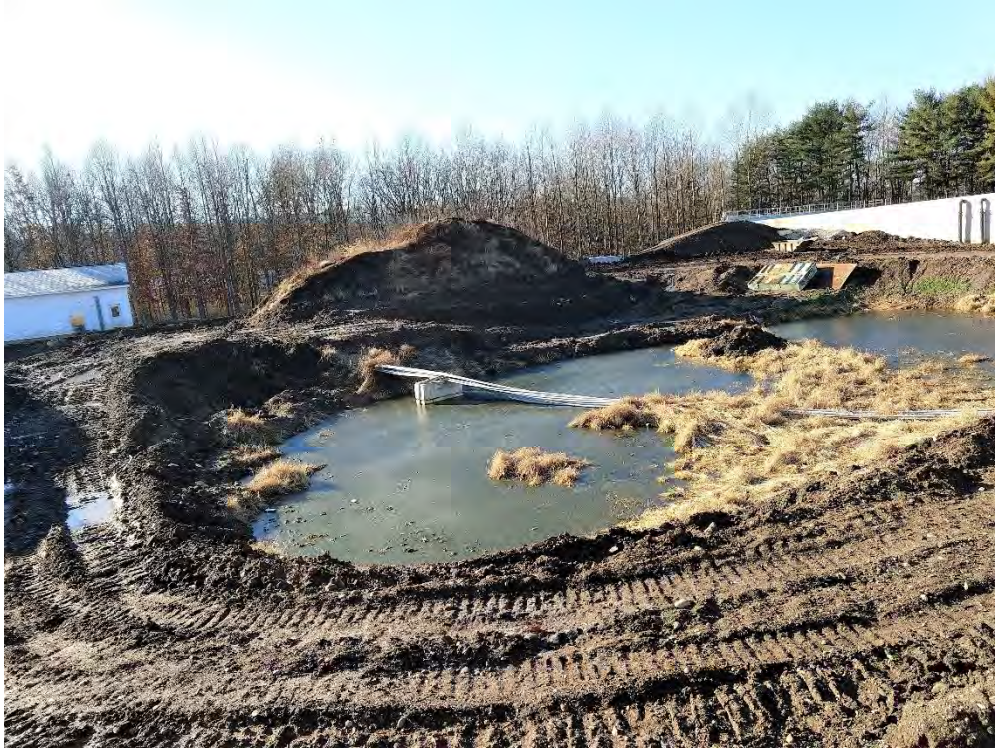
12/04/2019: Sludge pond (Status: Not removed)
