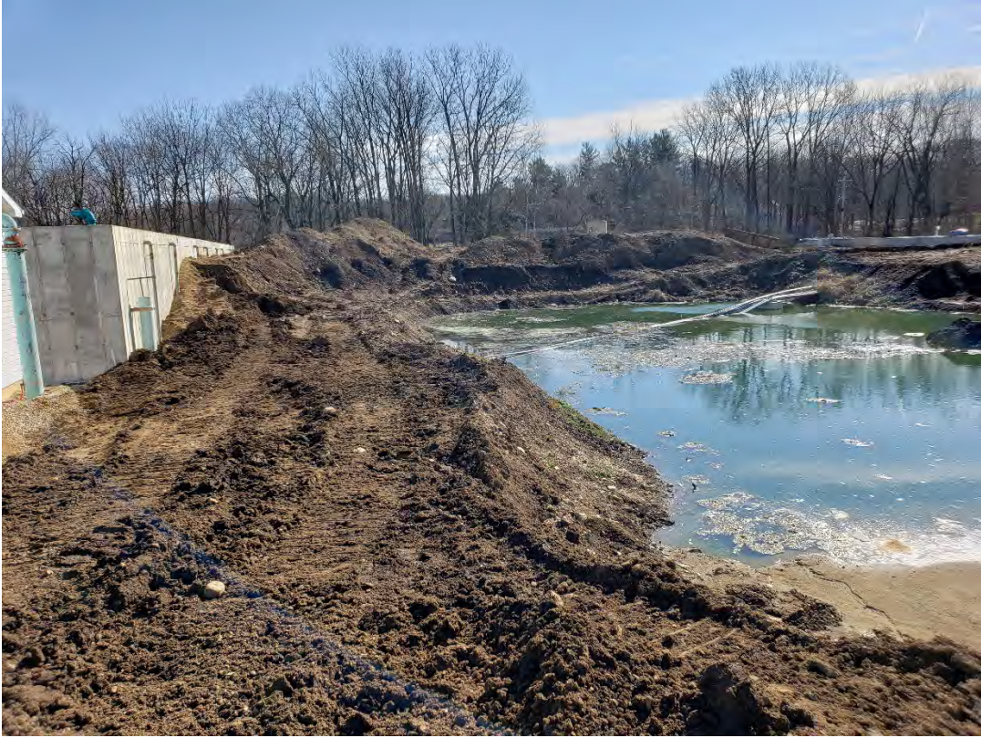
03/05/2020: Sludge pond not closed
