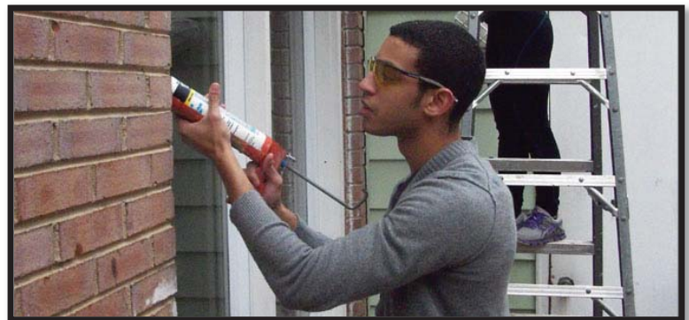
Weatherization of homes is easy and effective way to reduce energy use Source: Habitat for Humanity, Prince William County, VA
