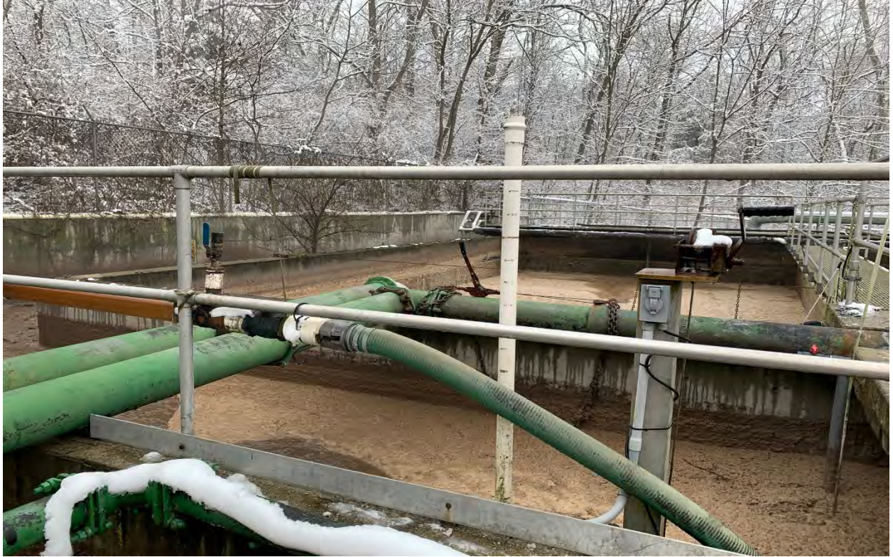
Sequence Batch Reactor Tanks Photo 1
