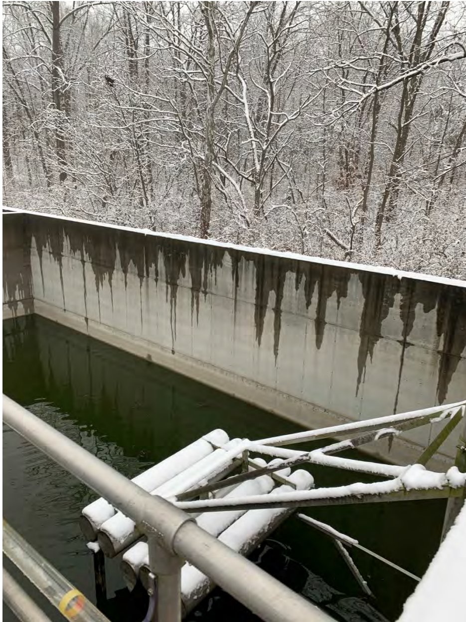
Sequence Batch Reactor Tanks Photo 4
