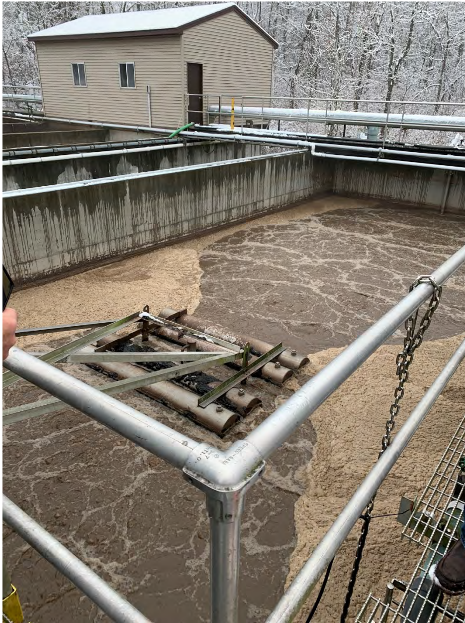
Sequence Batch Reactor Tanks Photo 3
