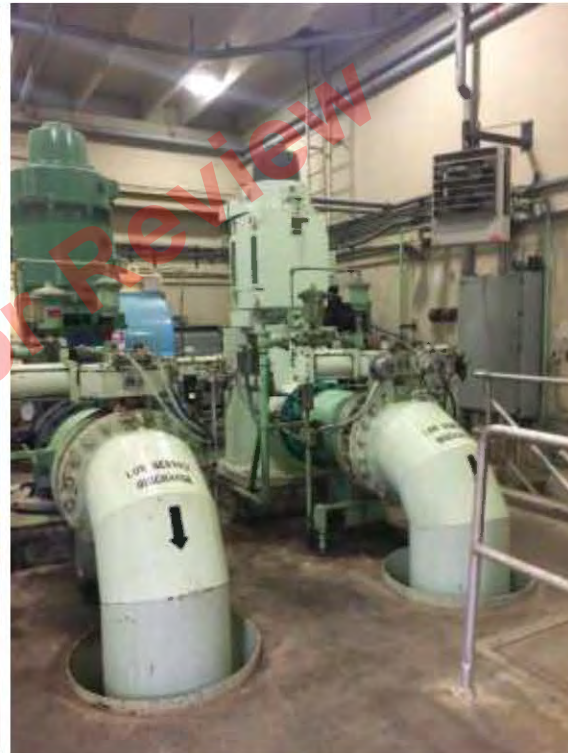
FIGURE 2-2 Low Service Pumps
