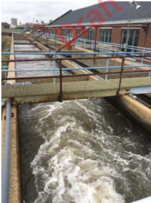
FIGURE 2-3 Raw Water Flume
