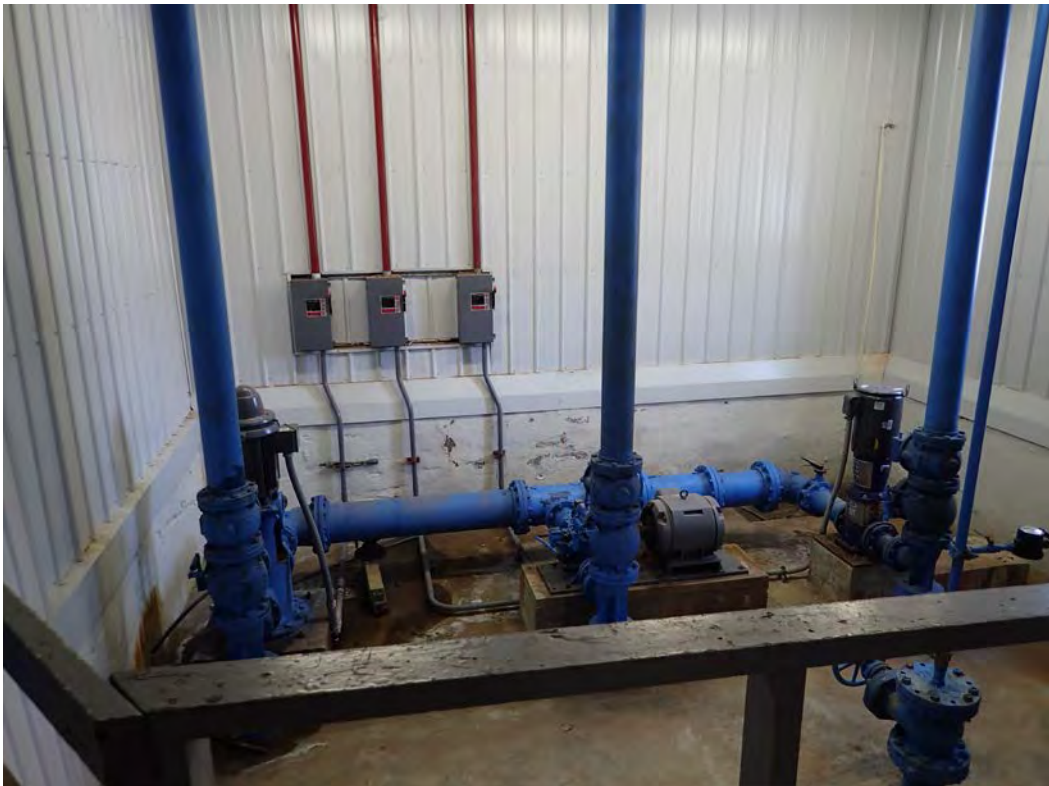
Interior of plant, high service pumps feeding 250,000 gallon elevated tank
