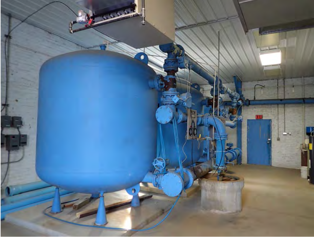
Interior of plant, filter room
