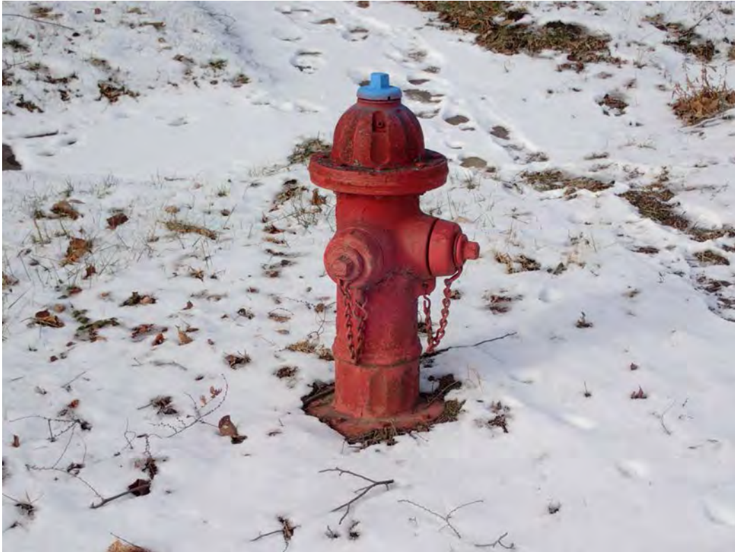
Typical Mueller hydrant with blue marking indicating flushing
