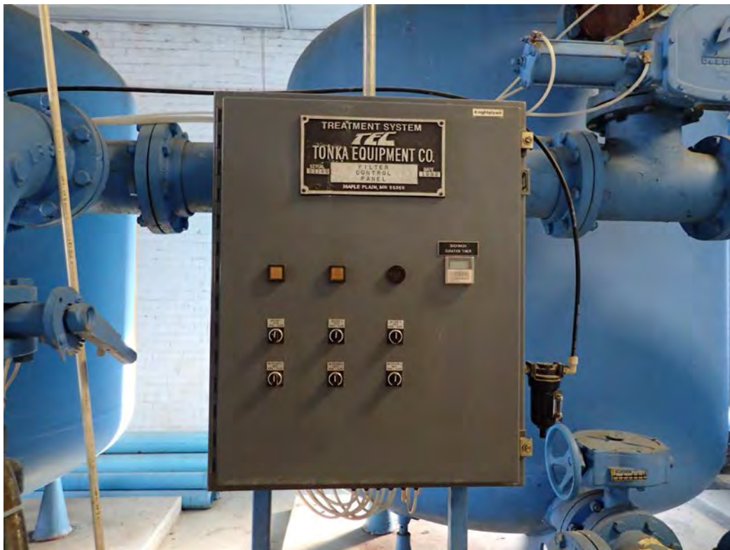
Filter control panel
