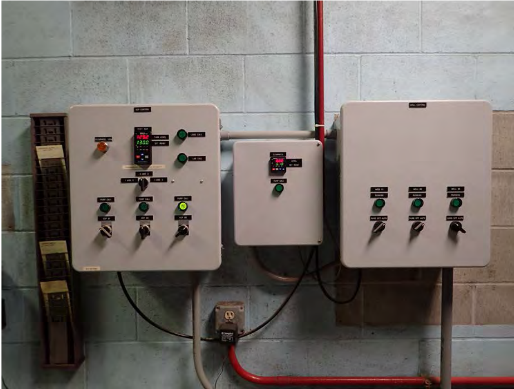
High service pump (L) and well (R) controls, driven by elevated tank and clearwell levels
