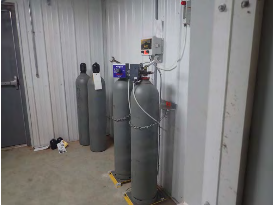
Interior of plant, chlorine storage room
