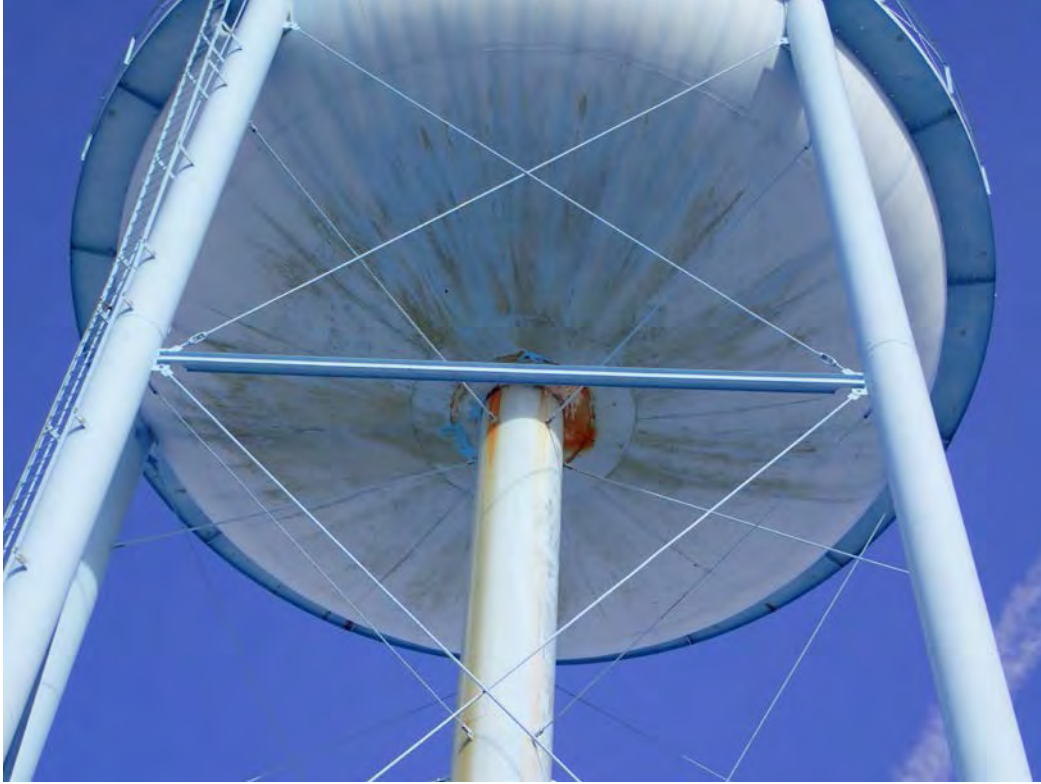
Close-up of tank bottom showing 2016 repairs due to leakage
