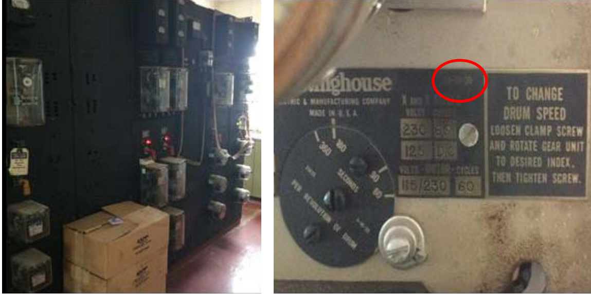
Figure 1. This photo shows a relay system from 1939 that is still in service.
