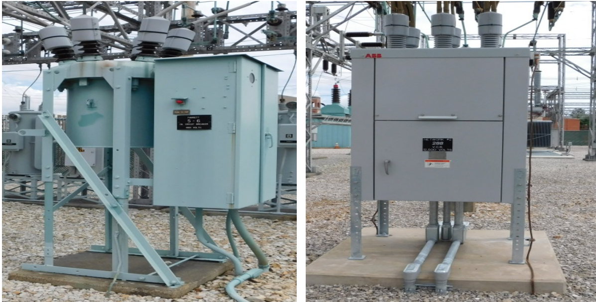
Figure 1. Example of an aged 12kV oil breaker (left) and a new 12kV vacuum breaker (right)
