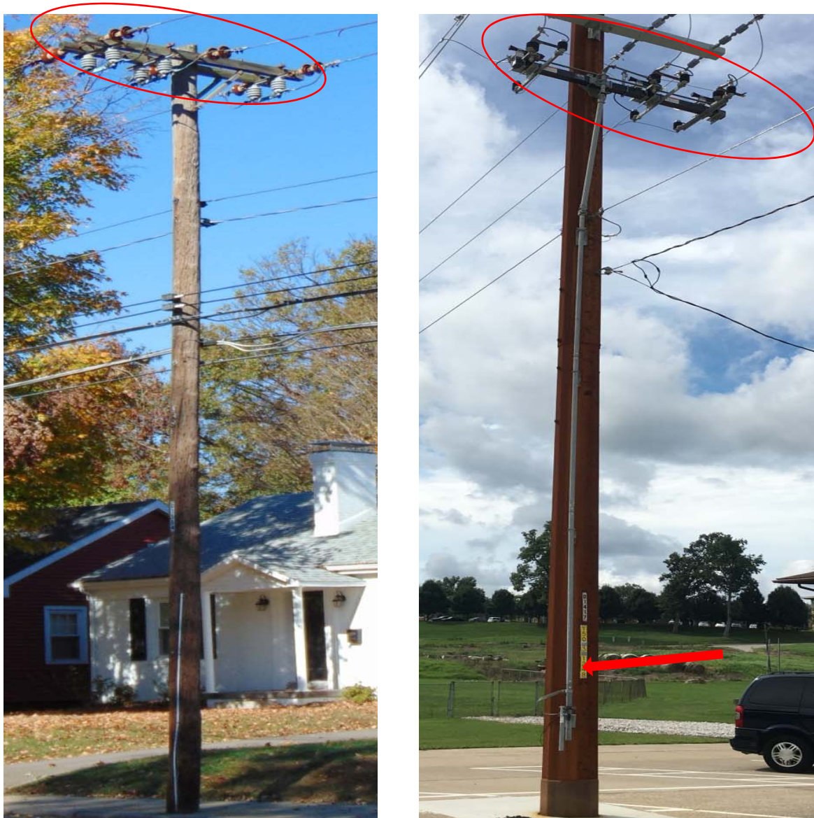
Figure 1. Example of three single underslung switches (left) and example of GOAB switch (right)
