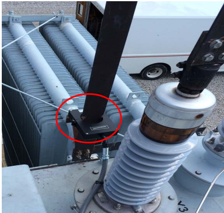
Figure 2. Current Transformer (CT) installed to measure transformer neutral to ground.
