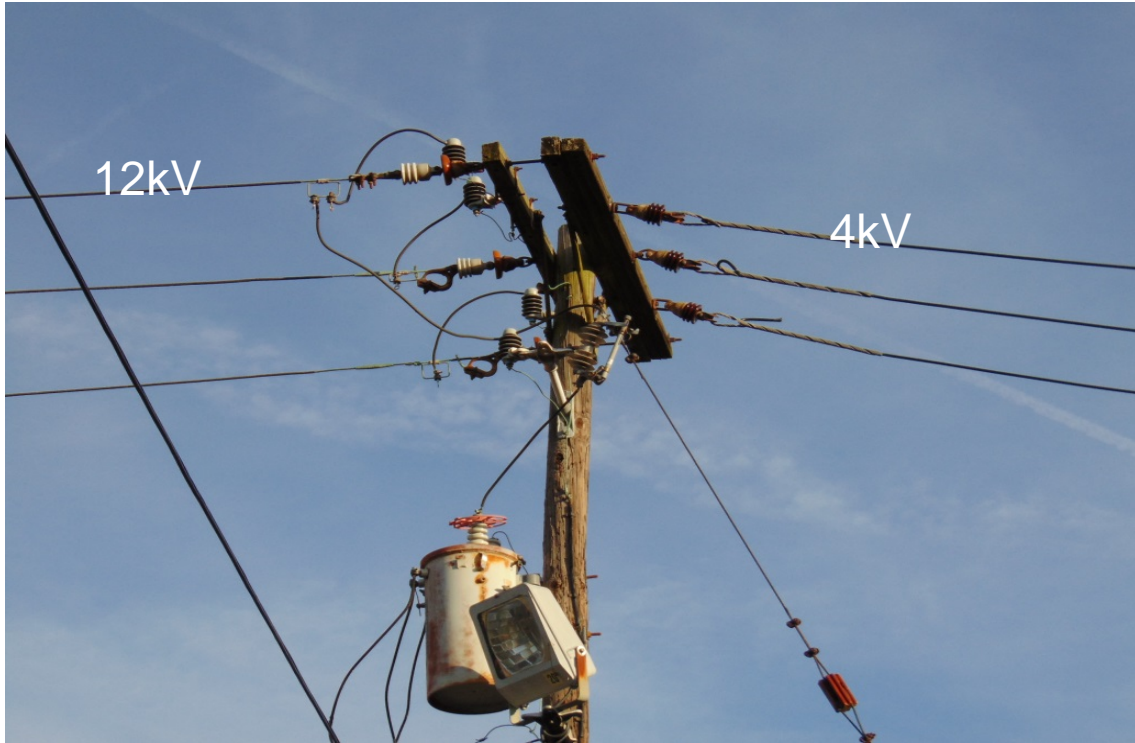
Figure 1. Pole location where a 12kV feeder and 4kV feeder meet. After converting the 4kV system to 12kV, this location and others will be outfitted with switches enhancing operational flexibility in support of increased reliability.
