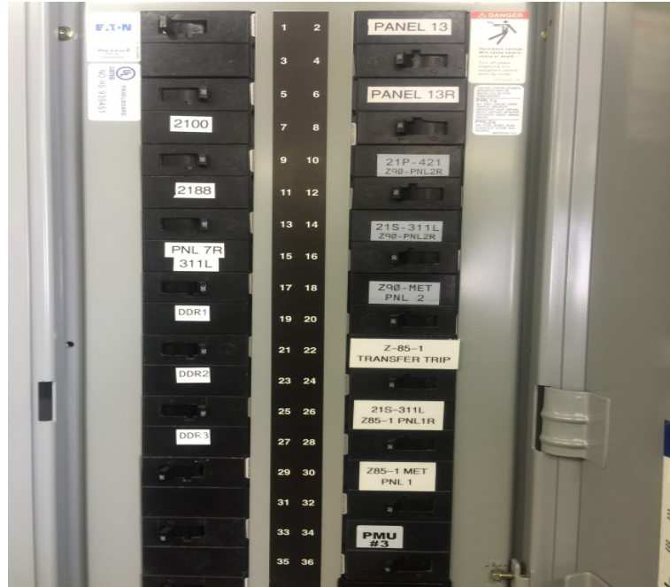
Figure 1. Current battery backup equipment and panel
