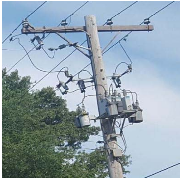
Figure 1. Example of switched capacitor bank with oil switches
