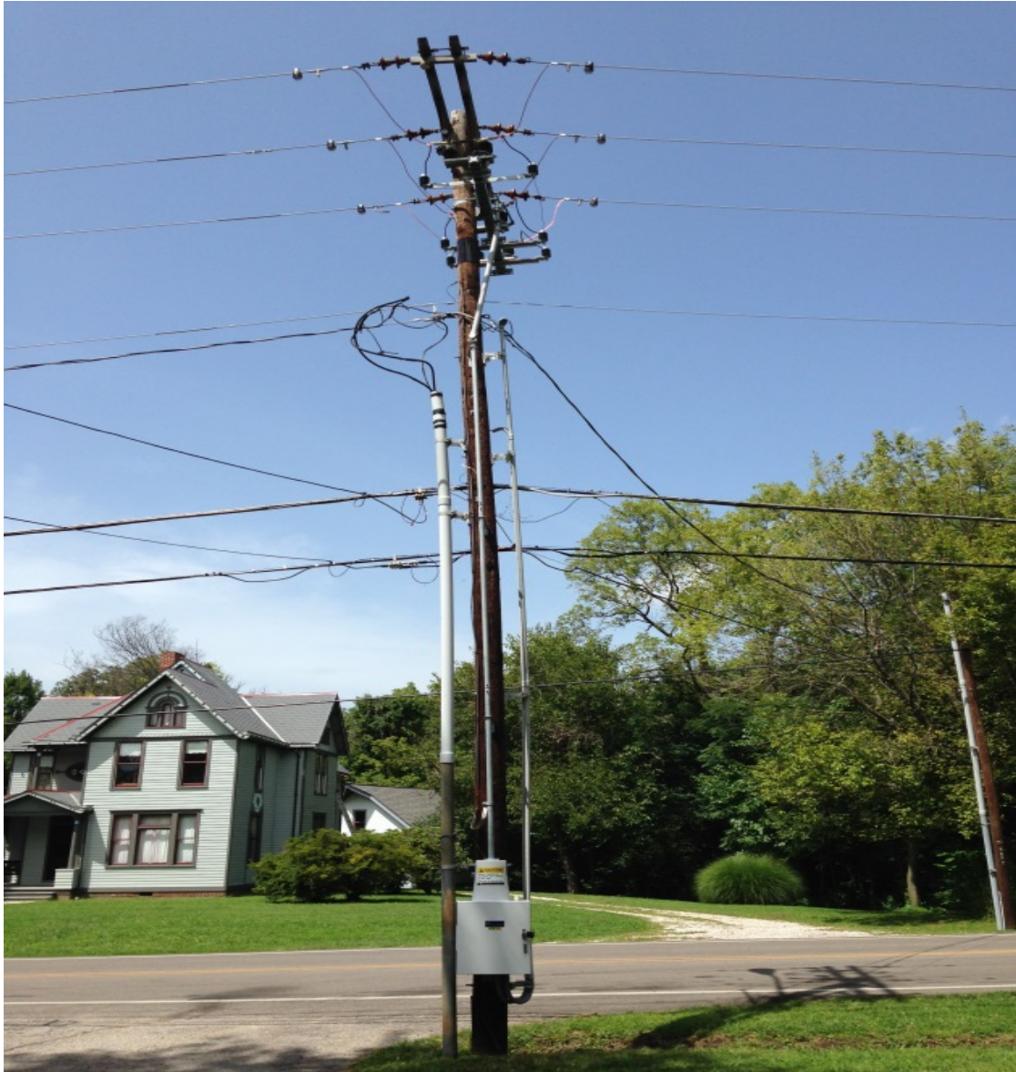
Figure 2. Example of entire DA switch installation showing GOAB switch at top of pole and motor operator/controls cabinet with connecting linkage to switch
