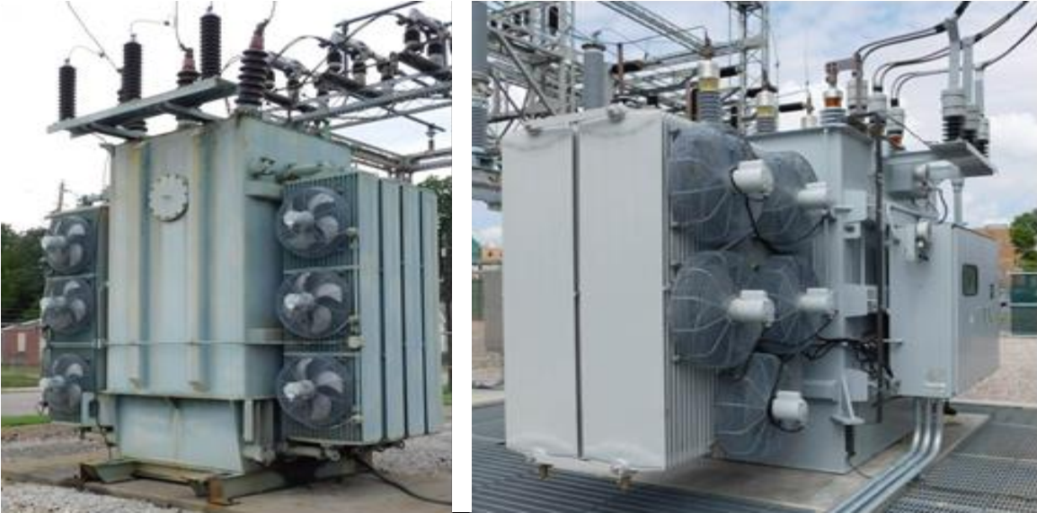
Figure 1. Example of an older substation transformer (left) and an example of a new substation transformer (right)
