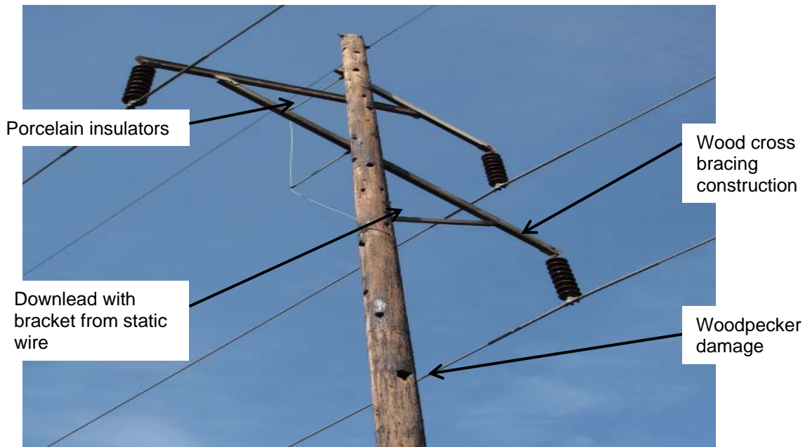
Figure 2. Existing transmission structure with woodpecker damage and older style construction
