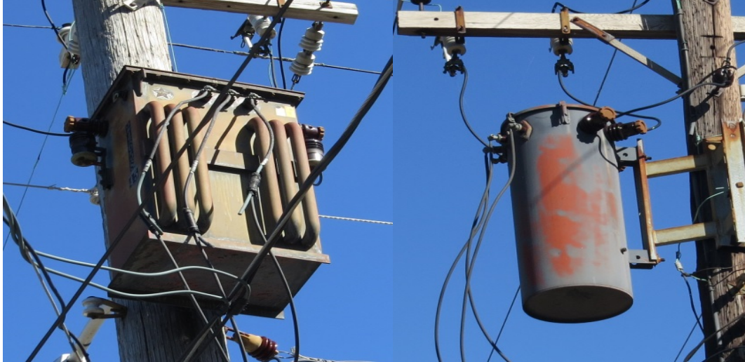
Figure 1. Examples of transformers manufactured before PCB ban
