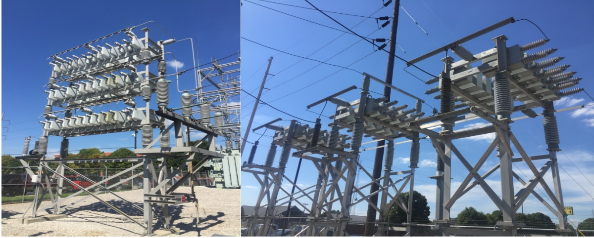
Figure 1. An added benefit of the new internally fused capacitor banks (right) versus the older externally fused capacitor banks (left) are the reduced risk of outages due to birds nesting and other varmints getting into the openings.
