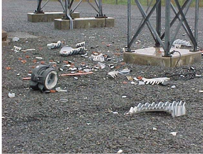
Figure 1. Example of a failed porcelain housed arrester
