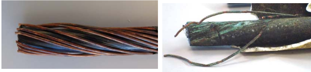
Figure 1. Pictures above show an example of an UG cable with a new bare concentric neutral cable (left) and an example of corroded concentric neutral cable (right). Notice that the corroded concentric neutral cable is missing most of its copper strands.
