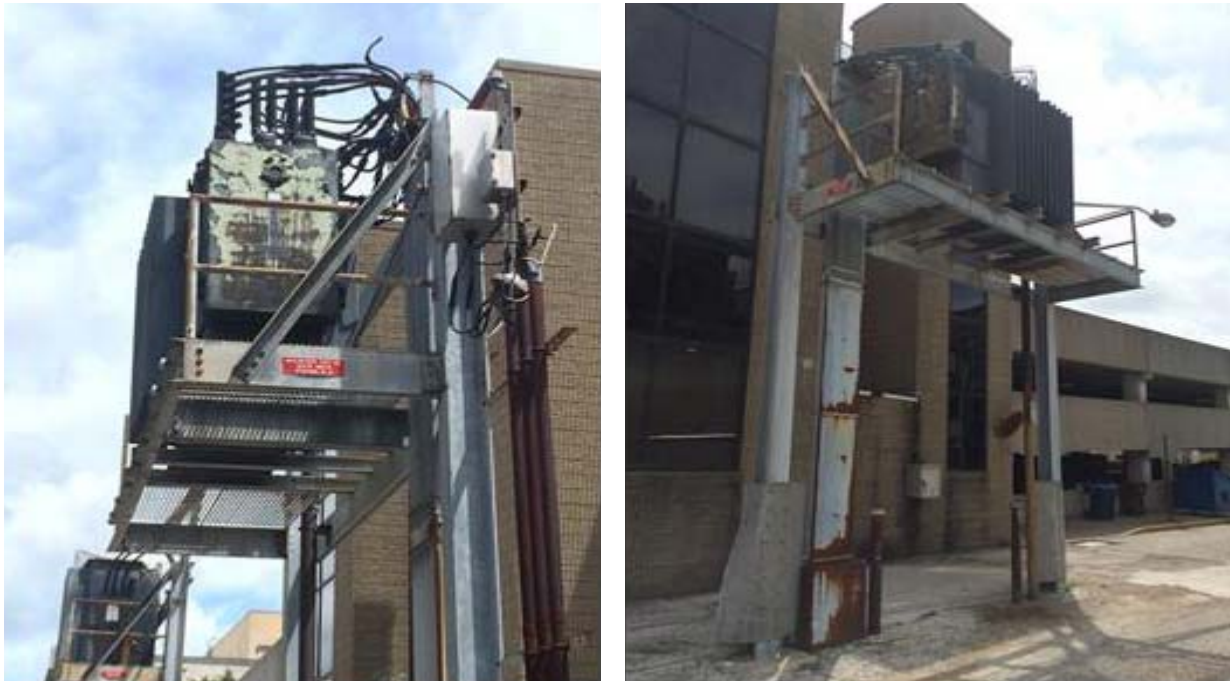
Figure 1. Although most network equipment is installed below grade, this example shows aged network protector and transformer installed on an elevated platform.
