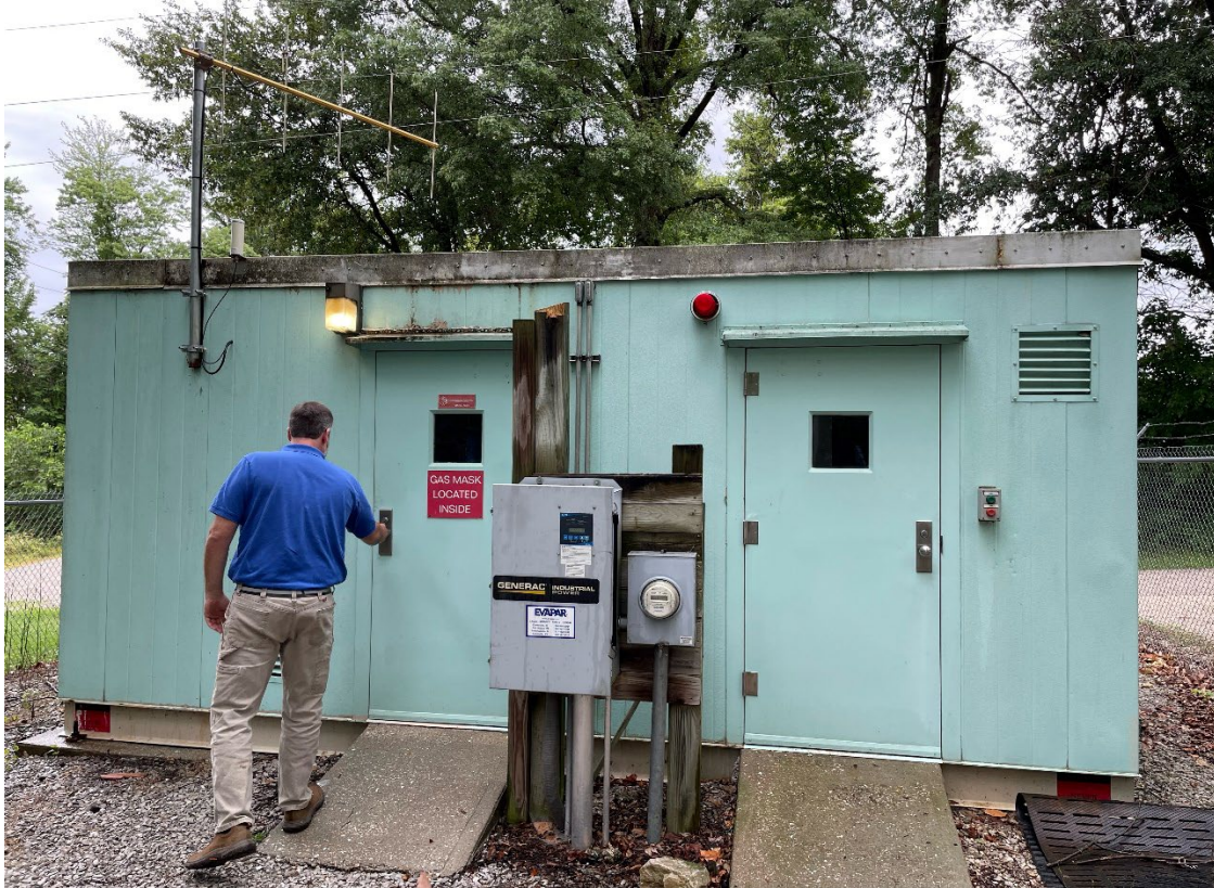
Bogard Bottoms Wellfield Water Treatment Plant Exterior
