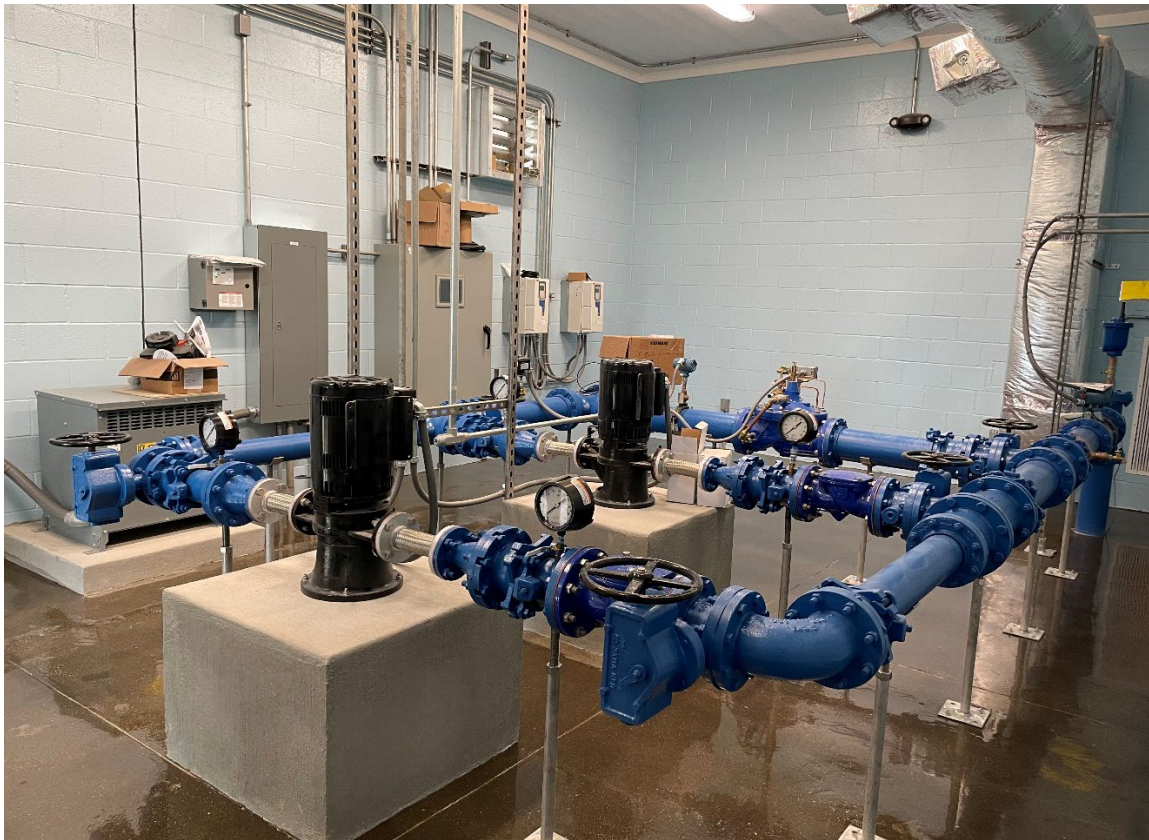
New Booster Station #2 Interior
