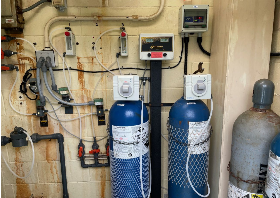
White River Wellfield Water Treatment Plant Interior #2
