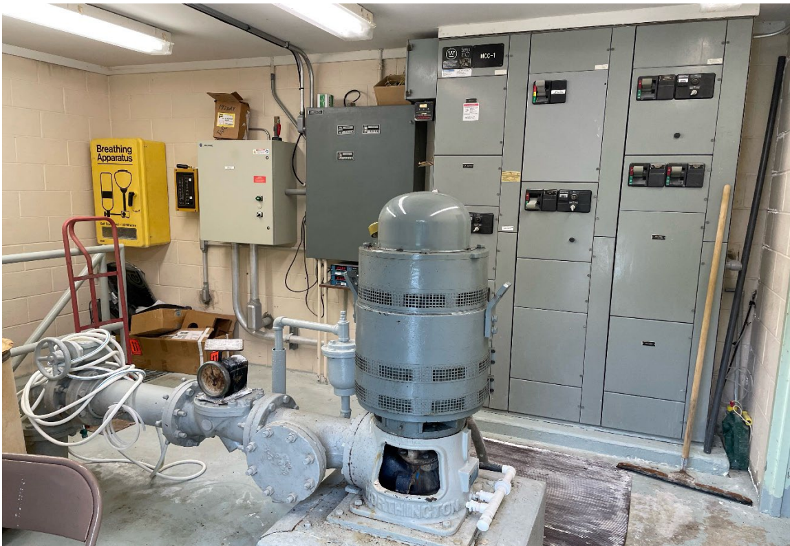
White River Wellfield Water Treatment Plant Interior #1
