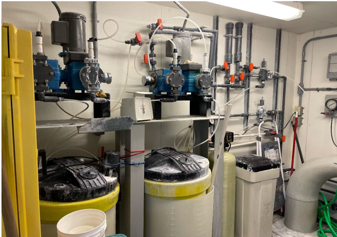
Bogard Bottoms Wellfield Water Treatment Plant Interior
