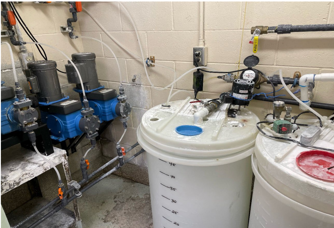
White River Wellfield Water Treatment Plant Interior #3
