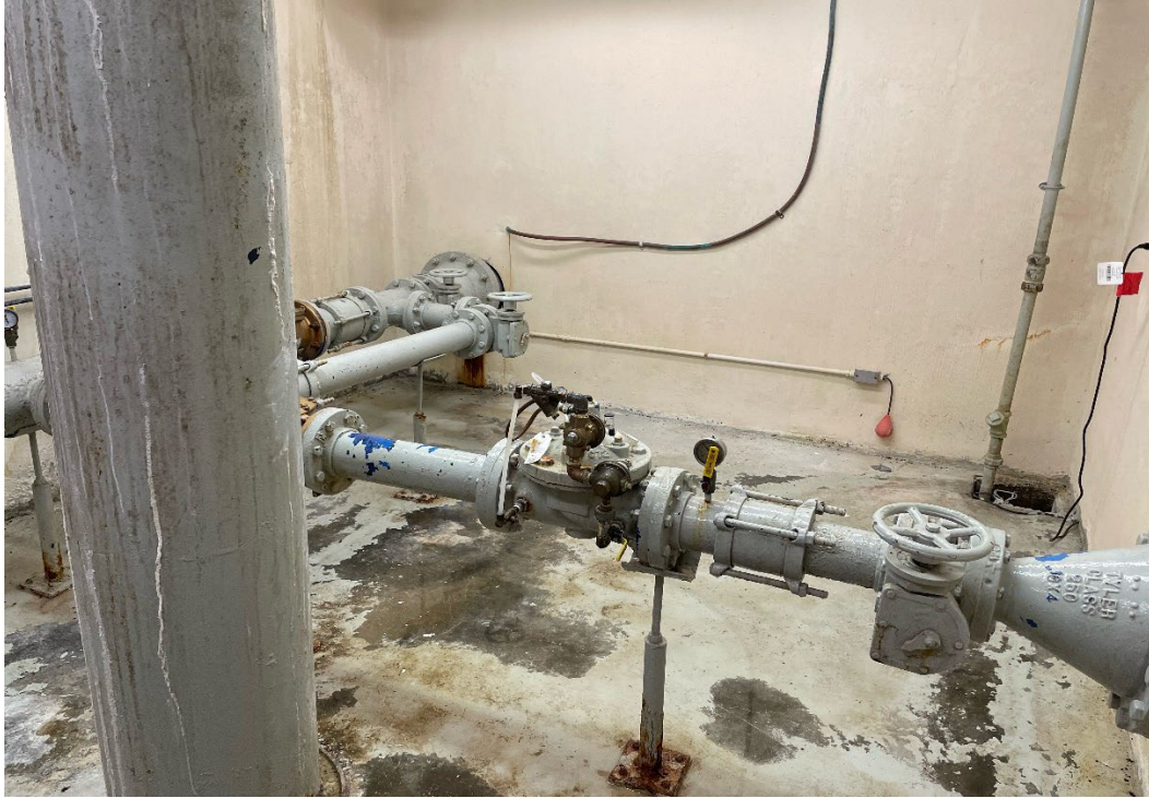
White River Wellfield Water Treatment Plant Interior #4
