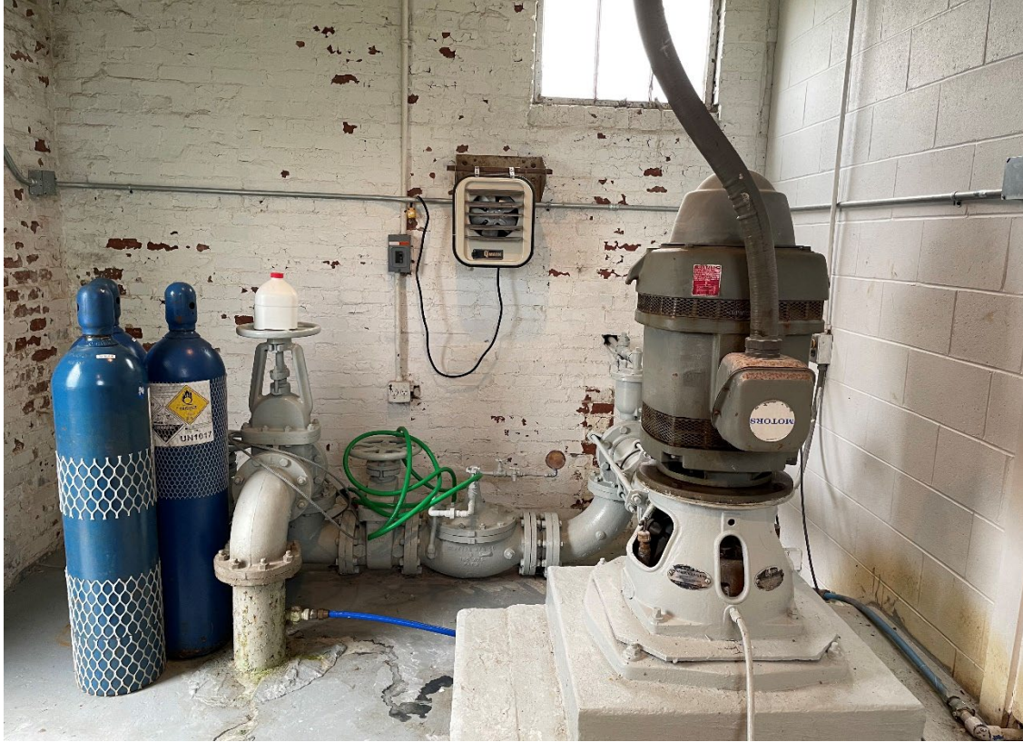
Bloomfield Wellfield Water Treatment Plant Interior #2
