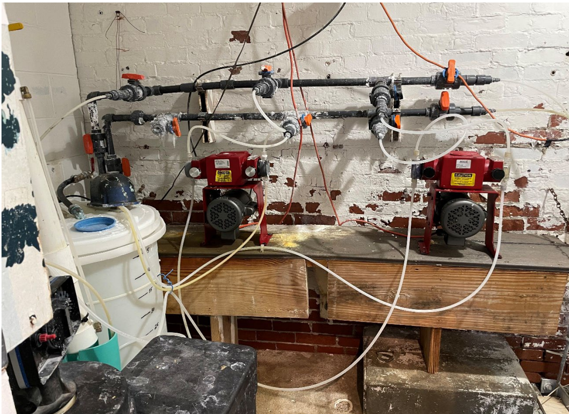
Bloomfield Wellfield Water Treatment Plant Interior #1
