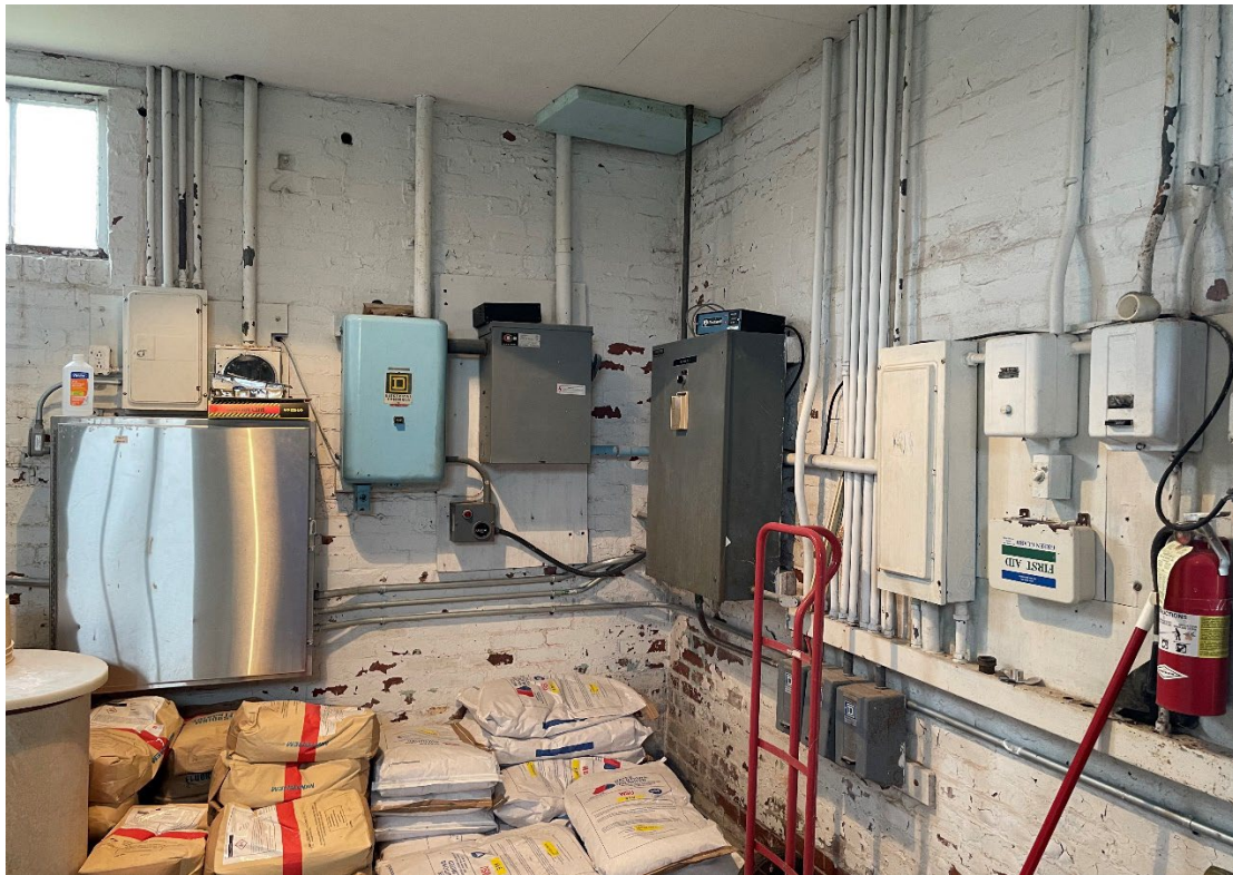
Bloomfield Wellfield Water Treatment Plant Interior #3
