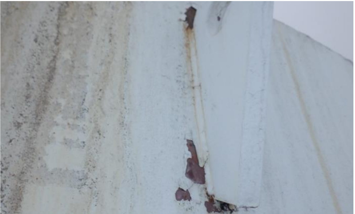
14. Corrosion on shell near lug at top of shell for bottom tank section.
