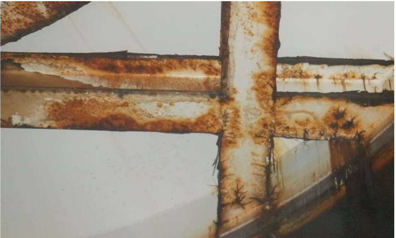
58. Corrosion on middle tank section interior roof support structure.
