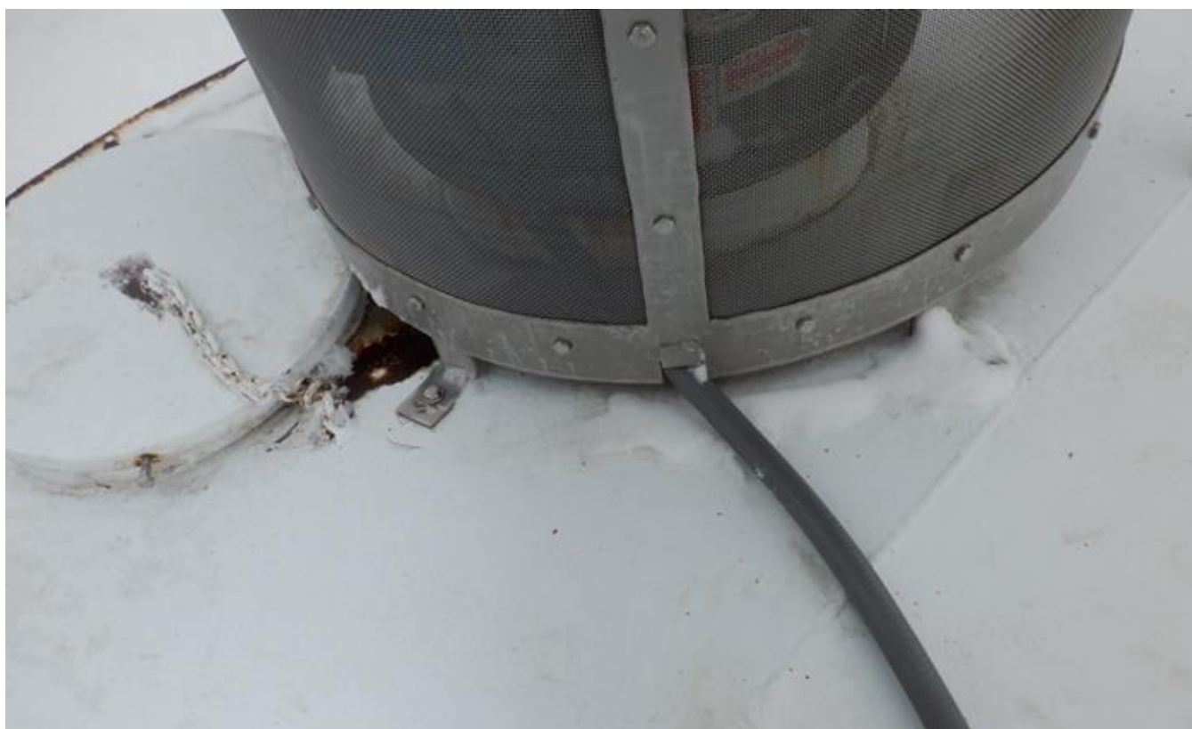
48. Conduit extending to blower on top tank section roof.
