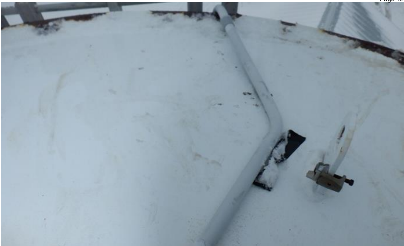
47. Conduit and lug on top tank section roof.
