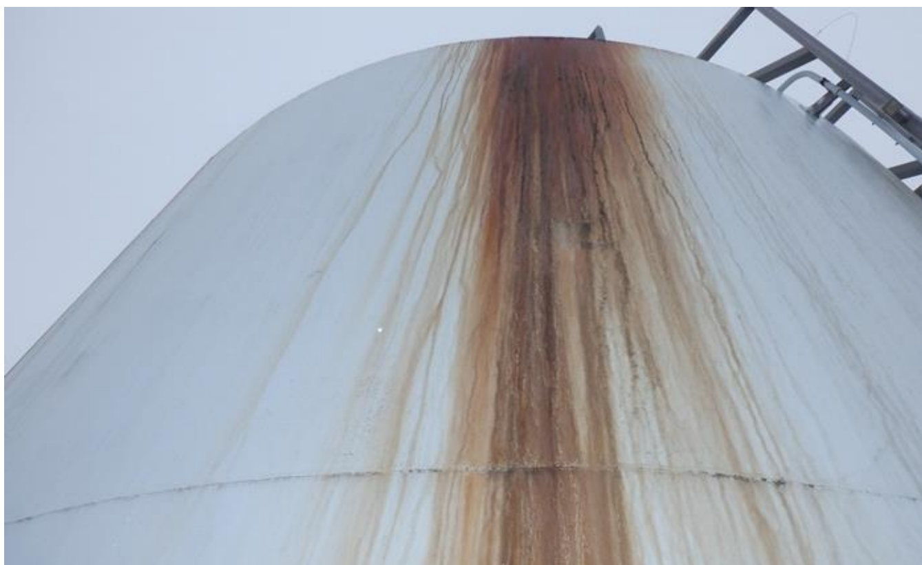
26. Rust staining on middle tank section.
