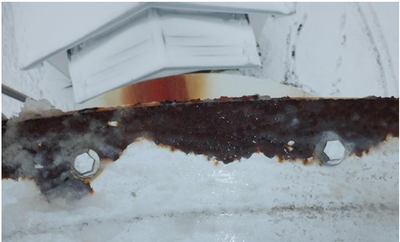
42. Coating failure and corrosion along roof perimeter of top tank section.
