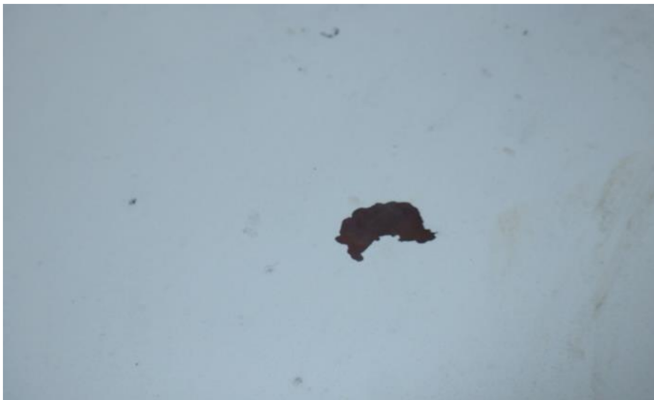
46. Coating failure on top tank section roof.
