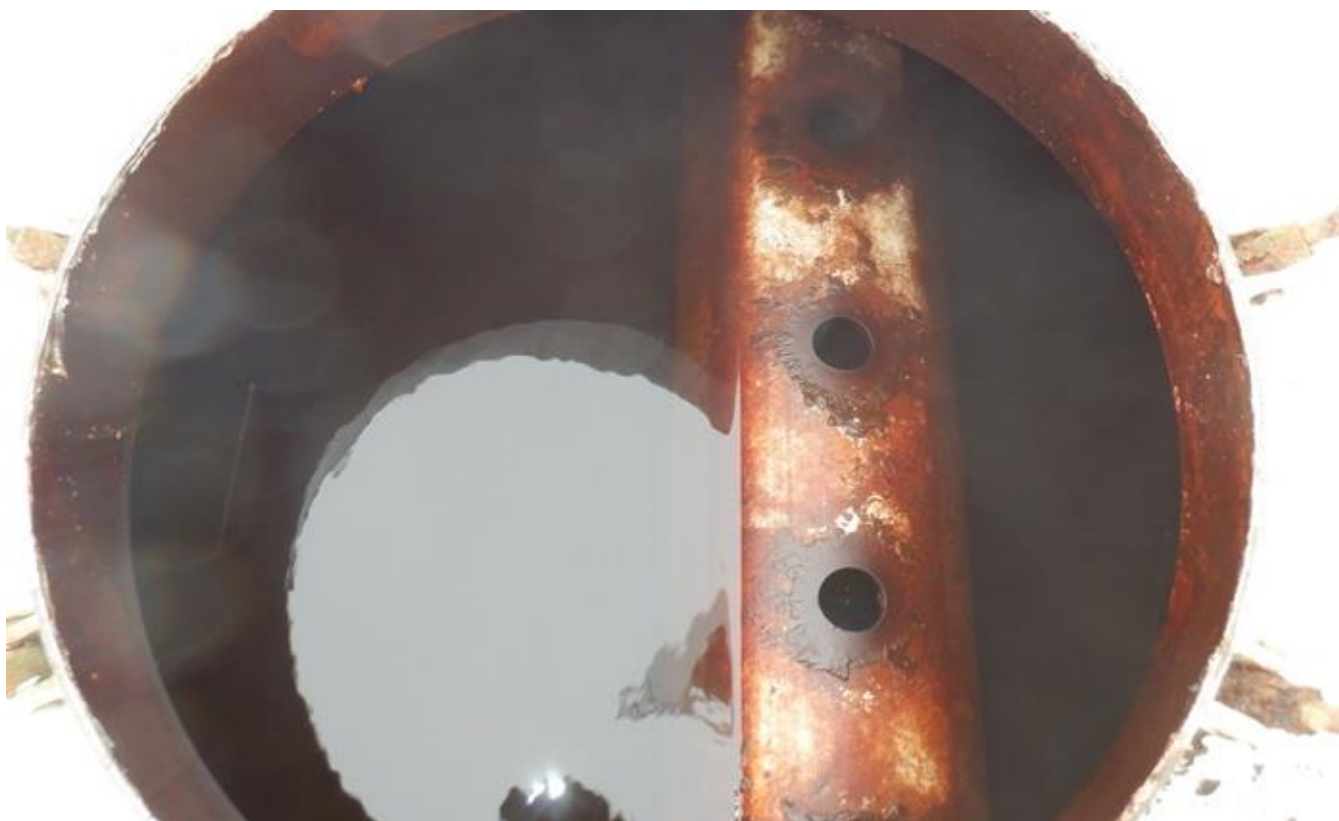
16. Corrosion on interior of bottom tank section roof manhole
