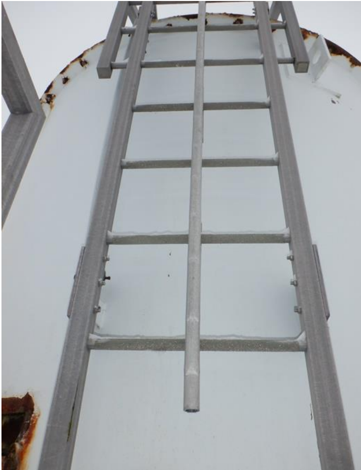
39. Top tank section ladder and safe-climbing device.
