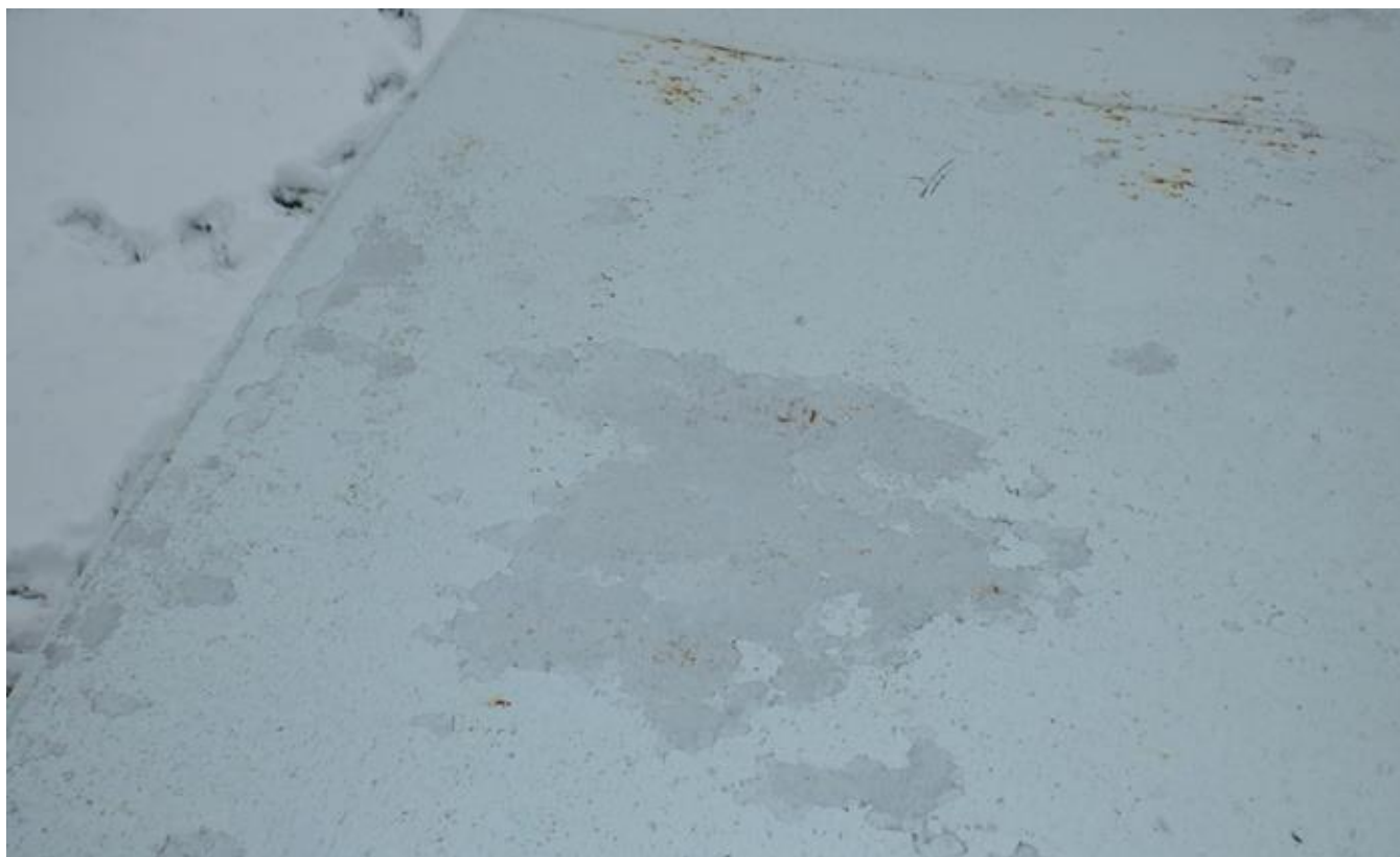
22. Coating failure on bottom tank section roof.
