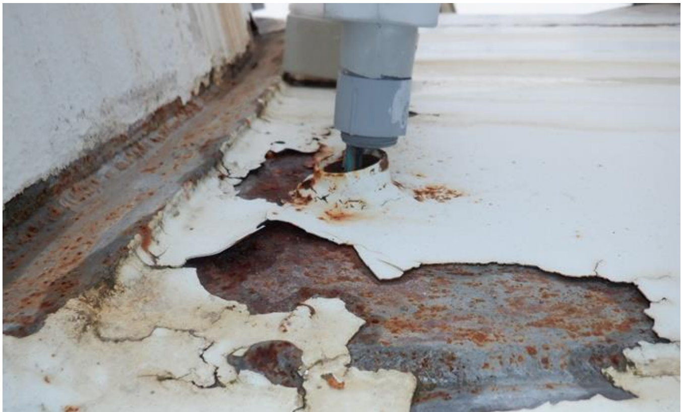
20. Coating failure on bottom tank section roof.
