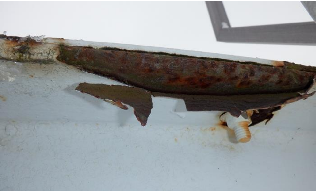
40. Coating failure and corrosion along top tank section roof-to-shell connection.
