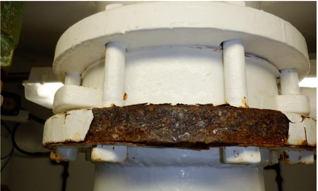
56. Corrosion on piping in bottom tank section interior dry.
