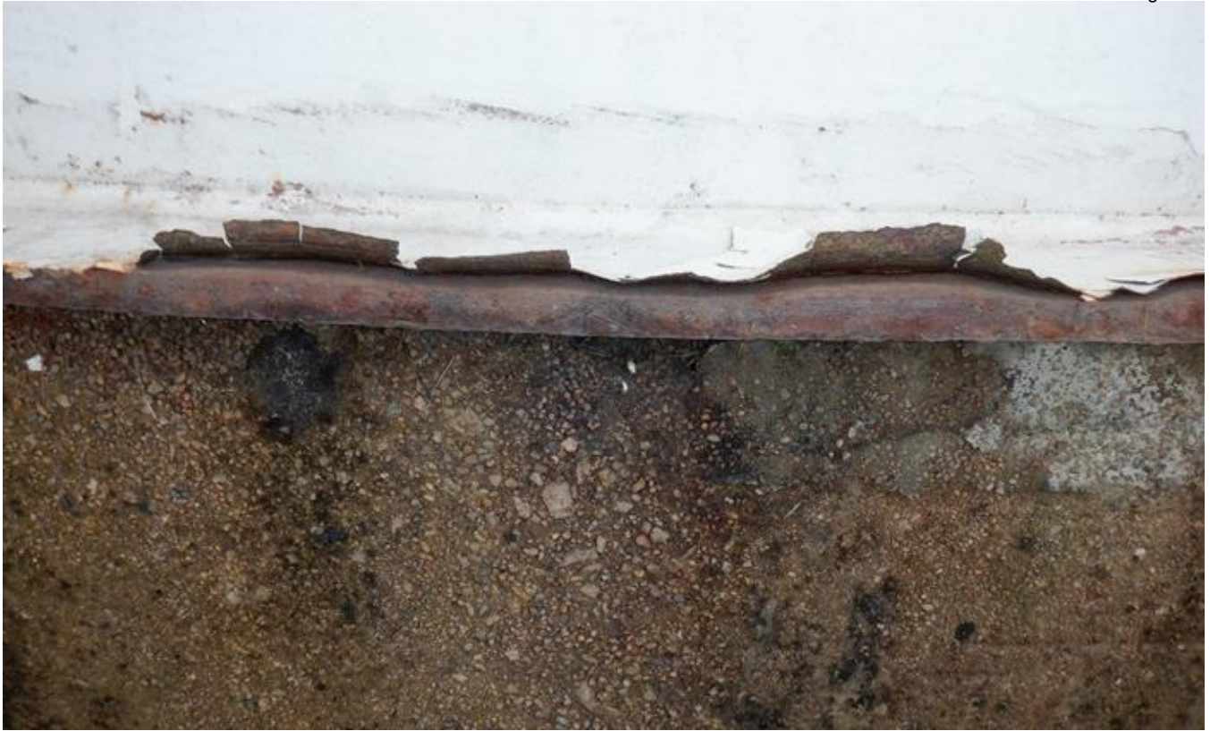
5. Corrosion and coating failure along bottom plate edge.
