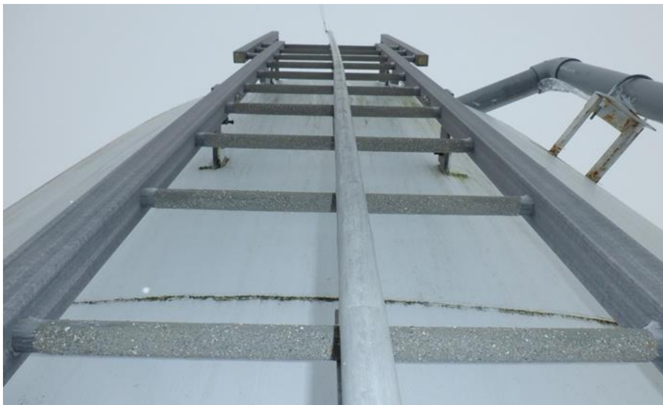
28. Middle tank section ladder and safe-climbing device.
