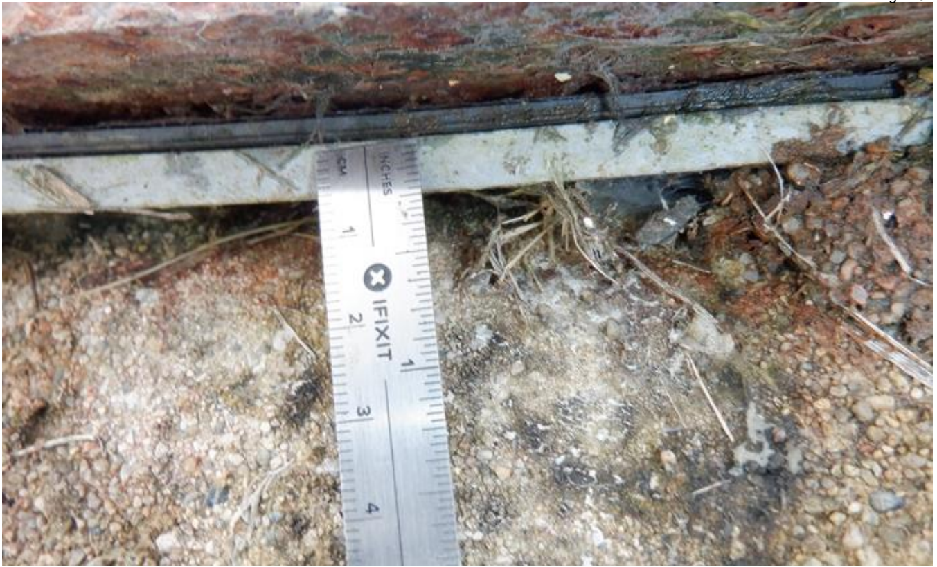
3. Gap between bottom plate and foundation.
