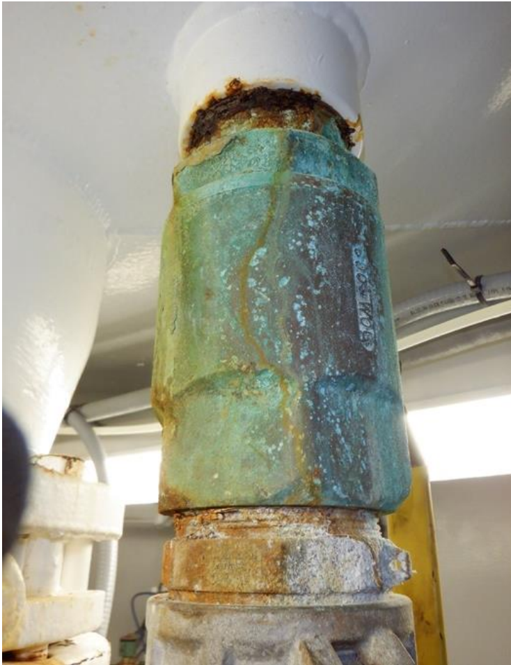
55. Corrosion on piping in bottom tank section interior dry.
