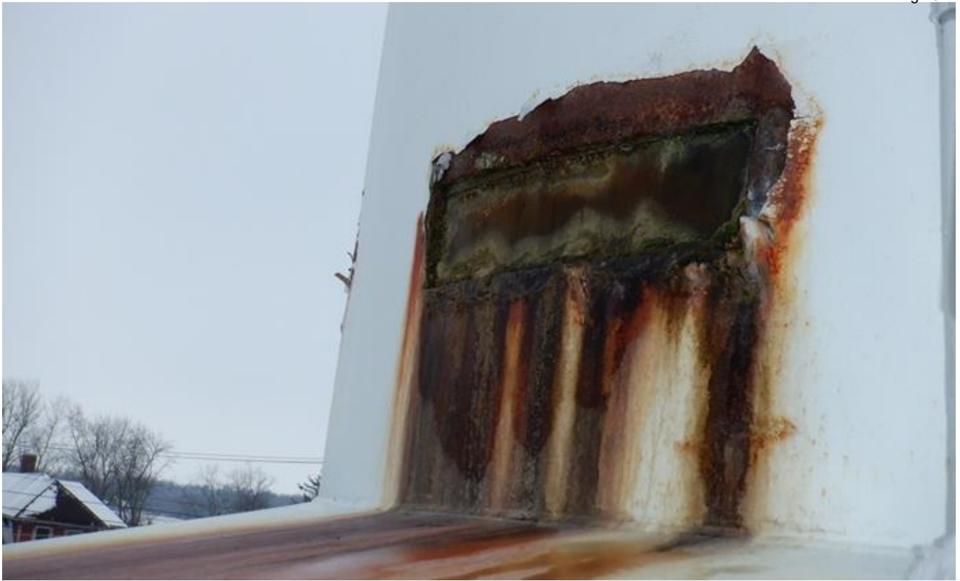
37. Corrosion around air intake in shell of top tank section.
