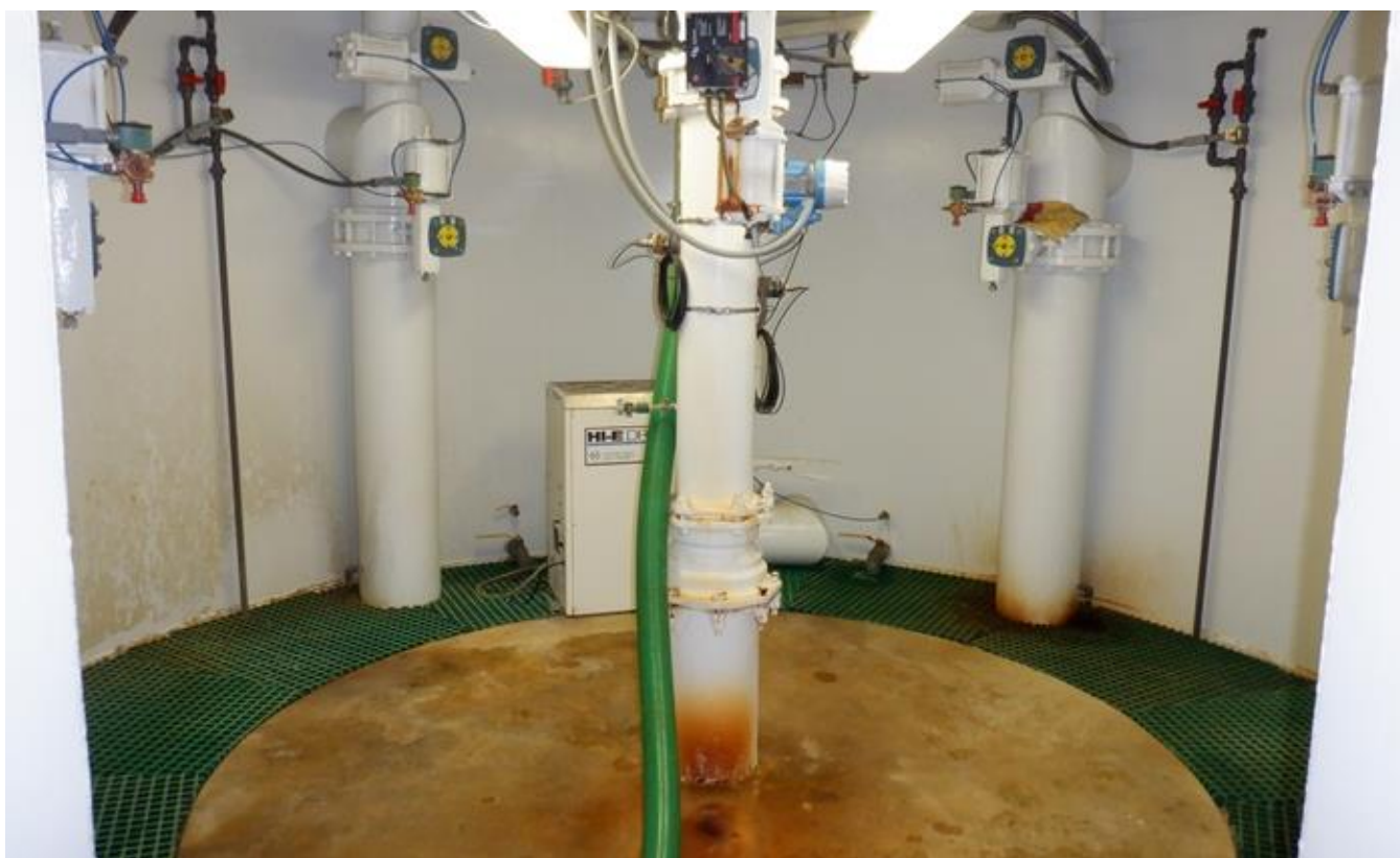
52. Piping in bottom tank section interior dry.
