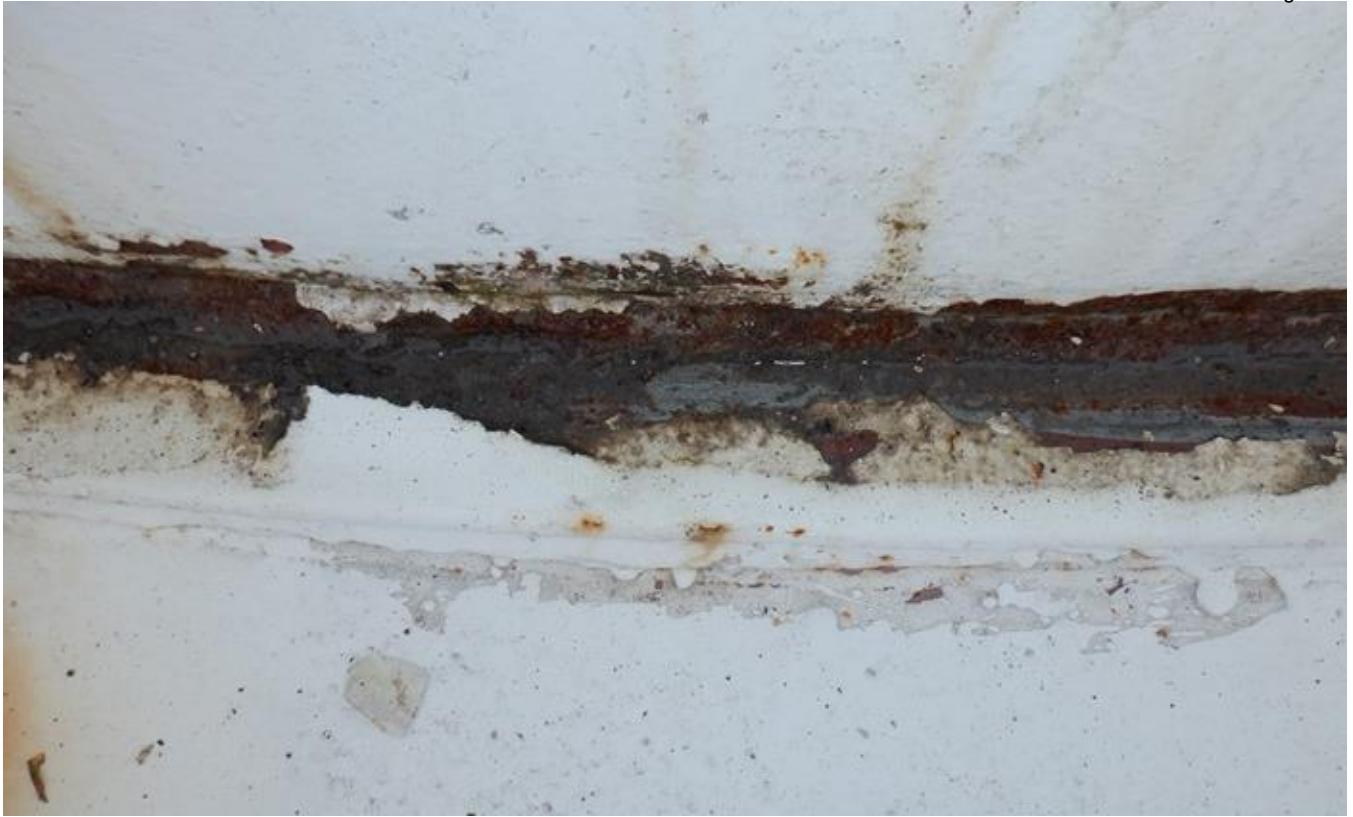
19. Corrosion along bottom-to-middle tank section connection.
