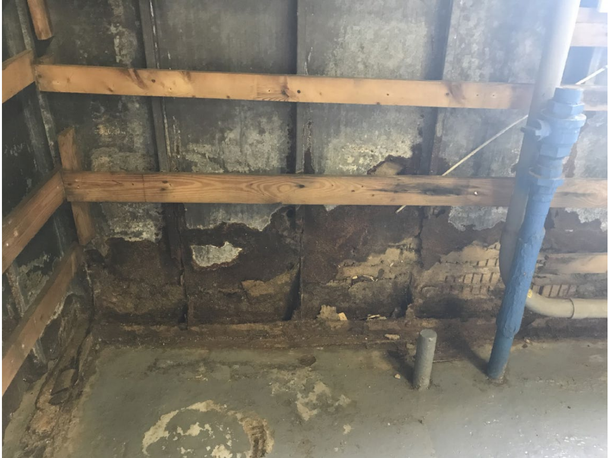
Exhibit 1-4: Photo of deterioration on exposed interior of western wall
