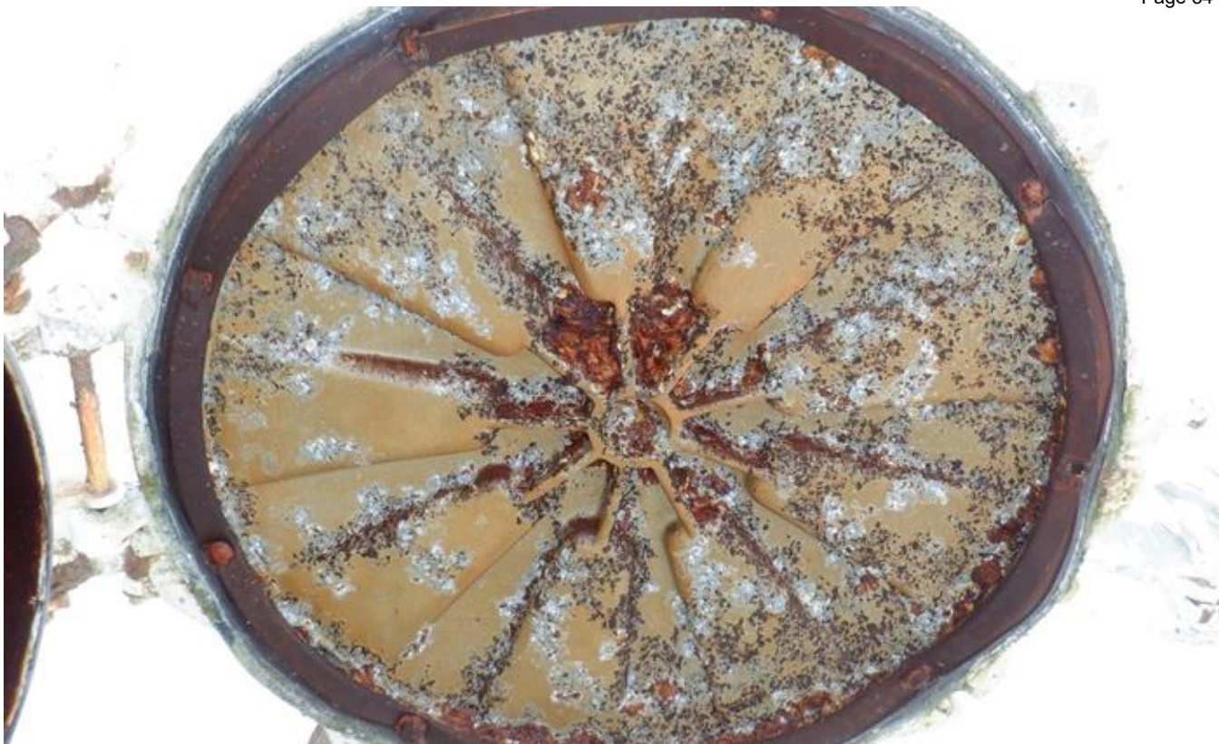
31. Corrosion on middle section roof manhole cover.
