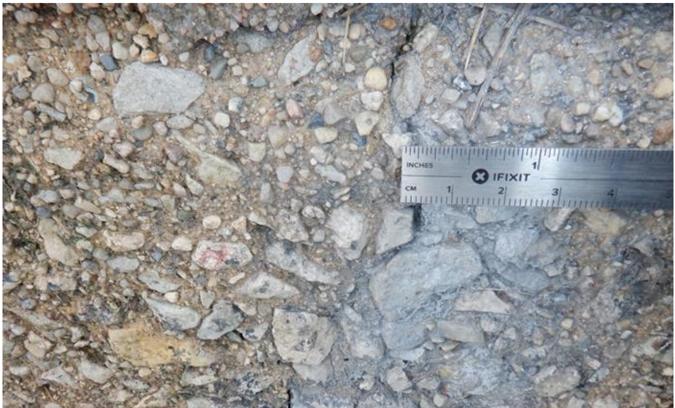
4. Crack in foundation.
