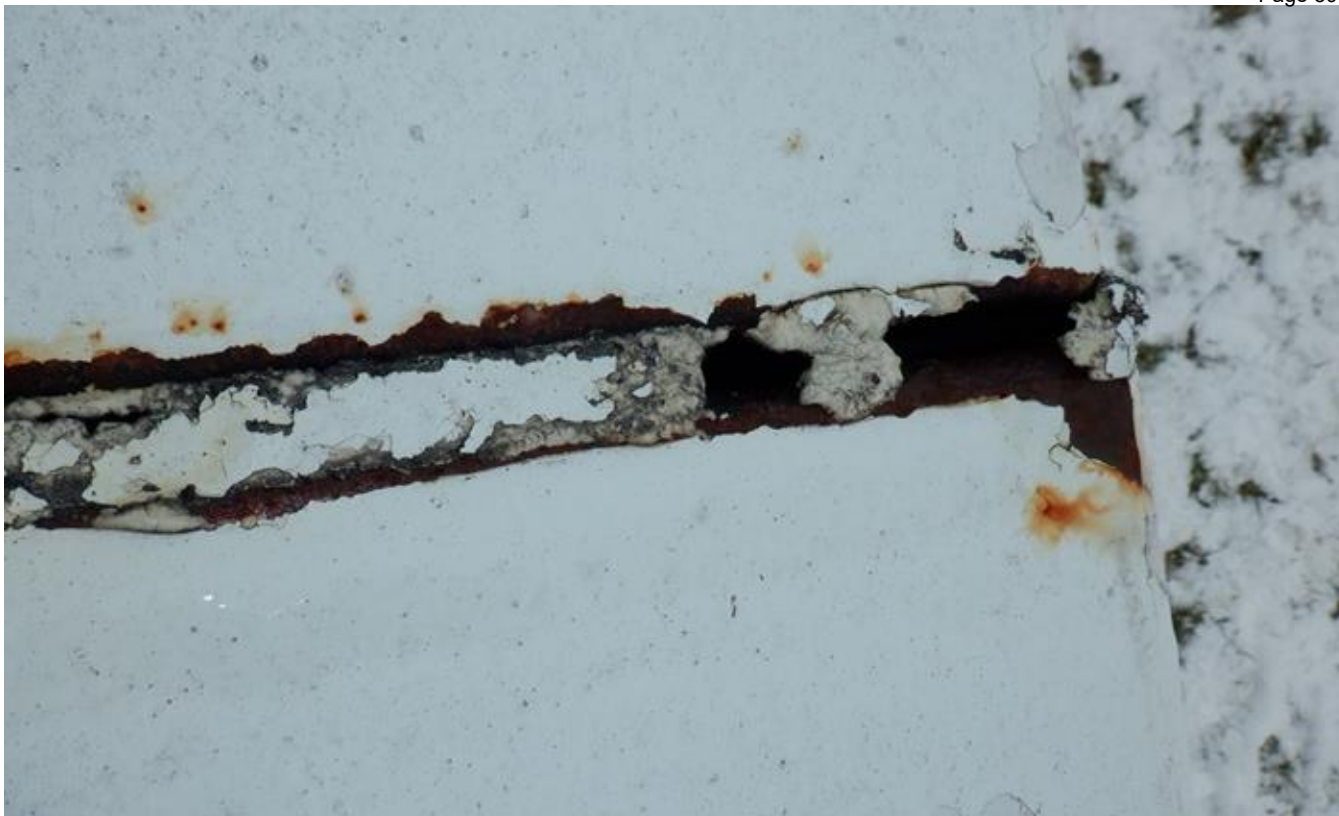
23. Hole in bottom plate roof seam.
