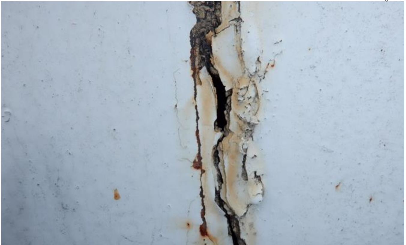
9. Crack in shell coating.
