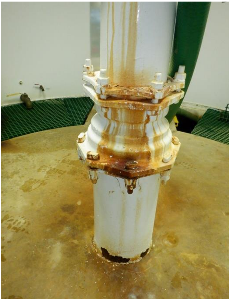
53. Rust staining on piping in bottom tank section interior dry.
