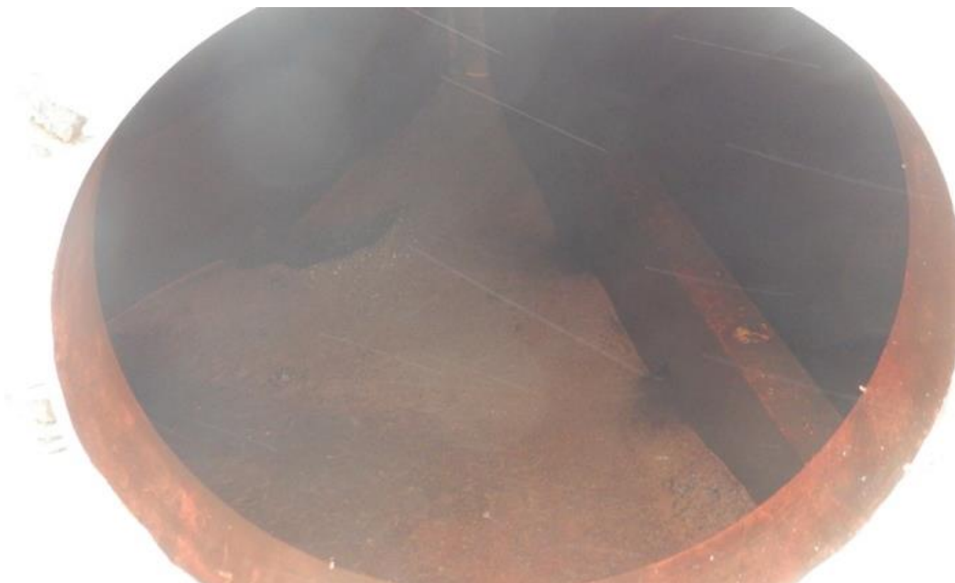
32. Corrosion on middle section roof manhole interior curb.
