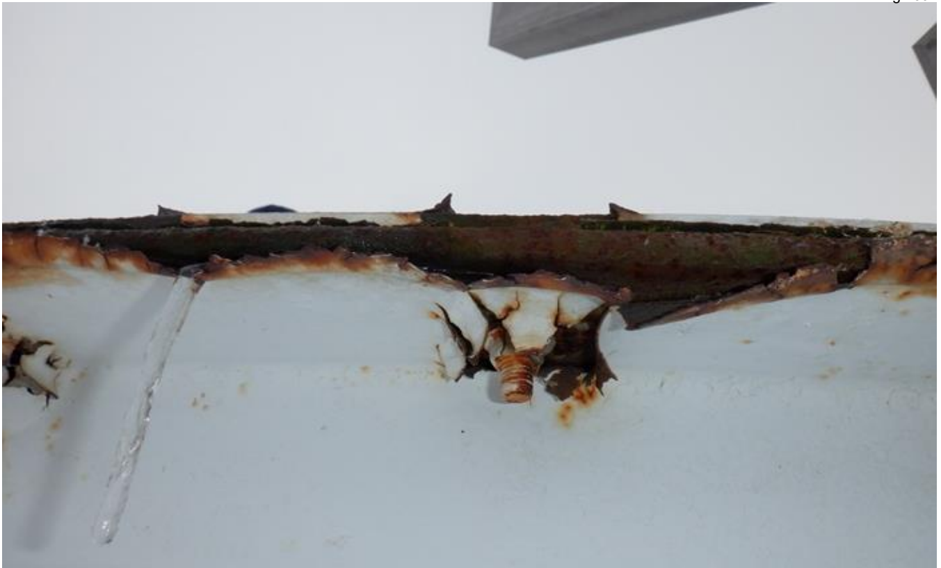
41. Coating failure and corrosion along top tank section roof-to-shell connection.
