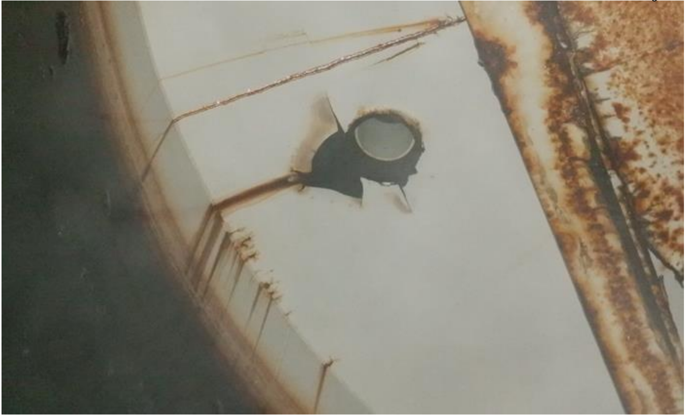
59. Corrosion and coating failure around middle tank section roof manhole opening.
