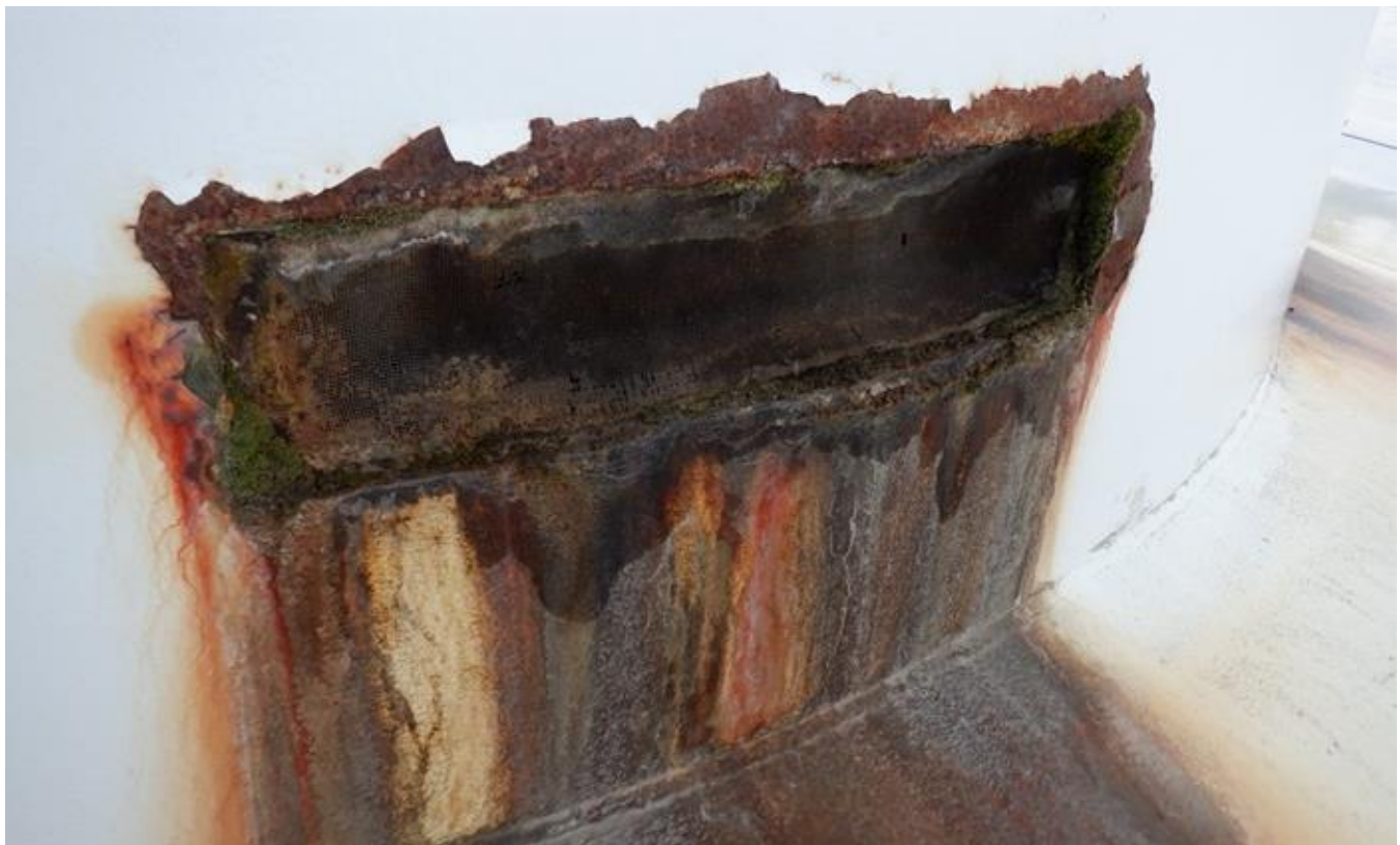
38. Corrosion around air intake in shell of top tank section.
