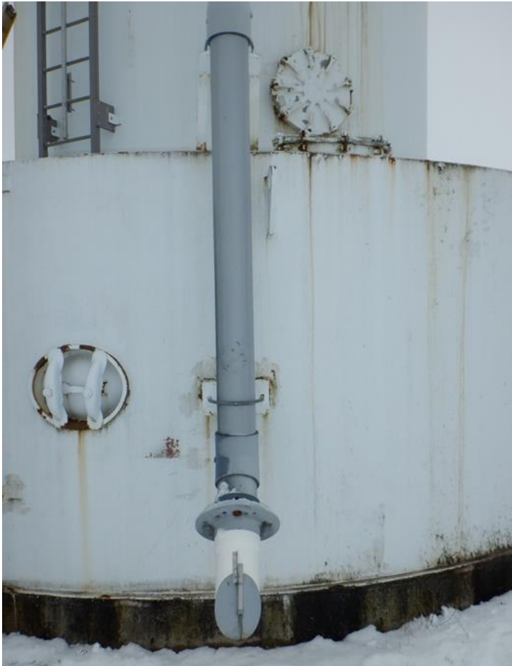
13. Overflow pipe and flap gate.
