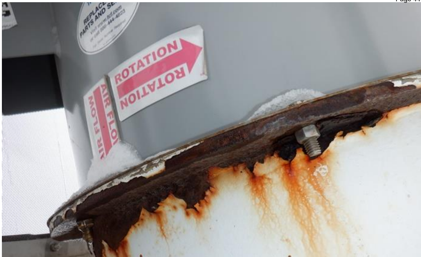
51. Corrosion along blower flanged connection.
