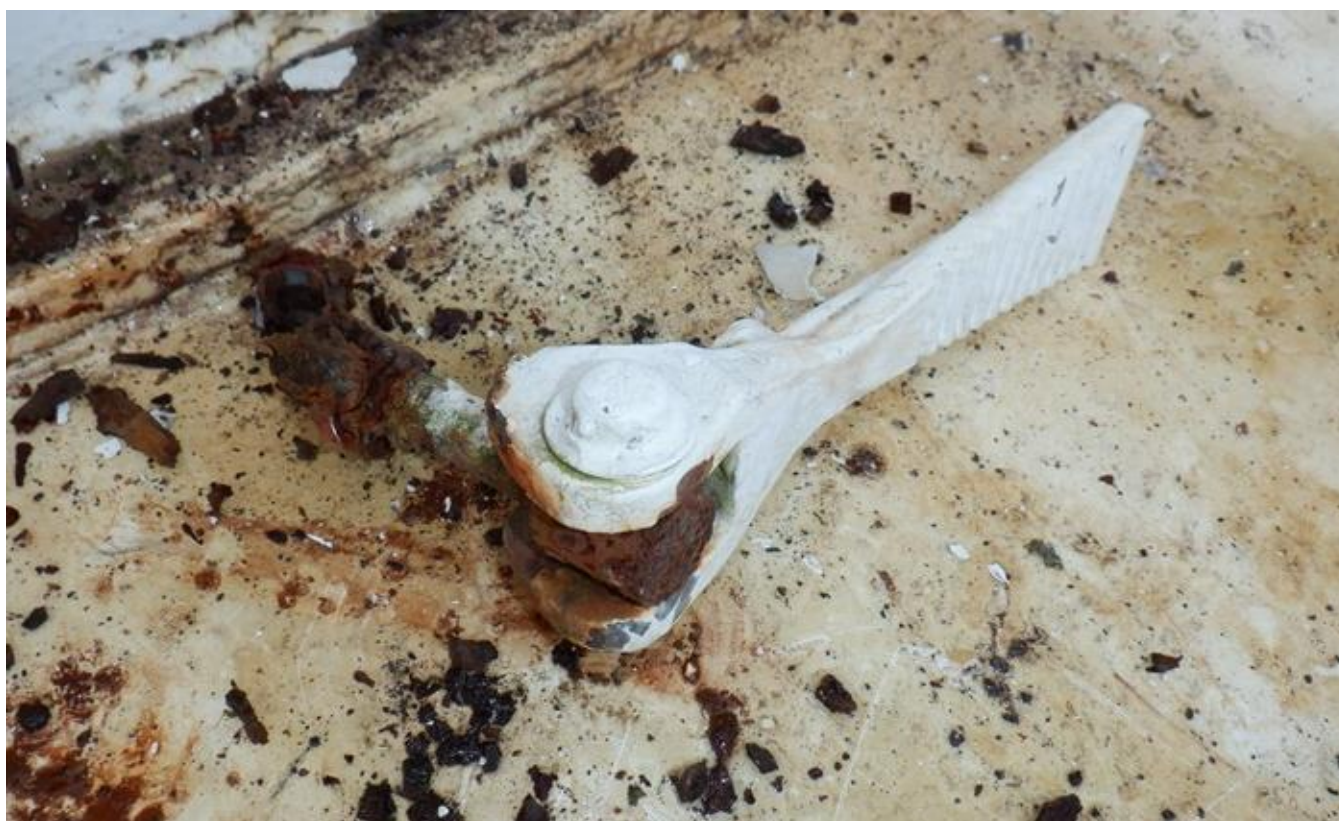
34. Detached manhole cover latch.
