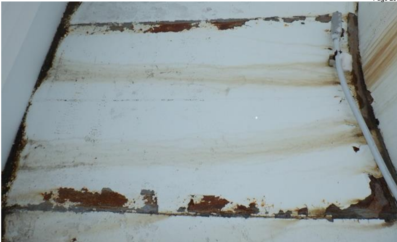
21. Coating failure on bottom tank section roof.
