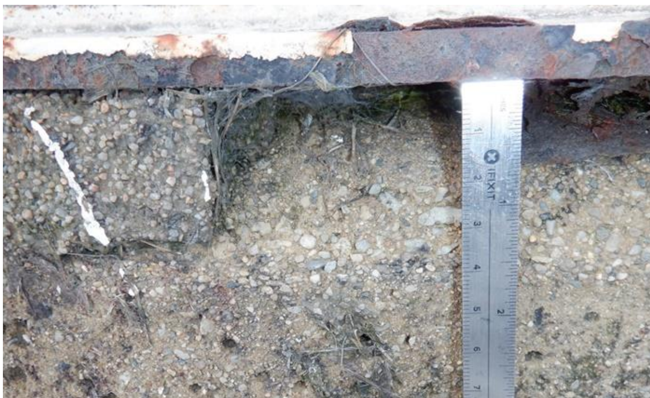
2. Gap between bottom plate and foundation.
