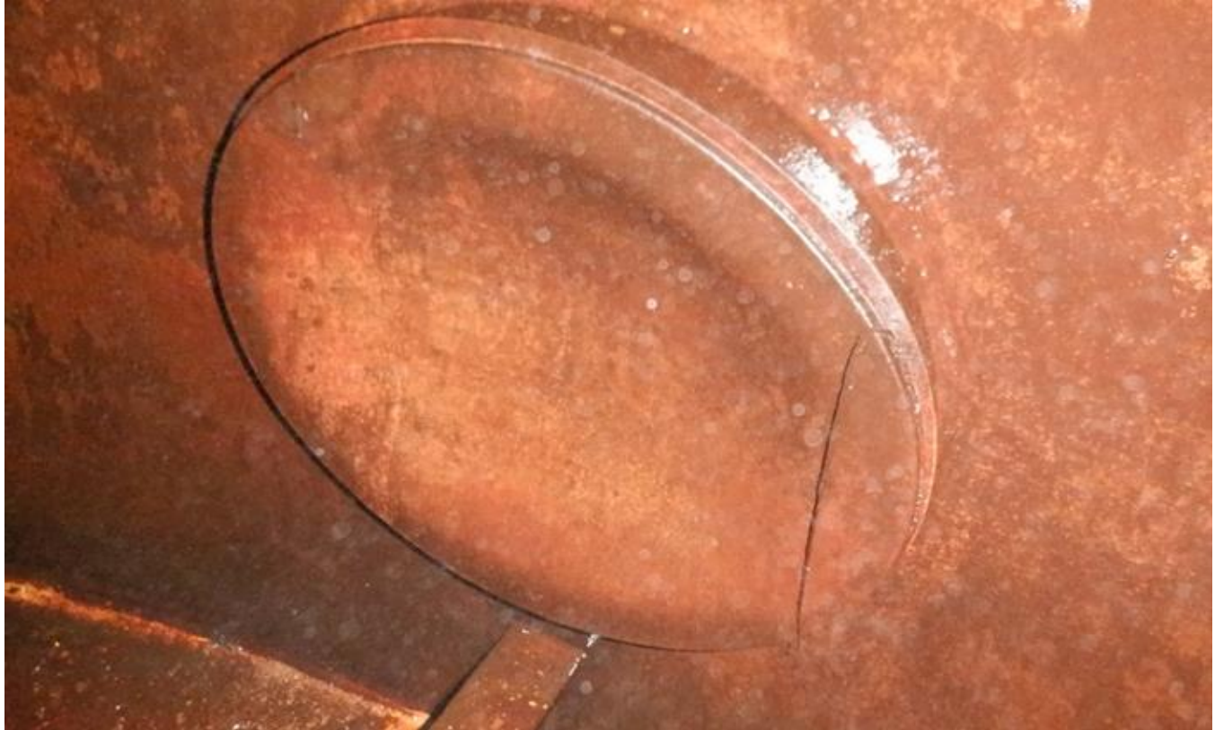
60. Mineral staining on middle section shell manhole cover.
