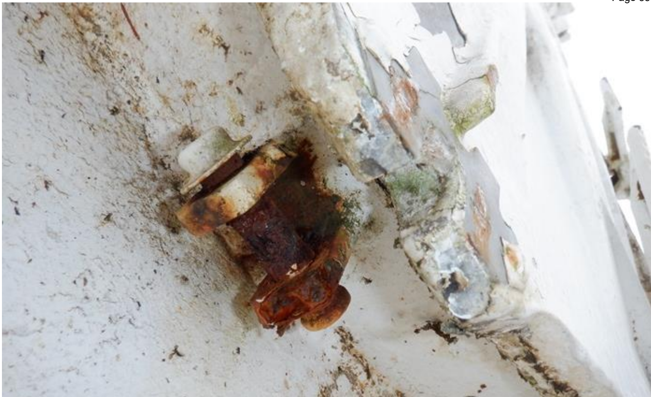
33. Corrosion on middle section roof manhole cover latch.
