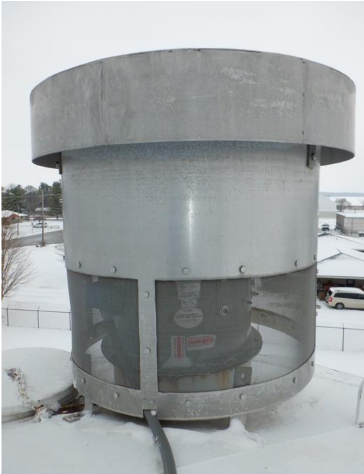
49. Blower with shroud on top tank section roof.
