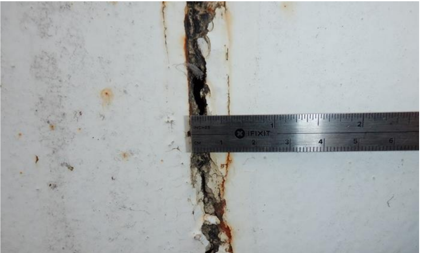
8. Crack in shell coating.
