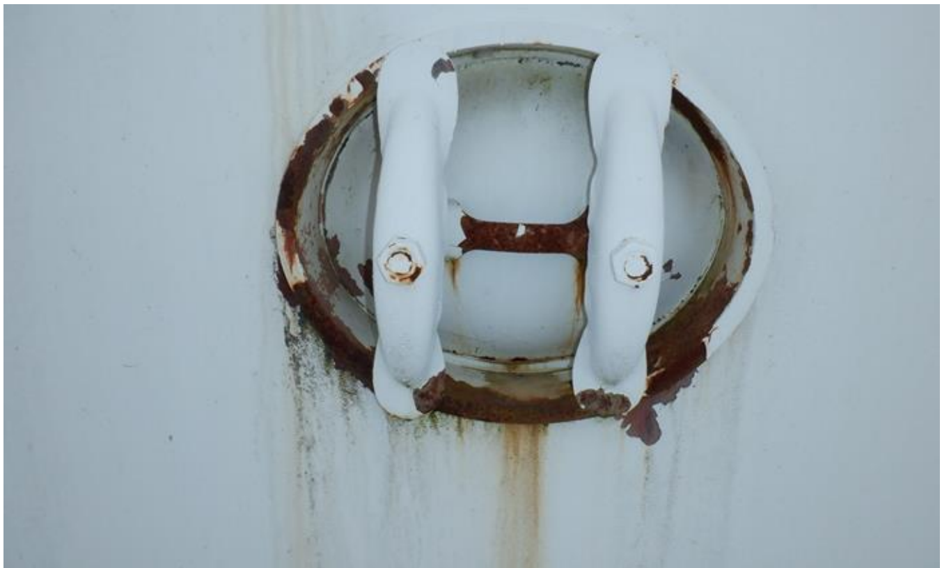
10. Corrosion on shell manhole in bottom tank section.
