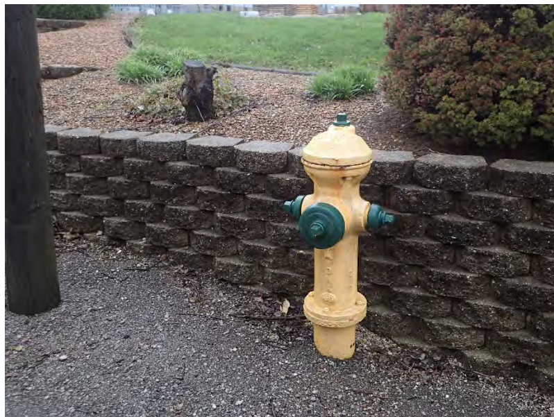
Fire hydrant without valve to be replaced
