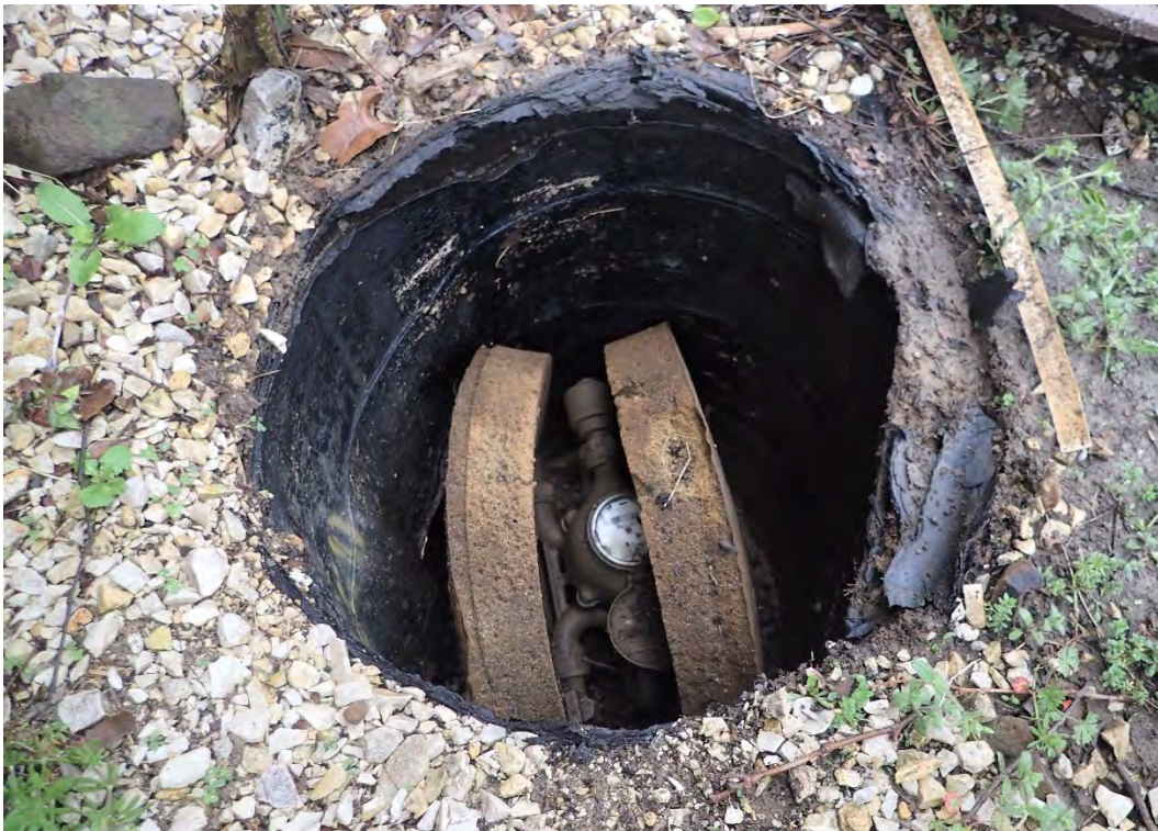
Fiber/asphalt meter pit to be replaced
