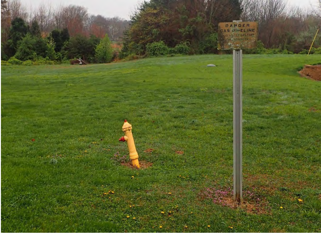
Flush hydrant to be replaced
