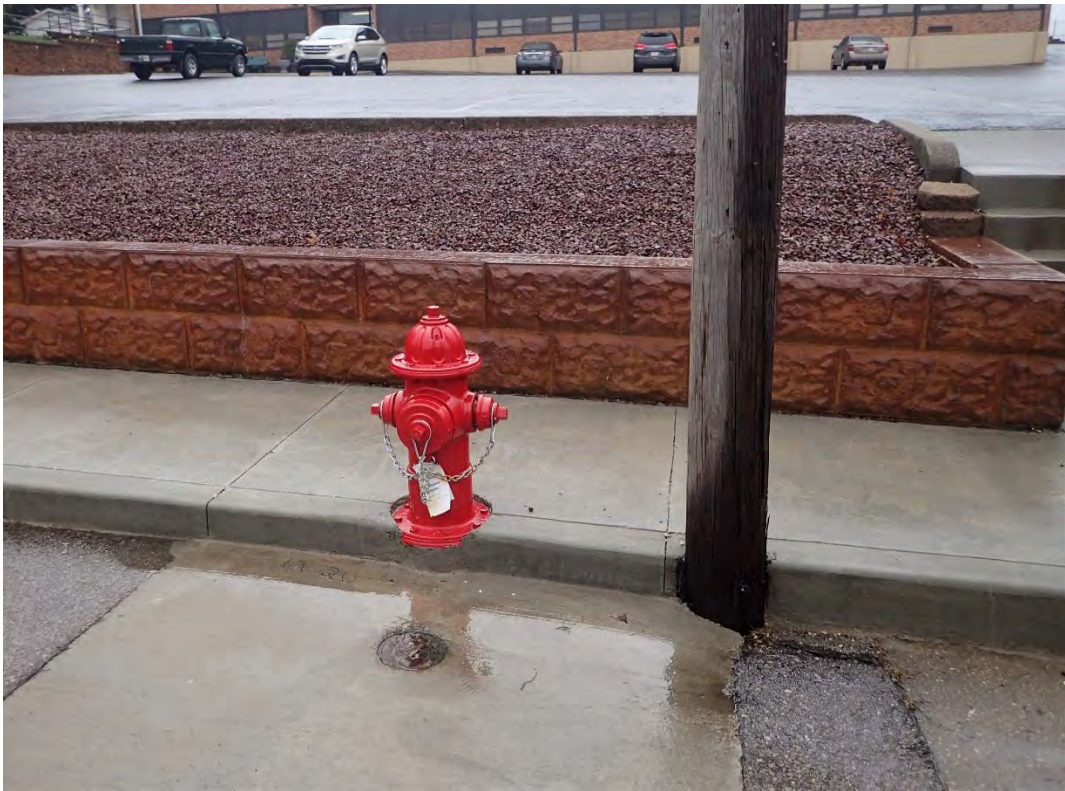
New hydrant with valve example
