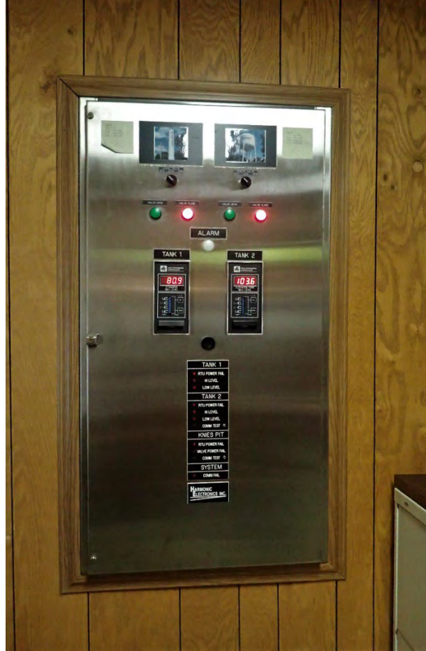
Existing SCADA panel in garage office
