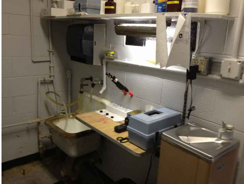
Figure 1.1.10 Laboratory at Wheeler Water Treatment Plant
