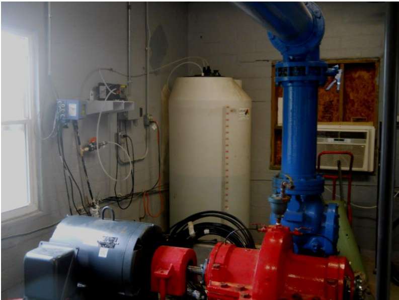
Figure 5 High service pump and motor, chemical feed in corner.
