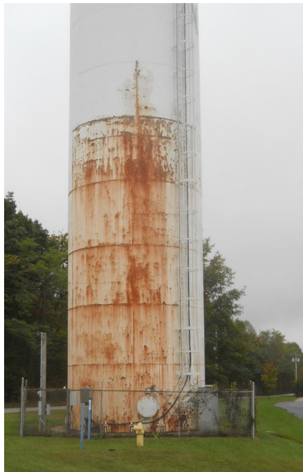
Figure 2 Standpipe rust and coating failure
