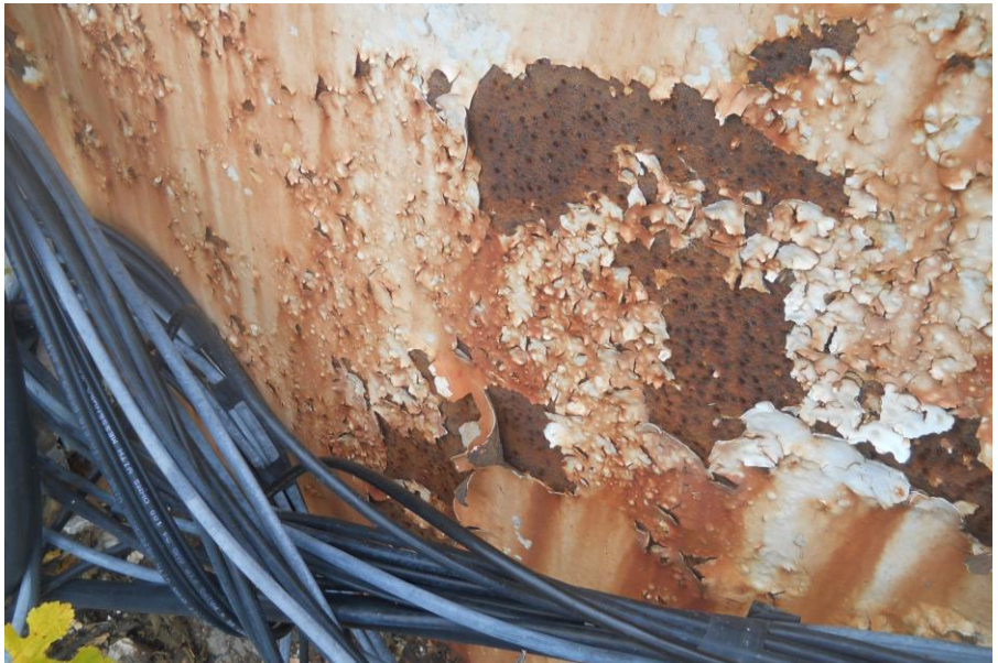
Figure 7 Standpipe lower section with coating failure and corrosion.
