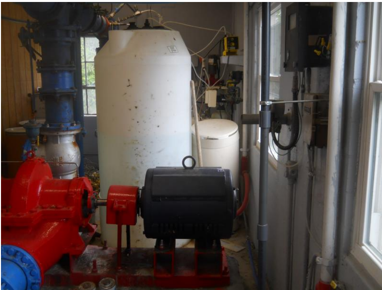
Figure 7 High service pump (red) and motor, Clearitas tank
