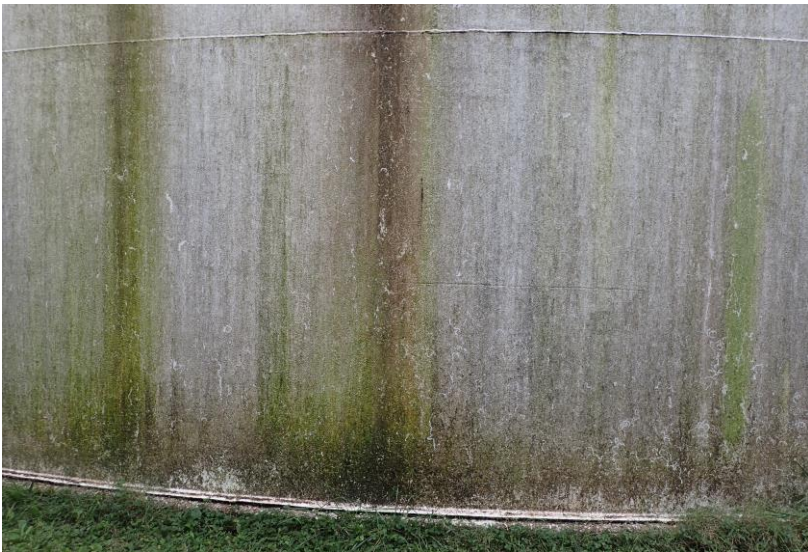
Figure 13 – 1.5 MG GST showing rust streaks. Oct. 12, 2017
