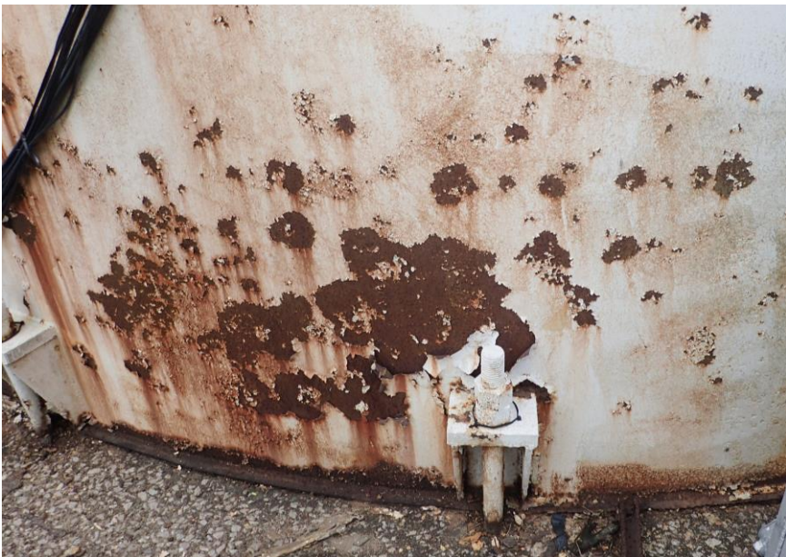
Figure 6 Surface rust and pitting including chine corrosion (bottom).
