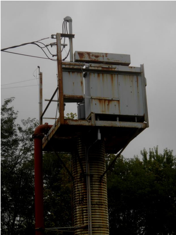
Figure 5 Elevated well platform close-up
