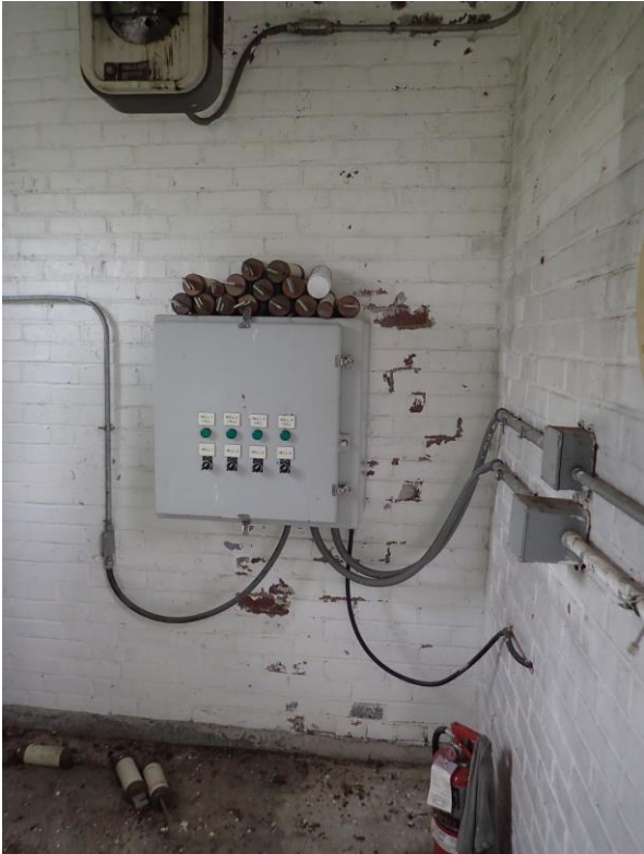
Figure 7 Inside view - Control Building
