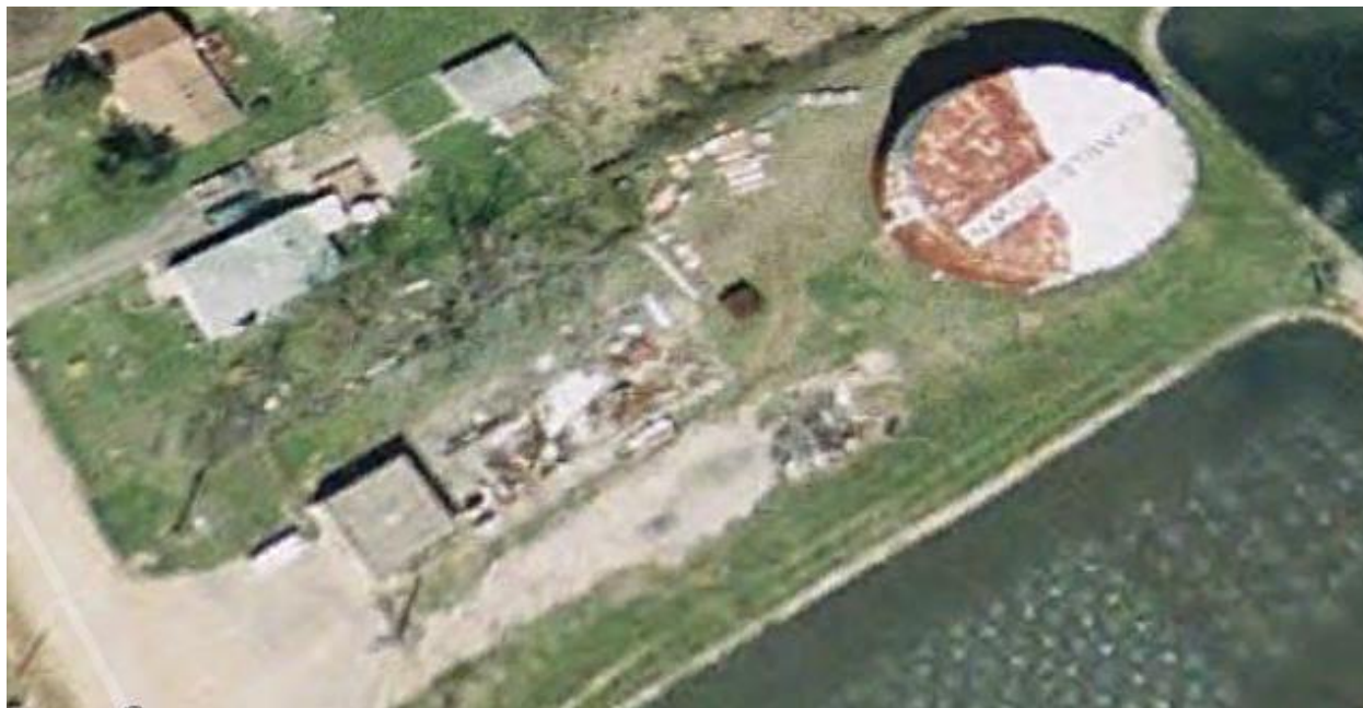
Figure 1 - December 2002 – Aerial of Charlestown’s 1.5 MG Ground Storage Tank showing extensive rusting of the roof and west half of the tank steel. Also shown is the Pump Building.
