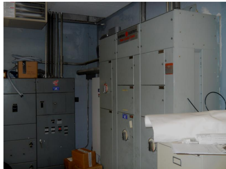
Figure 4 Pump Building Motor Control Center
