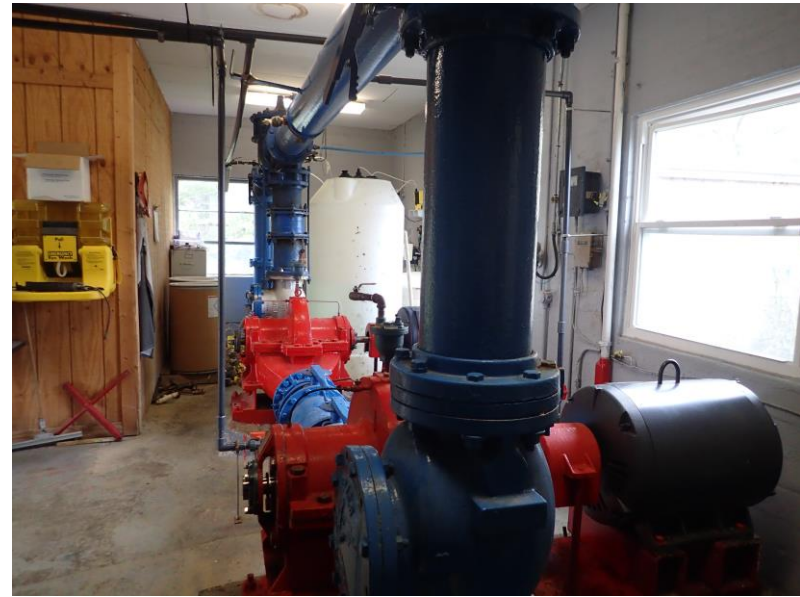
Figure 6 High service pumps and motor, overhead discharge pipe.
