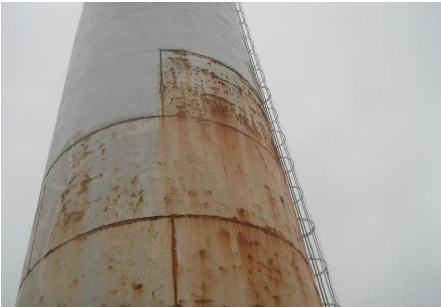
Figure 5 Rusty welds and plate steel (10/12/17 photos)
