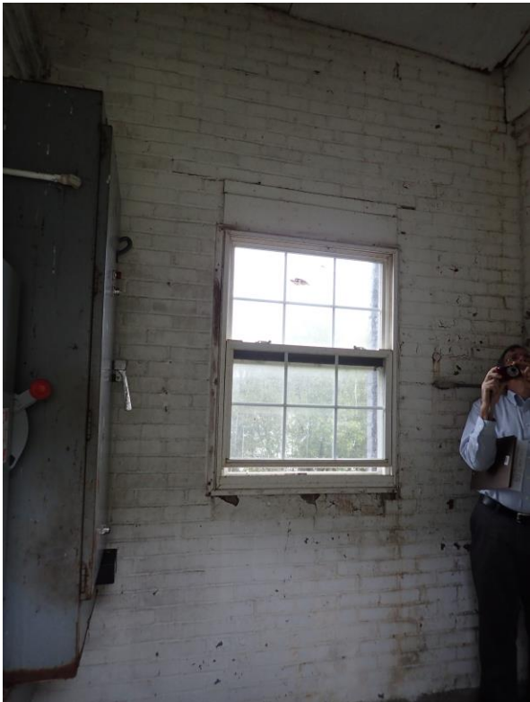
Figure 8 Inside view - Control Building
