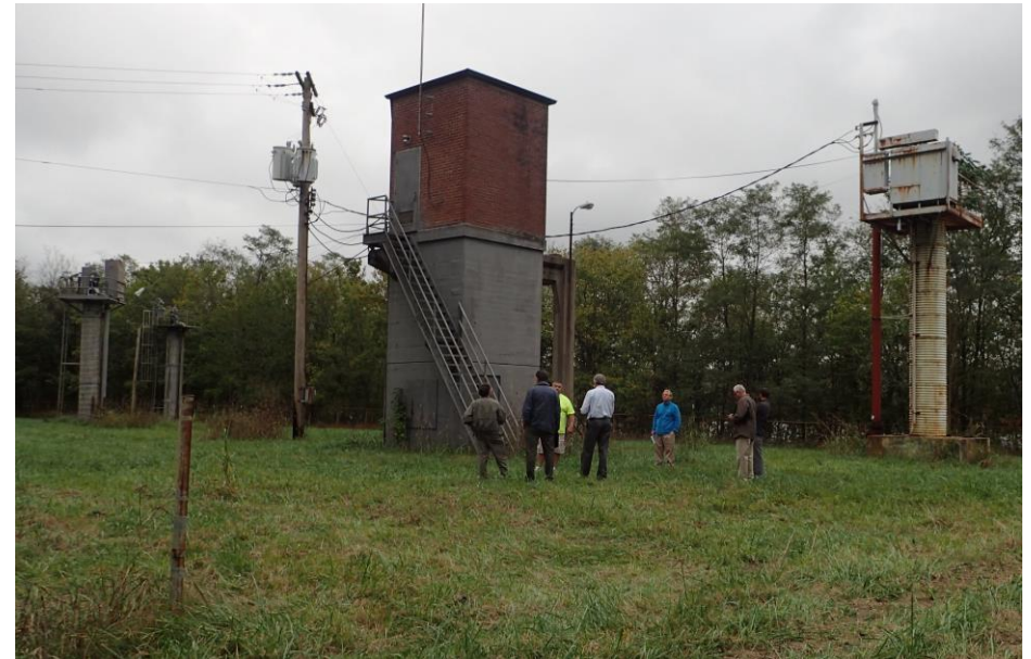
Figure 4 Well platforms and Control Building (three wells shown)
