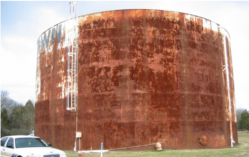
Figure 9 – 1.5 MG GST showing extensive rust. Photo taken in 2005.
