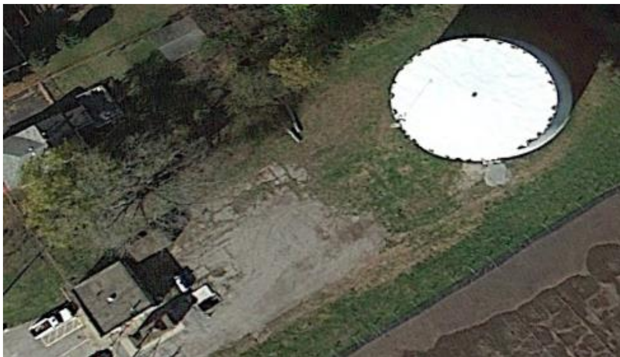
Figure 4 – November 2013 – Aerial of Charlestown’s 1.5 MG Ground Storage Tank showing the tank has been repainted. Note that the roof shows rust pockets at the roof-wall interface.
