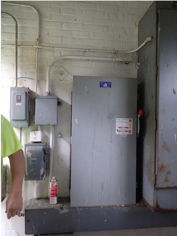
Figure 6 Control Bldg. electrical / controls
