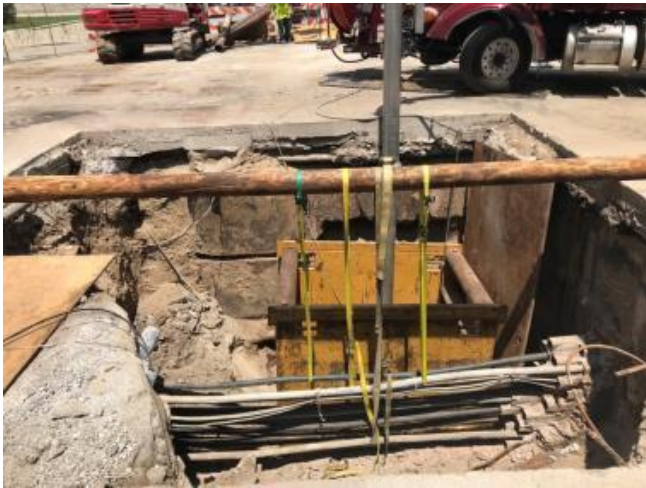
Pennsylvania Ave & Ohio St Sewer Failure
