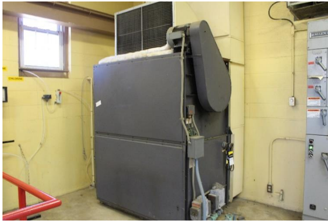
FIGURE 3. NON-WORKING HVAC TO BE DEMOLISHED
