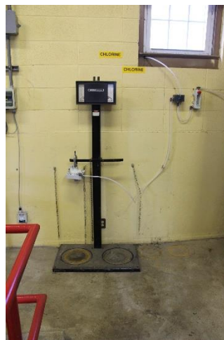
FIGURE 1. EXISTING DISINFECTANT FEED
