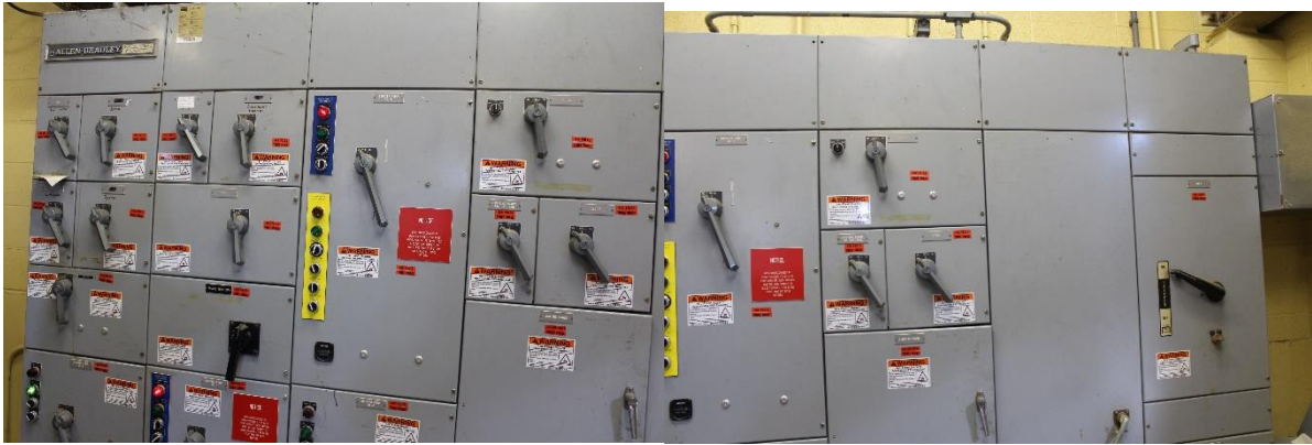
FIGURE 1. EXISTING MOTOR CONTROL CENTER AND TRANSFORMER
