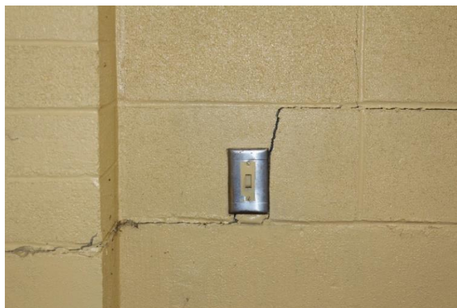
FIGURE 2. INTERIOR BLOCK REPAIR NEEDS
