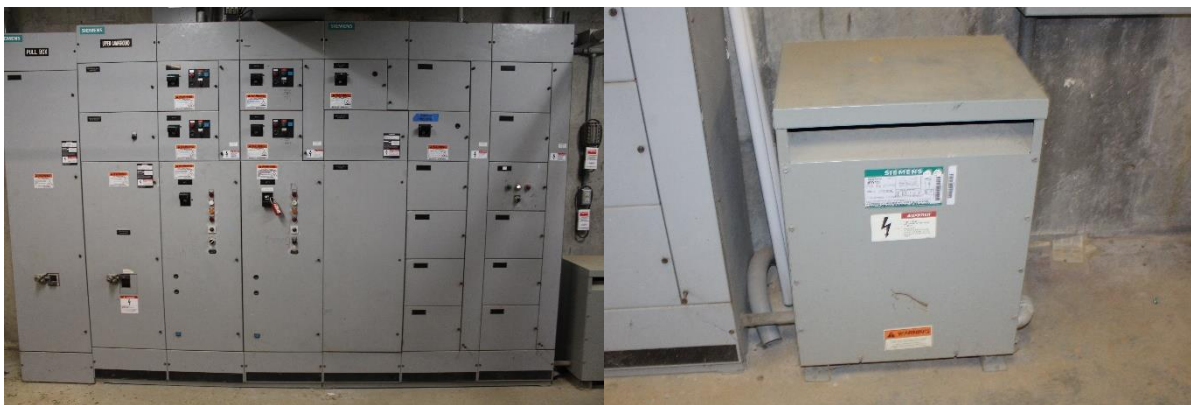
FIGURE 1. EXISTING MOTOR CONTROL CENTER AND TRANSFORMER
