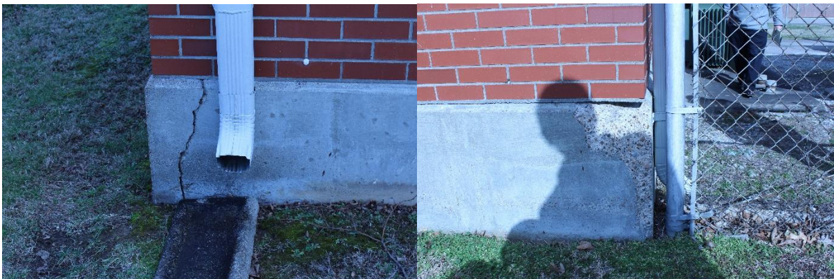
FIGURE 1. FOUNDATION REPAIR NEEDS
