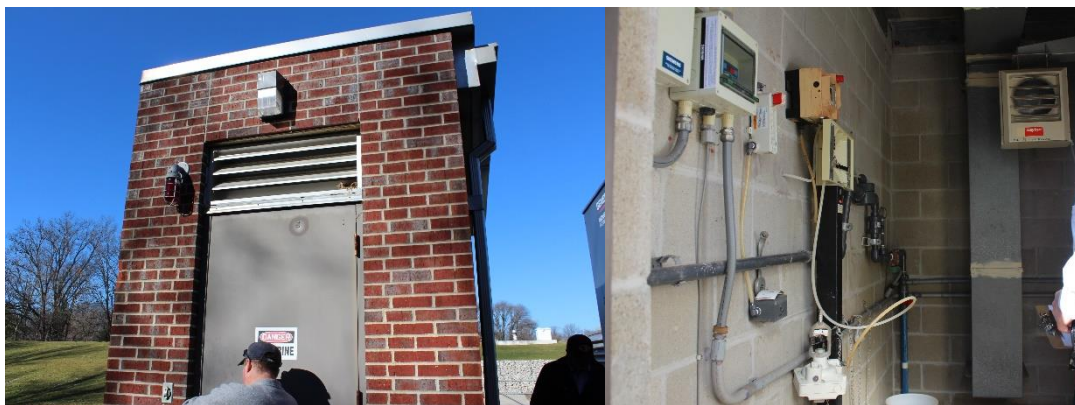
FIGURE 1. EXISTING DISINFECTANT FEED
