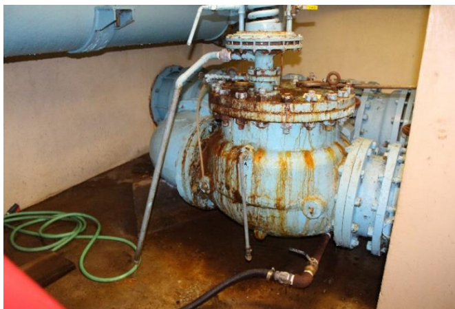
FIGURE 4. EXISTING ALTITUDE VALVE
