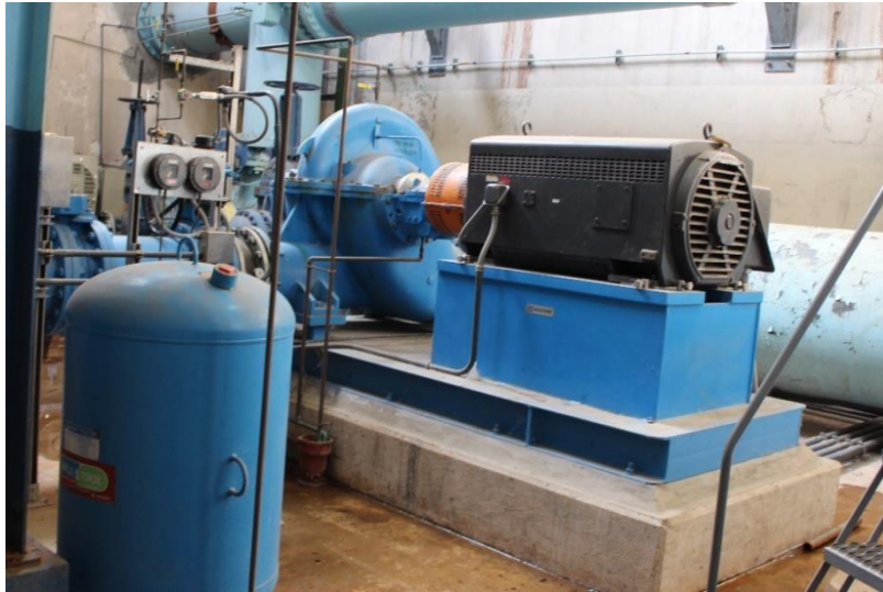
FIGURE 2-17 Emergency Valve Closure System Water Storage Tanks
