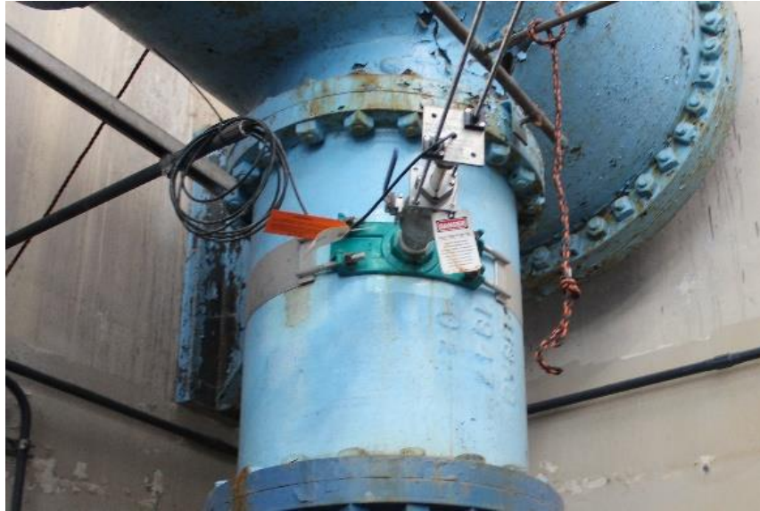
FIGURE 2-15 HSP No. 7's Flow Sensor
