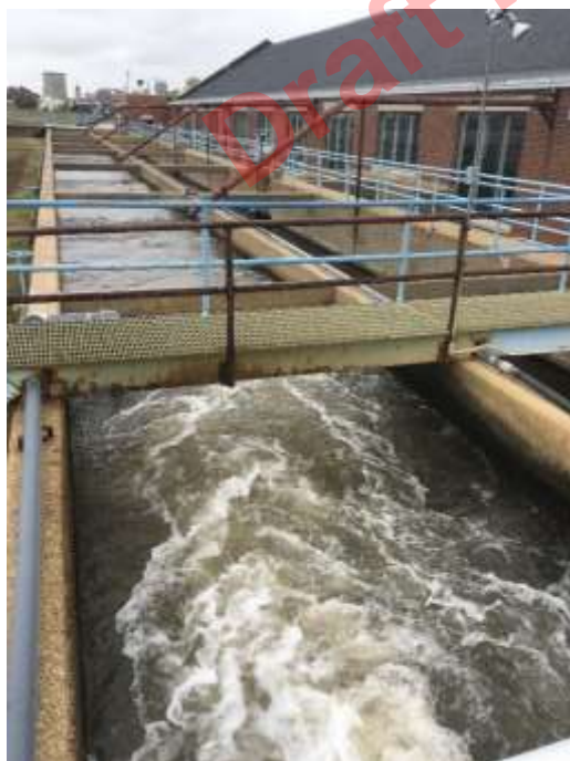
FIGURE 2-3 Raw Water Flume
