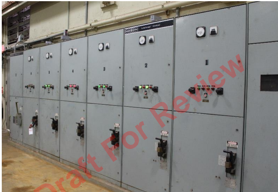
FIGURE 2-5 Low Service Pump Station Switchgear
