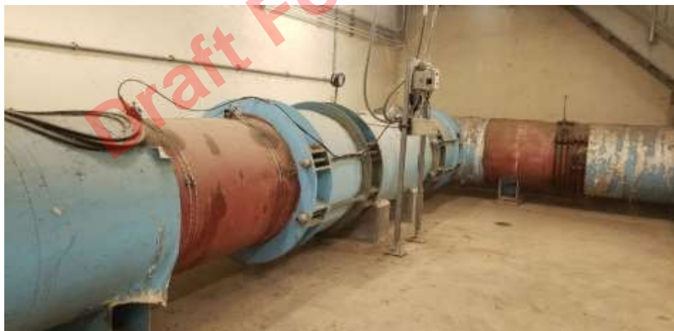
FIGURE 2-29 Effluent Piping in High Service Pump Station No. 3
