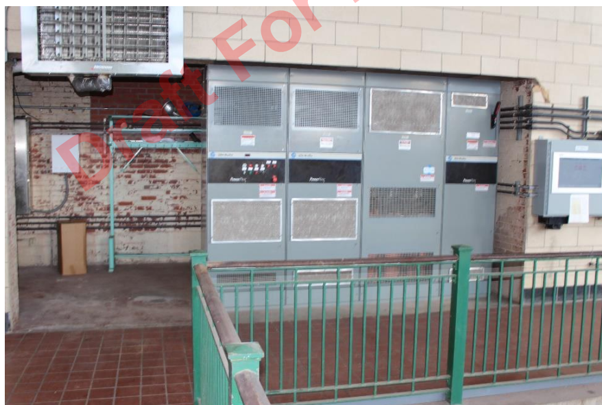
FIGURE 2-14 VFD for HSP No. 5
