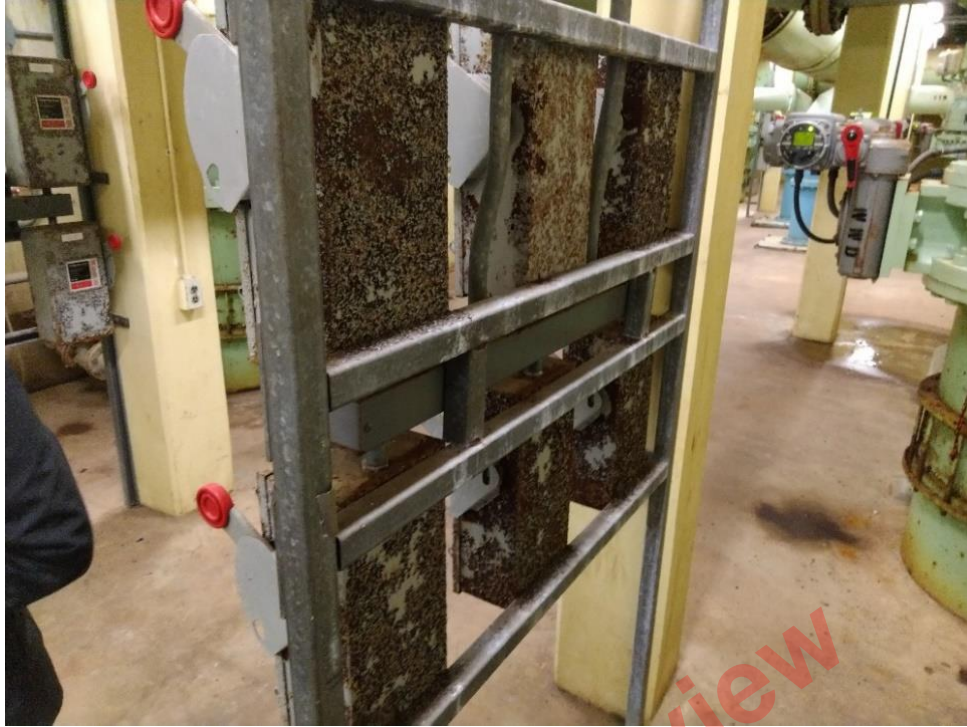
FIGURE 2-10 Electrical Enclosure Corrosion
