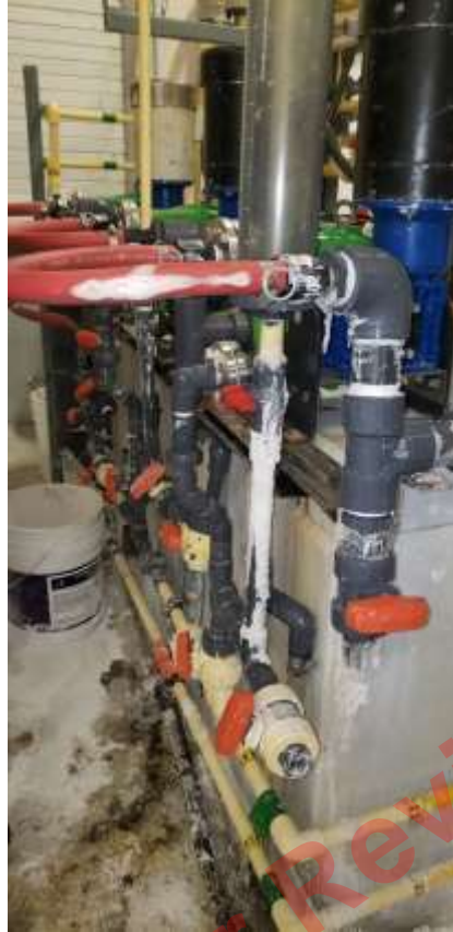
FIGURE 2-19 Leaking Caustic Chemical Feed System
