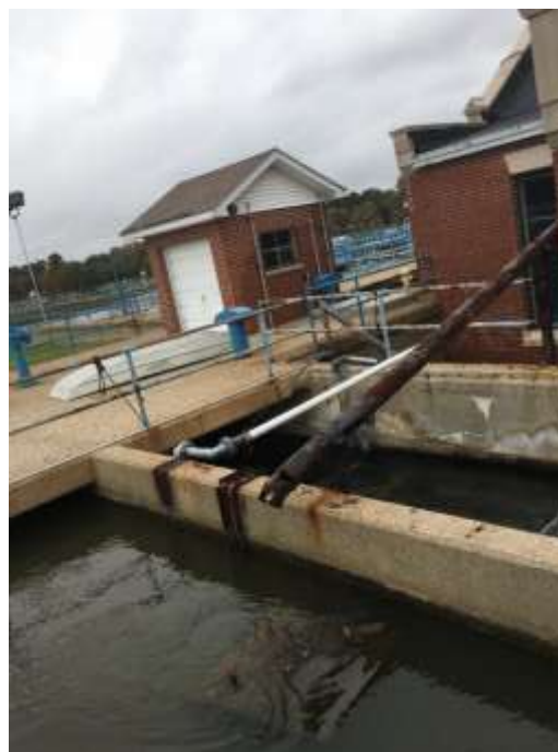
FIGURE 2-4 Corroded Roof Drain Downspout
