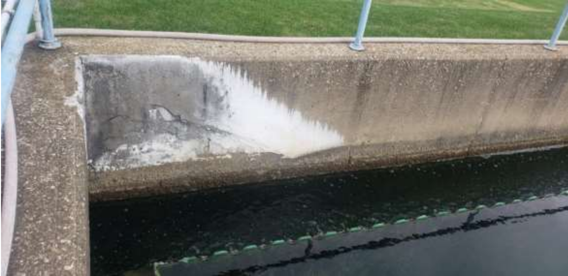
FIGURE 2-7 Concrete Surface Deterioration (Previously Repaired)
