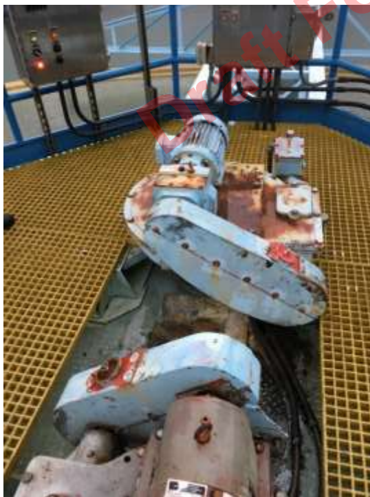
FIGURE 2-10 Primary Clarifier Flocculator Drive
