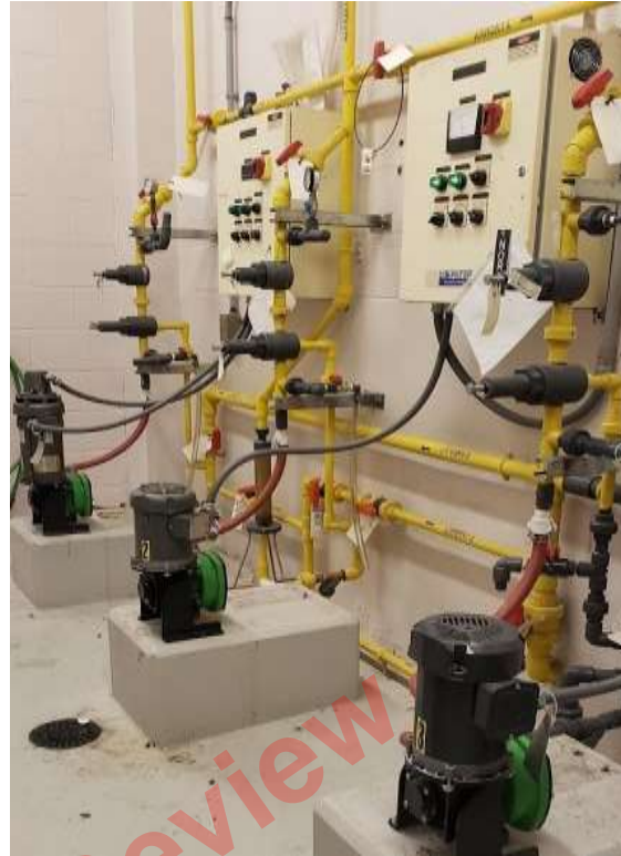
FIGURE 2-24 Ammonia Feed System
