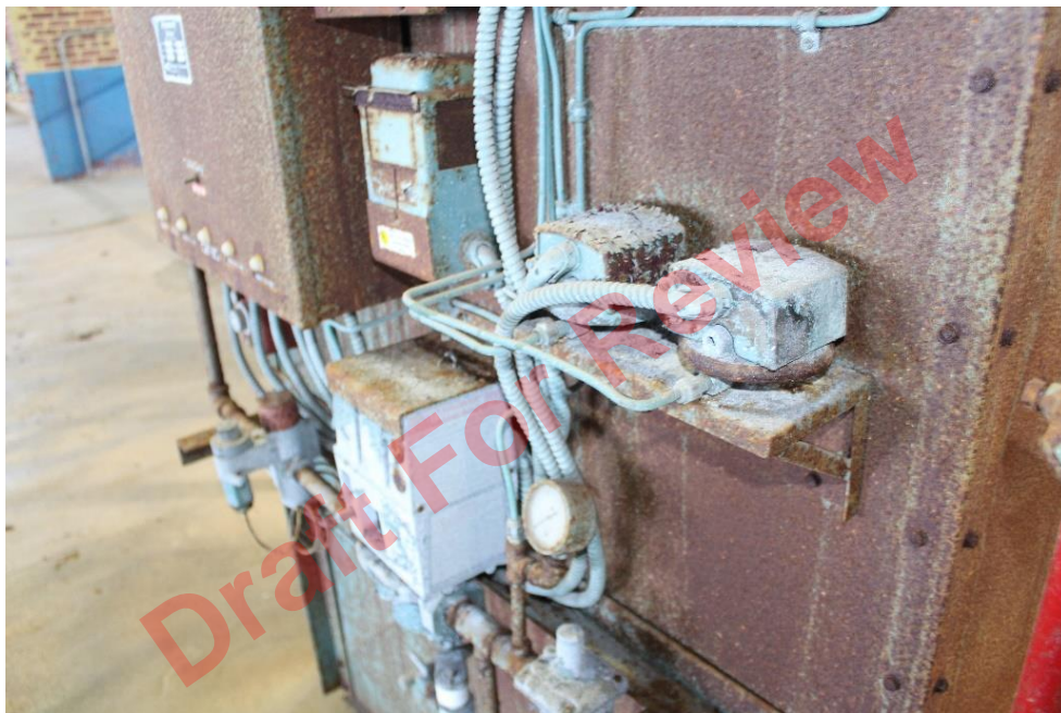
FIGURE 2-9 Exposed Electrical Equipment Corrosion
