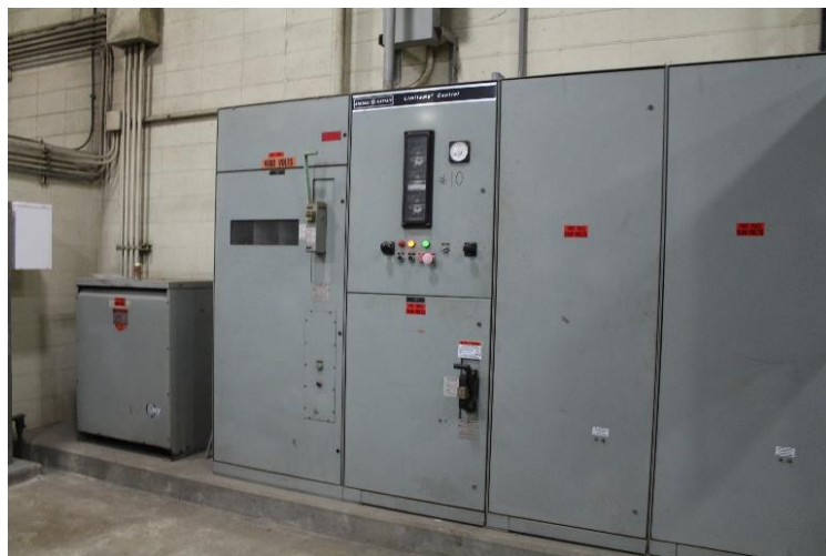
FIGURE 2-20 HSPS No. 3 Pump Controls
