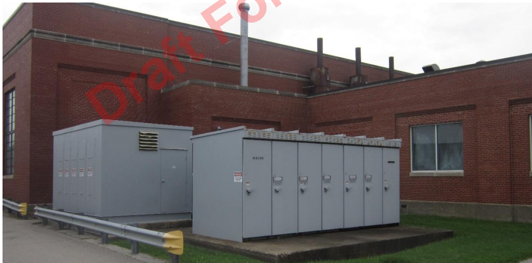
FIGURE 2-1 Generator Controls Enclosure
