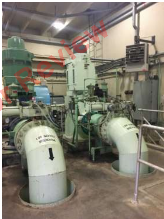
FIGURE 2-2 Low Service Pumps
