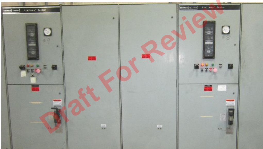
FIGURE 2-18 HSPS No. 3 Switchgear
