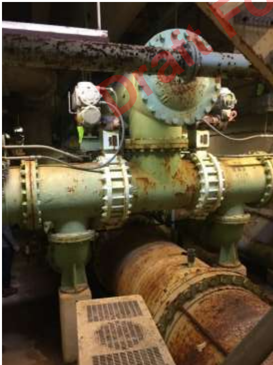
FIGURE 2-15 Corrosion in Pipe Gallery
