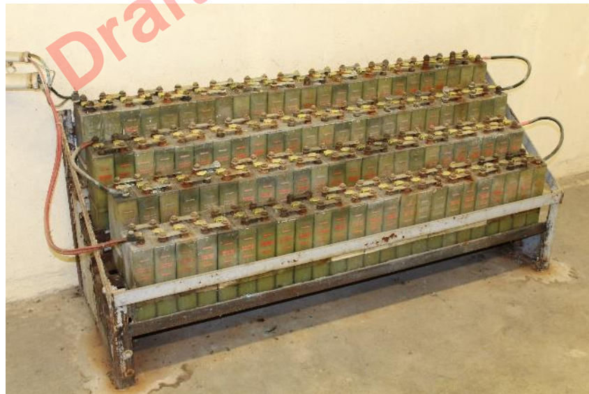
FIGURE 2-4 HSPS No. 3's Batteries for Battery Backup System
