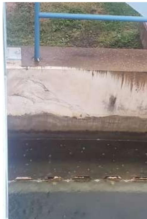
FIGURE 2-11 Primary Clarifier Concrete Degradation
