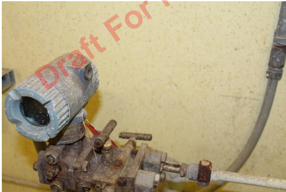
FIGURE 2-11 Pipe Gallery Controls Corrosion
