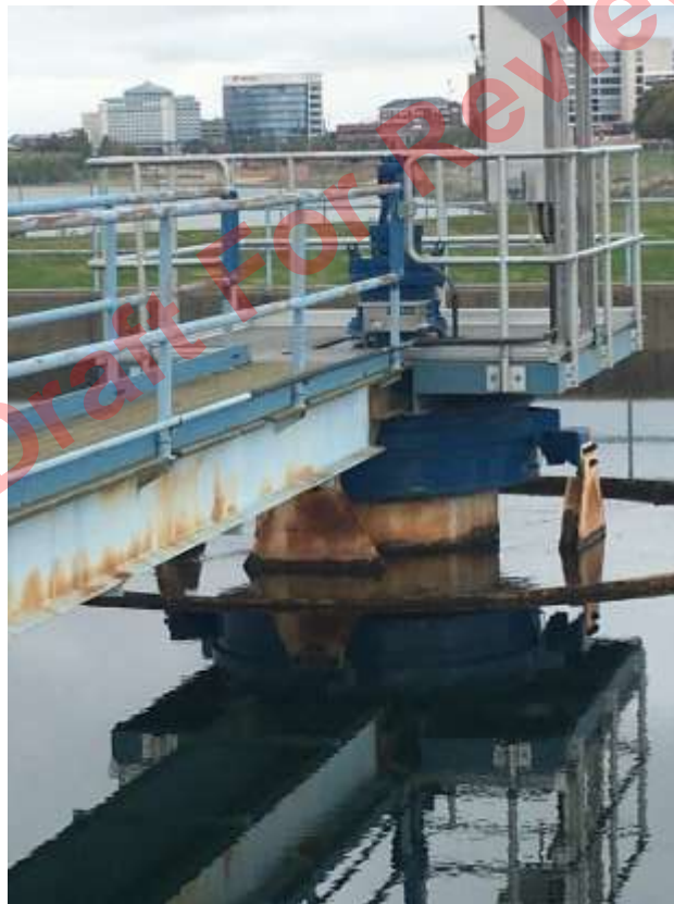
FIGURE 2-8 Support Column and Bridge Corrosion
