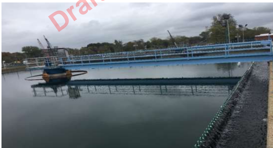
FIGURE 2-6 North Plant Primary Settling Basin
