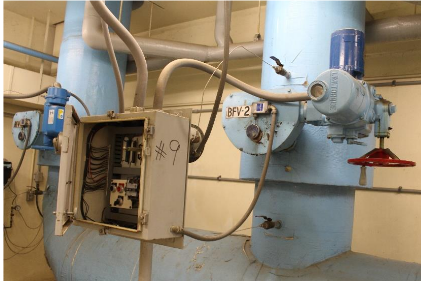
FIGURE 2-19 HSPS No. 3 Discharge Valve Actuators
