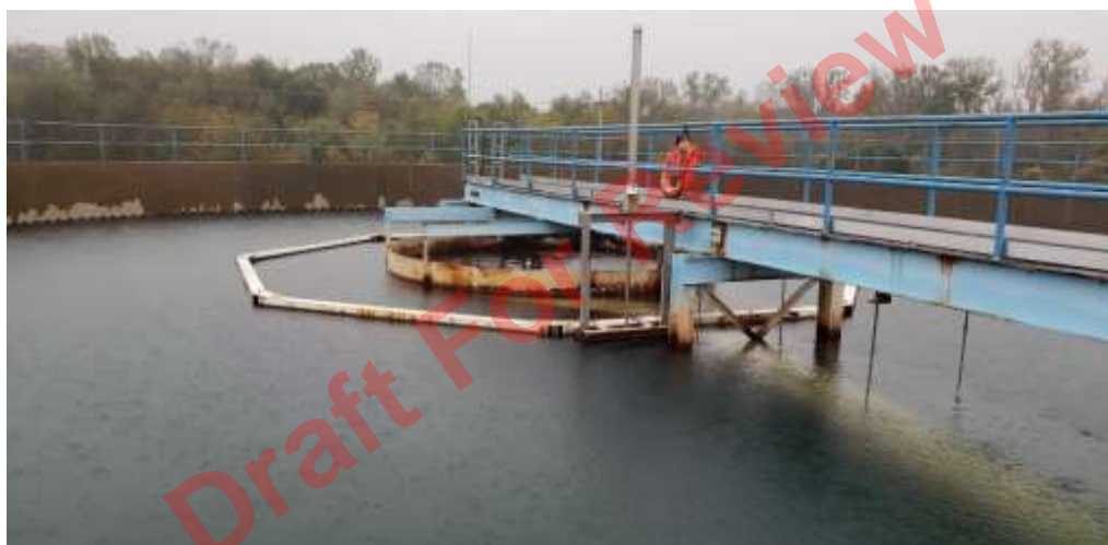
FIGURE 2-12 South Plant Secondary Clarifier
