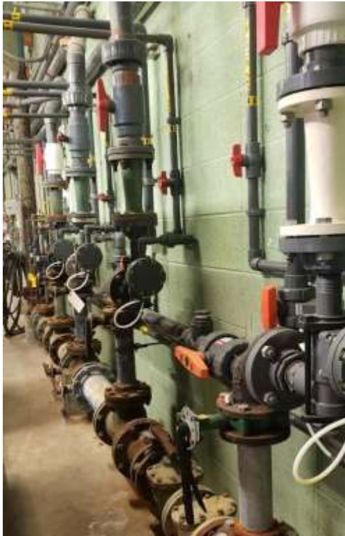
FIGURE 2-23 Chlorine Feed System
