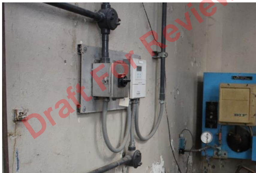
FIGURE 2-16 HSP No. 7's Flow Meter
