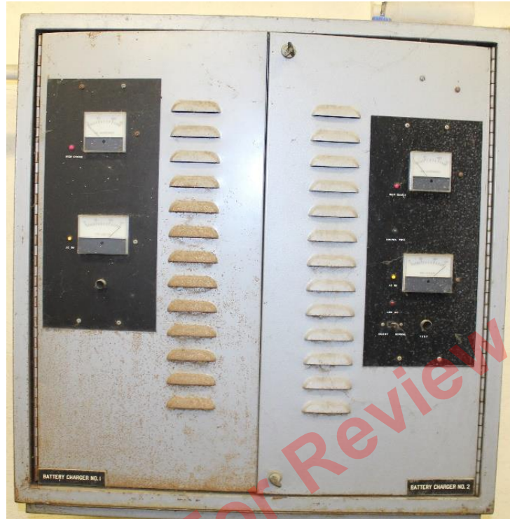
FIGURE 2-3 HSPS No. 3's Battery Backup Charging Station
