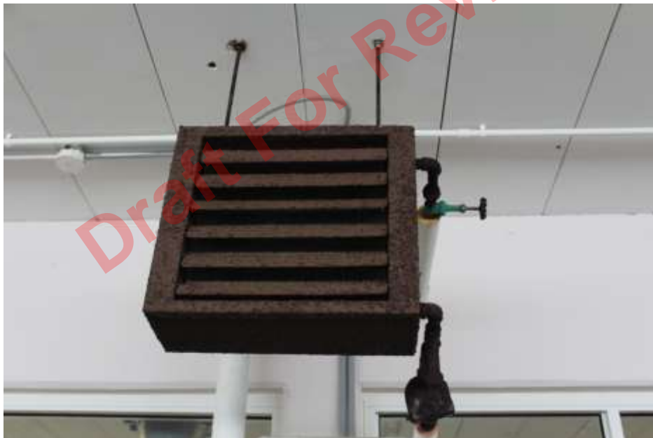
FIGURE 2-32 Unit Heater in South Filter Building
