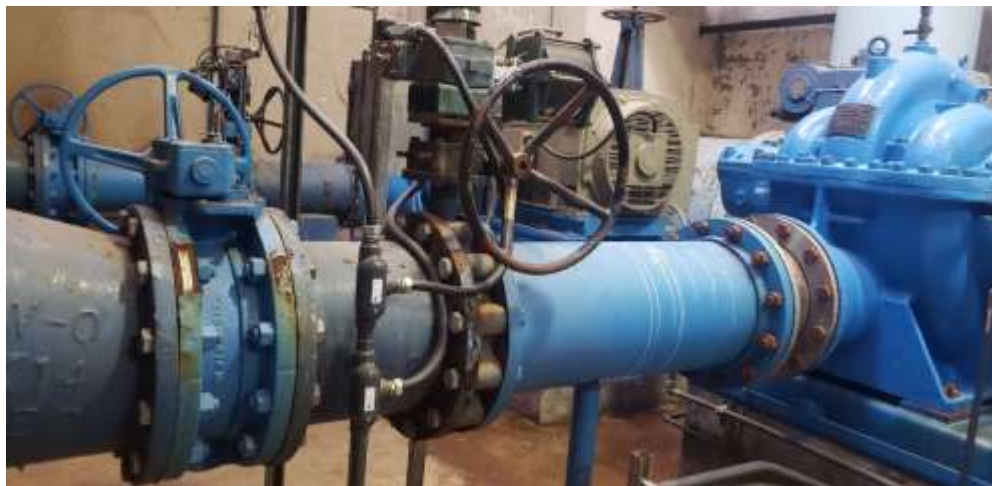
FIGURE 2-27 High Service Pump No. 6
