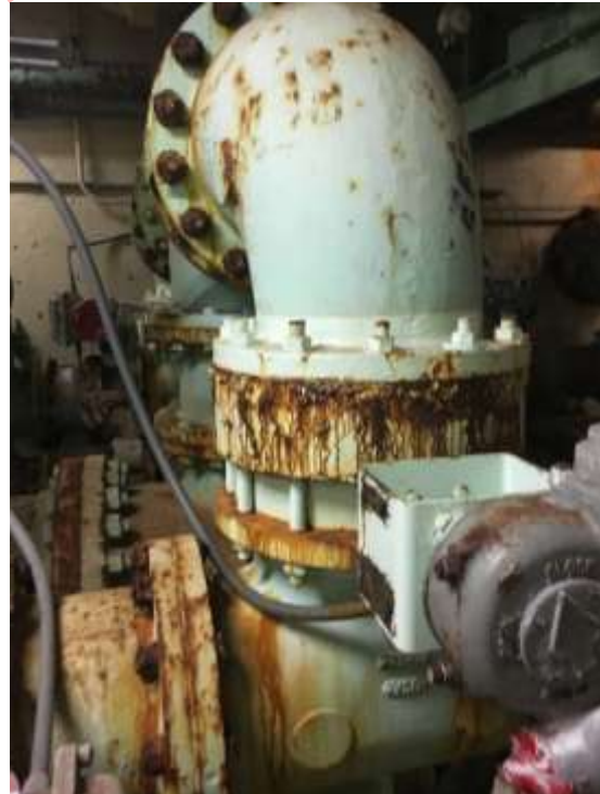
FIGURE 2-16 Corrosion in Pipe Gallery
