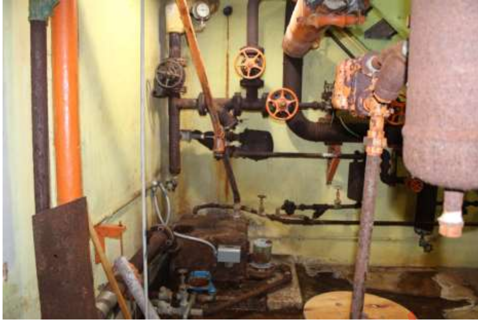
FIGURE 2-31 Condensate Pump and Steam/Condensate Piping in South Filter Gallery
