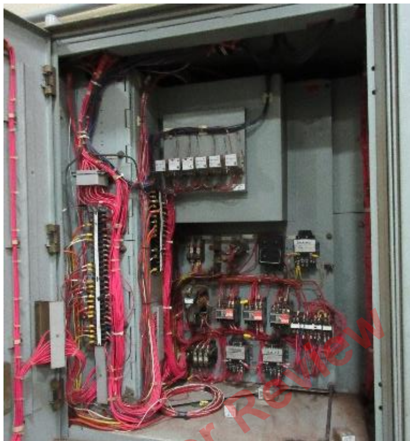
FIGURE 2-7 Low Service Pump Controls
