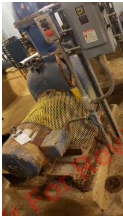
FIGURE 2-13 South Sludge Pump Station Pump Corrosion
