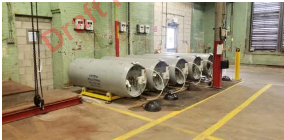
FIGURE 2-22 Chlorine Storage Tanks
