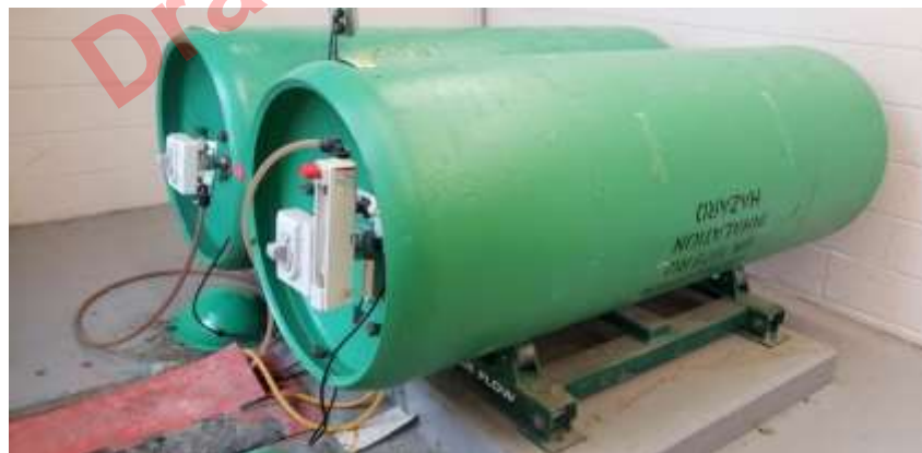
FIGURE 2-25 Sulfur Dioxide Chemical Feed System
