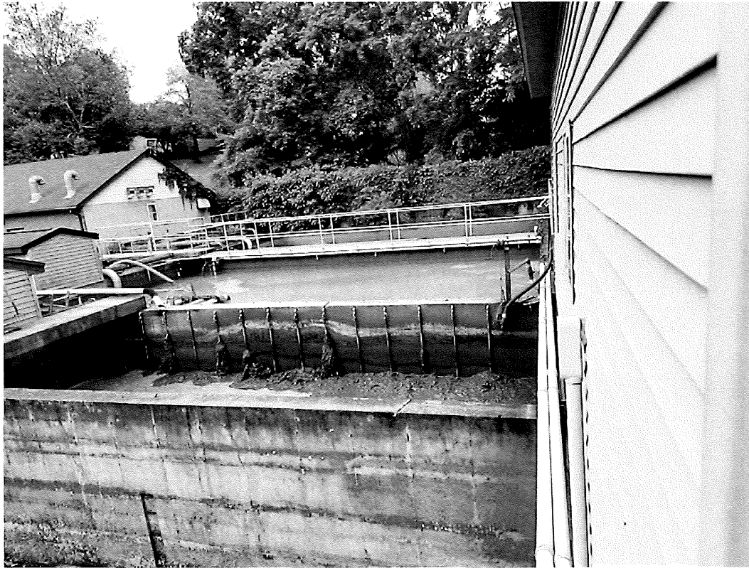
PHOTO 15: AEROBIC DIGESTER AND SBR TANK
