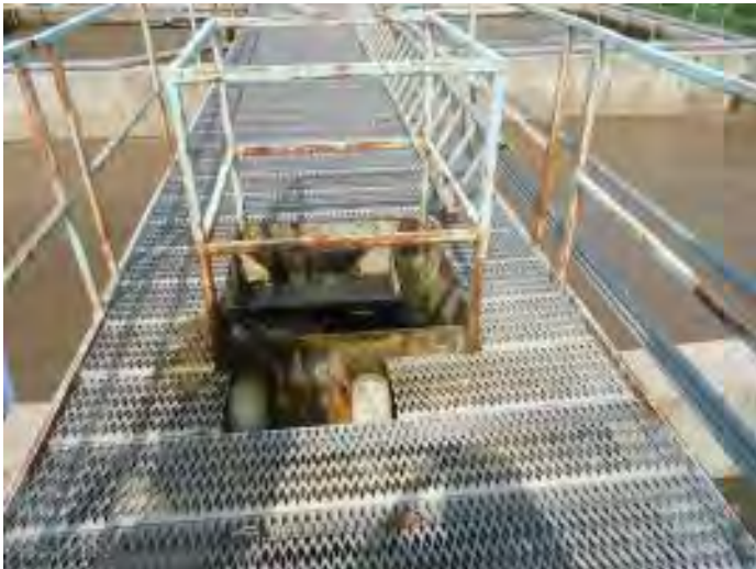
Influent Flow Splitter Box
