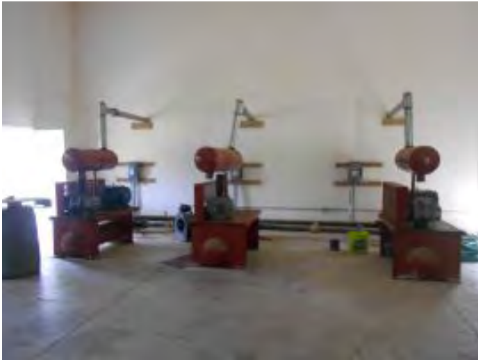
Blower Building Looking East Three of the Five Blowers
