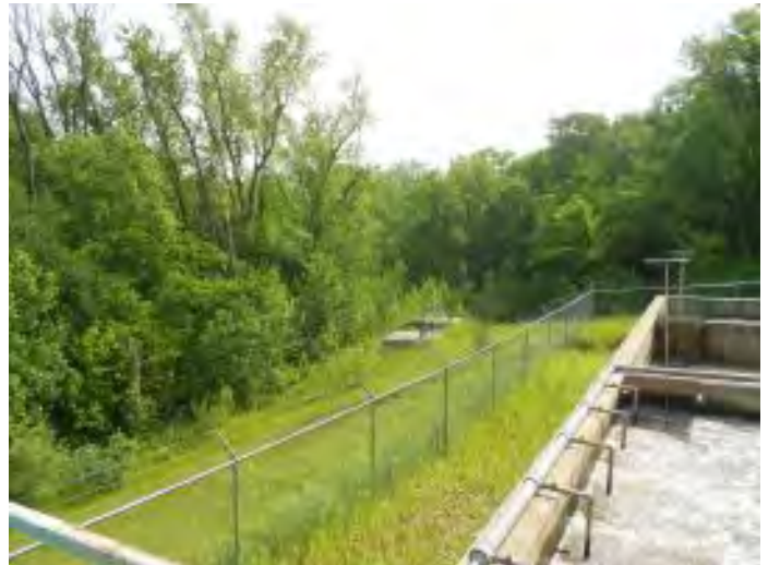
Looking Northeast Towards Influent Pump Station
