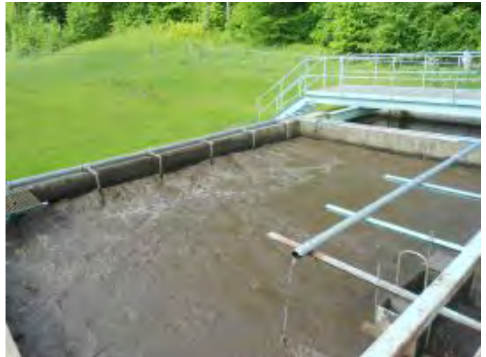
Aeration Tank, One of Two
