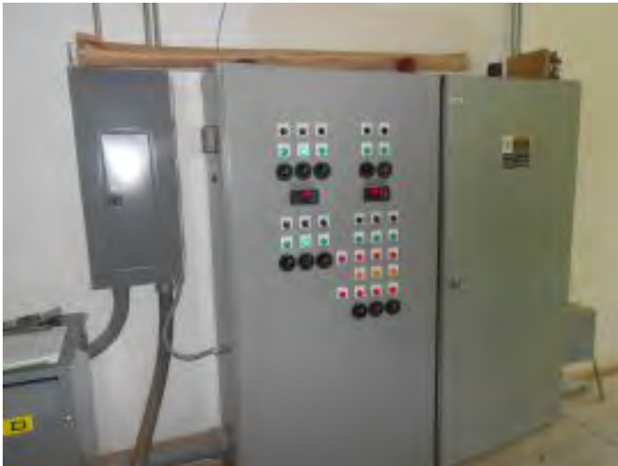
Electrical Gear in Control Building
