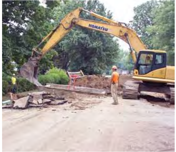
Workers prepare to install new pipe for the Sunset and Kessler STEP project.
