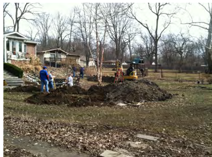
Grinder pump being installed. This view shows the trenching required for a typical installation.
