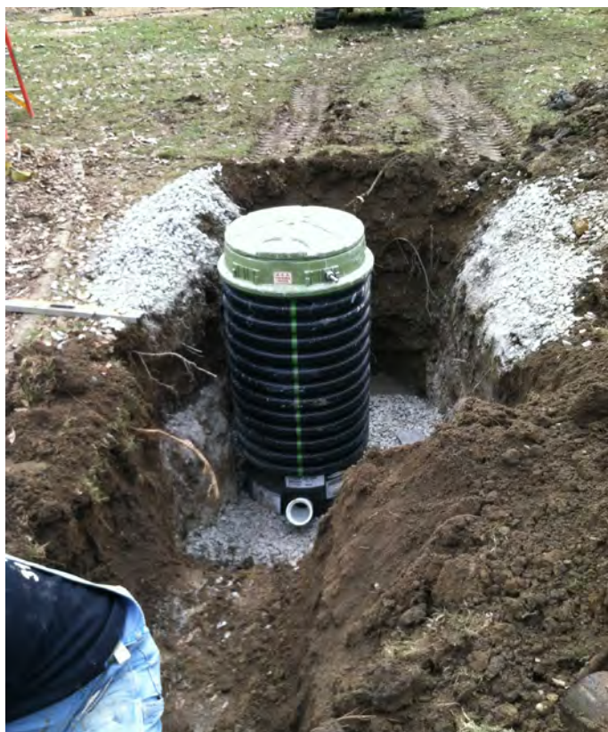
Here is a view of the grinder pump in the trench. This is prior to piping, refilling the trench with soil and leveling of the site.
