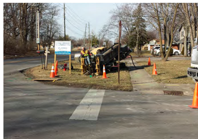
Above: Directional boring machines allow pipe to be installed under streets without the disruptive street cutting and excavation.
