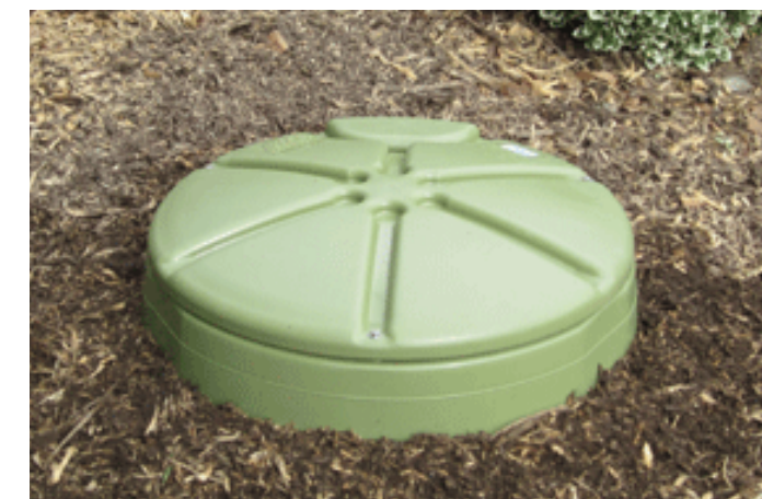
Surface View of the Grinder Pump (post-installation)
