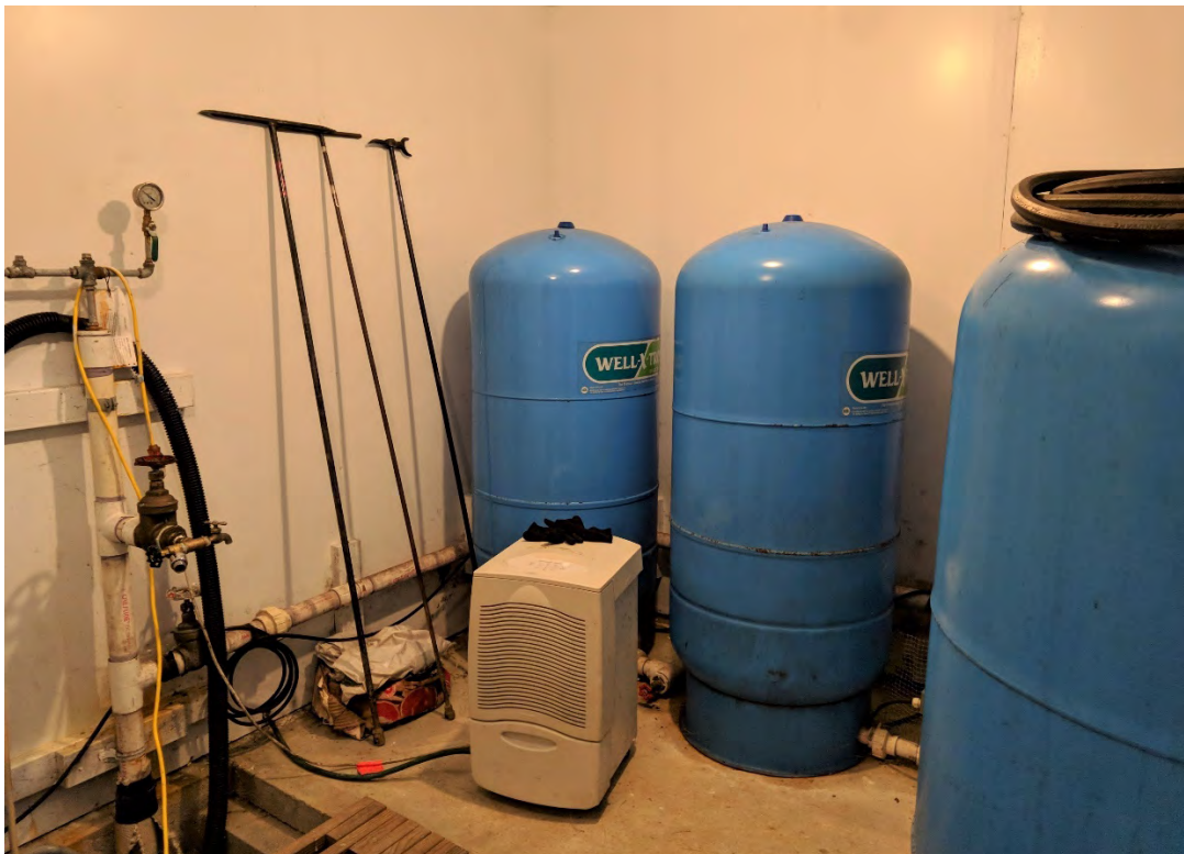
South well house interior, showing 3 of 4 pressure tanks, valve operation keys
