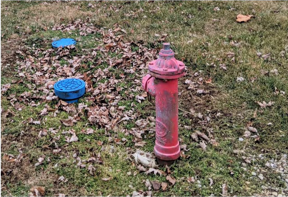
Example of post hydrant, valves near north well structure
