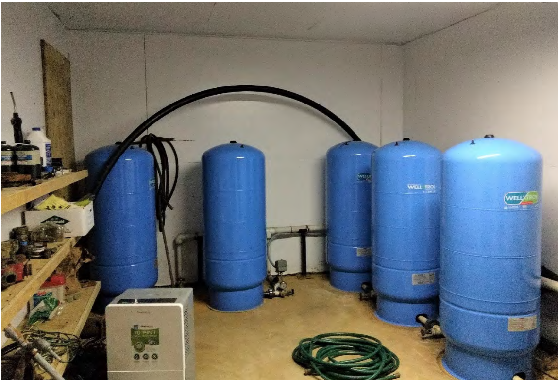
North well house interior
