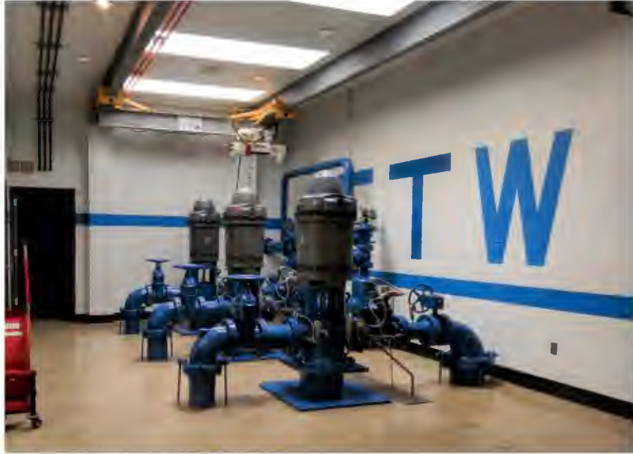
Cedar Grove Plant High Service Pumps
