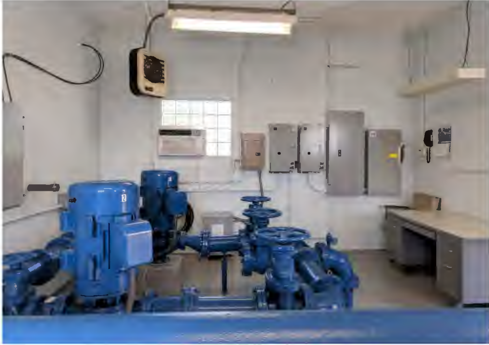
Morgan Road Booster Station pumps
