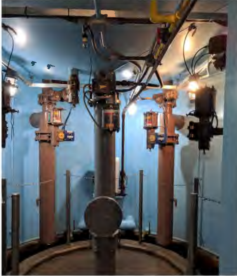
Jamison Road Plant Aerator Interior
