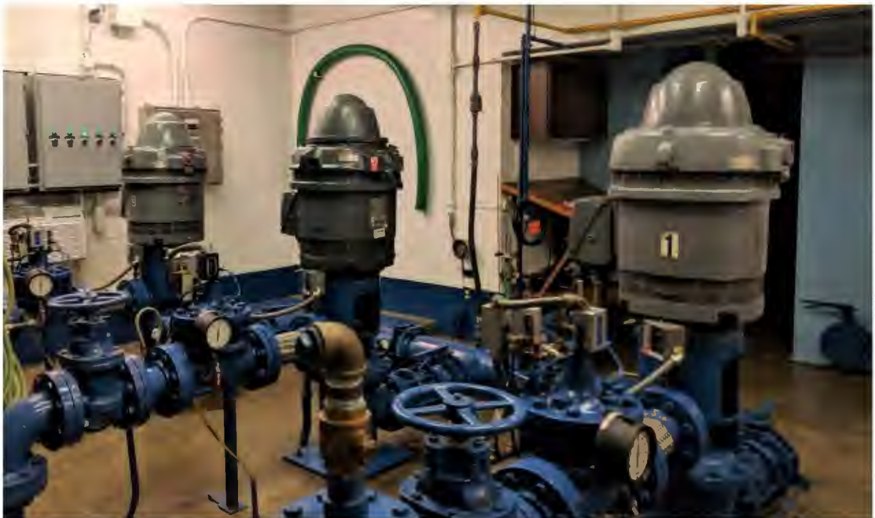
Jamison Road Plant high service pumps
