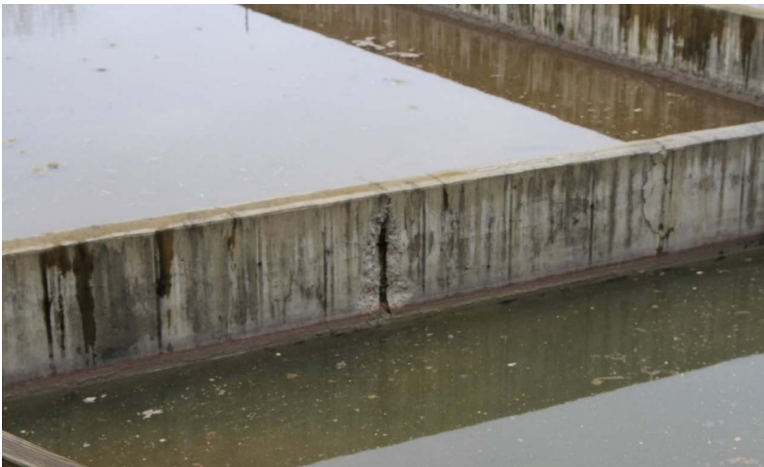
Figure 1 – View of exposed rebar in the west face of CSBR Tank No. 3 baffle wall. OUCC photo taken March 7, 2013.
