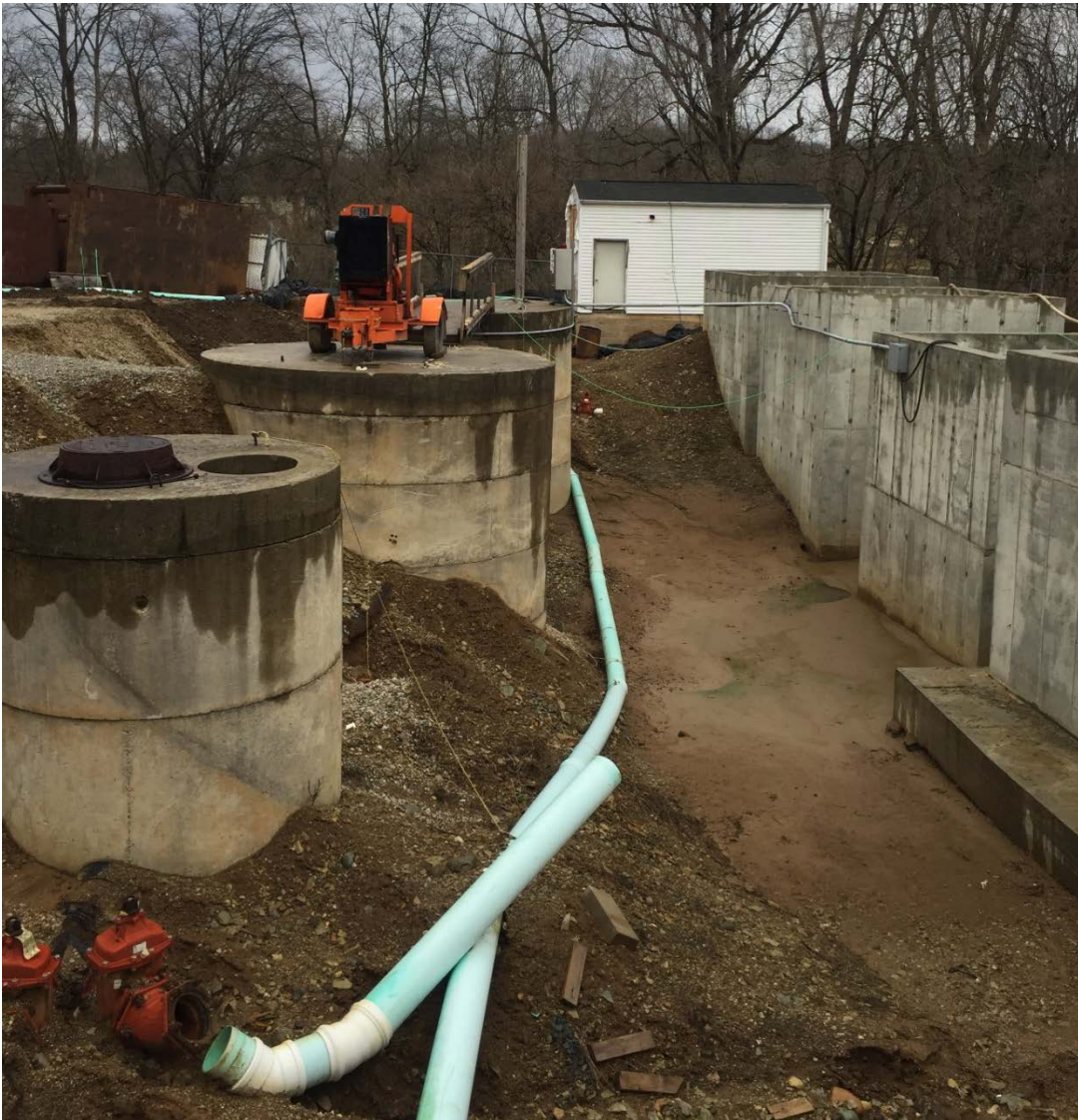
Figure 7 – View of a 6-inch portable trash pump over the existing valve pit at the Carriage Estates WWTP used during high flows. The unfinished Influent Lift Station concrete structures are shown at right. Photo taken by IDEM during the March 13, 2019 inspection. Trash pumps should be unnecessary if headworks was completed as certified by ASU. Note the valve ties into the force main to the existing CSBR tanks in the lower left but there is no connecting discharge pipe from the new lift station.
