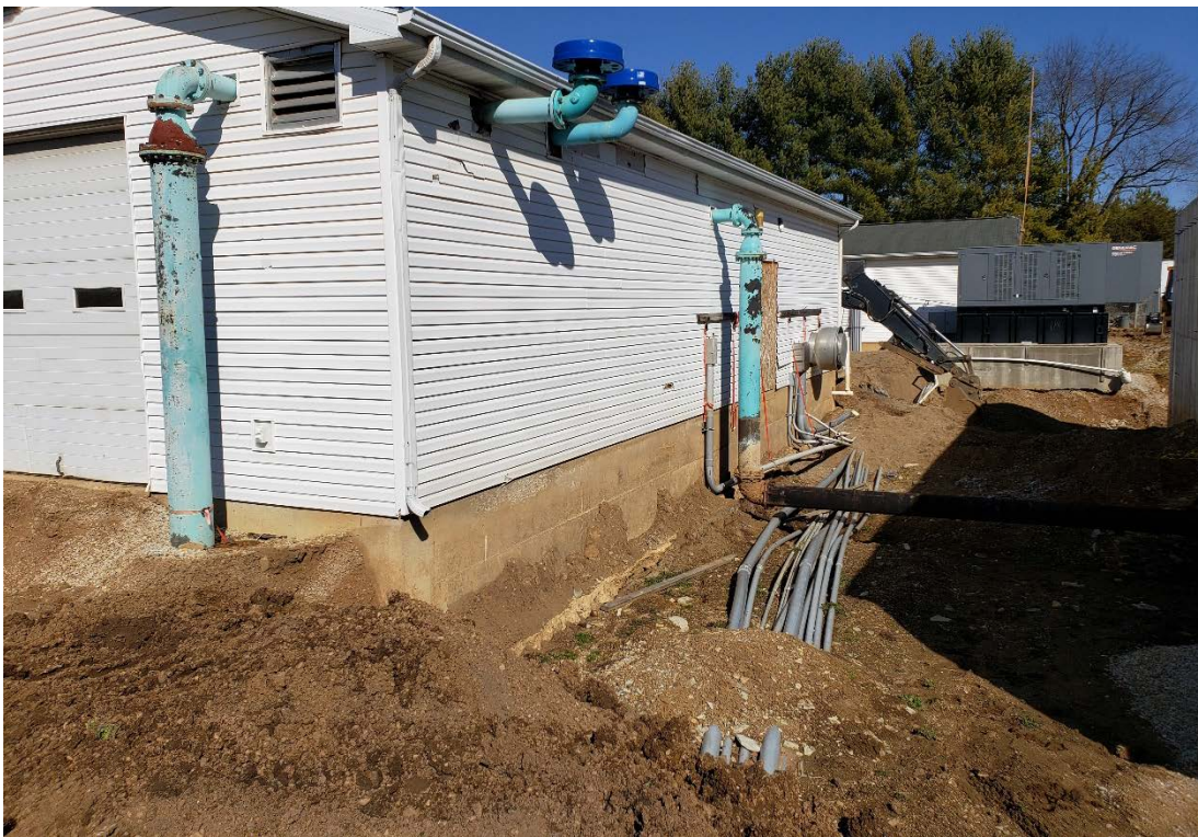
Figure 8 – View of electrical lines in conduits on the east side of the Existing Blower Building. The standby generator and the Control Building are in the background.
