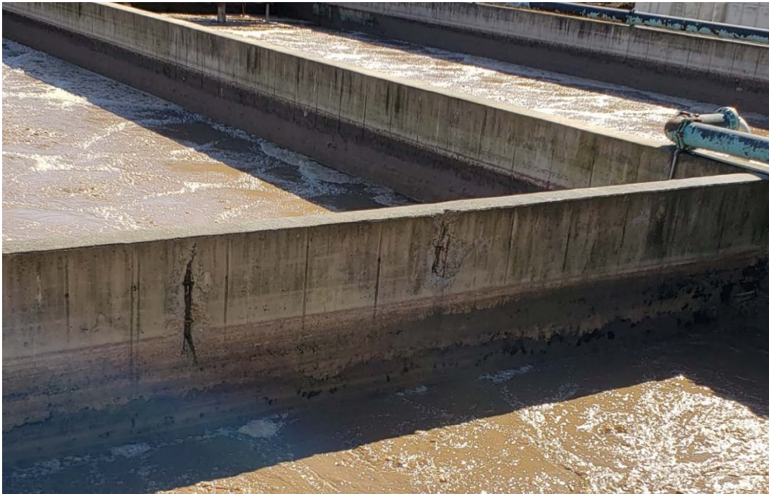
Figure 2 – View of exposed rebar in the same west face of CSBR Tank No. 3 baffle wall. OUCC photo taken March 5, 2020. The spalled concrete ends at the waterline.
