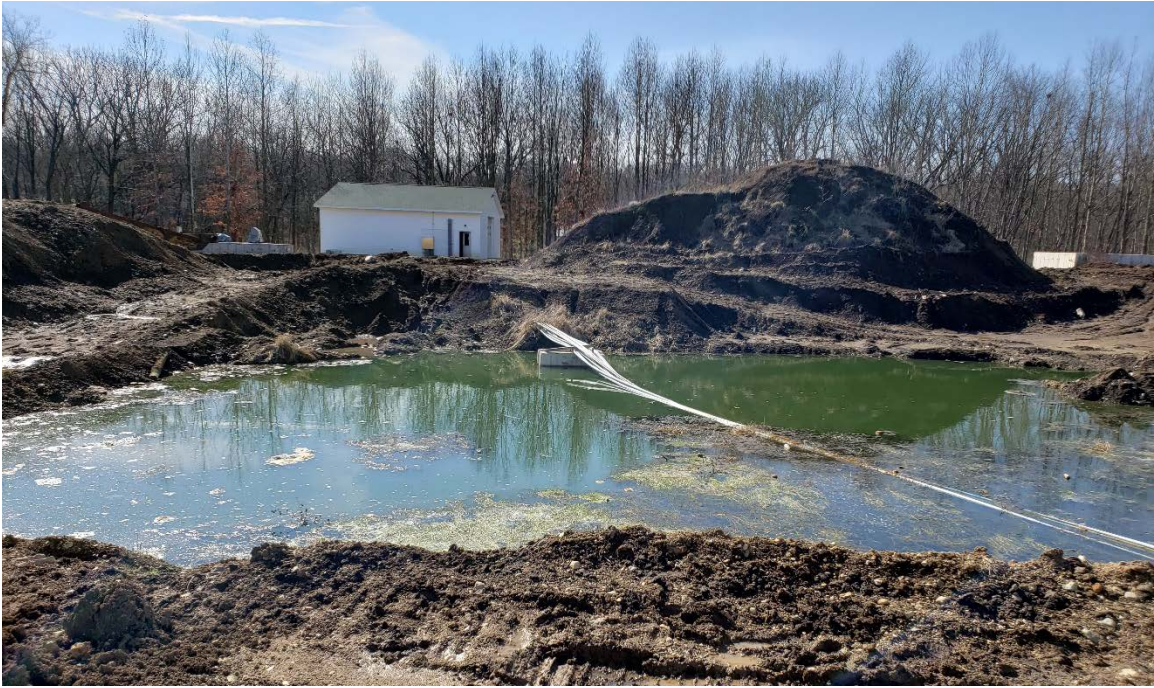
Figure 9 – View south of electrical lines running to the Aeration / UV Control Building.
