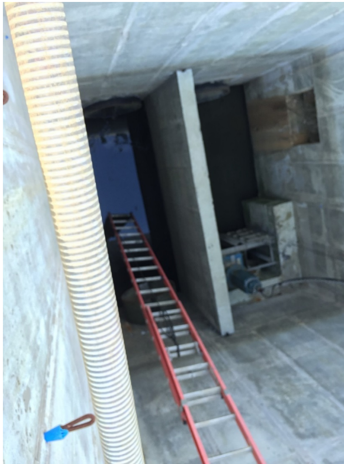
Figure 3 – Interior view of the Macerator structure showing unfinished construction with only one macerator installed (not two), an opening in the north wall but no connecting pipe to the existing Lift Station. Photo taken by IDEM on September 24, 2019.
