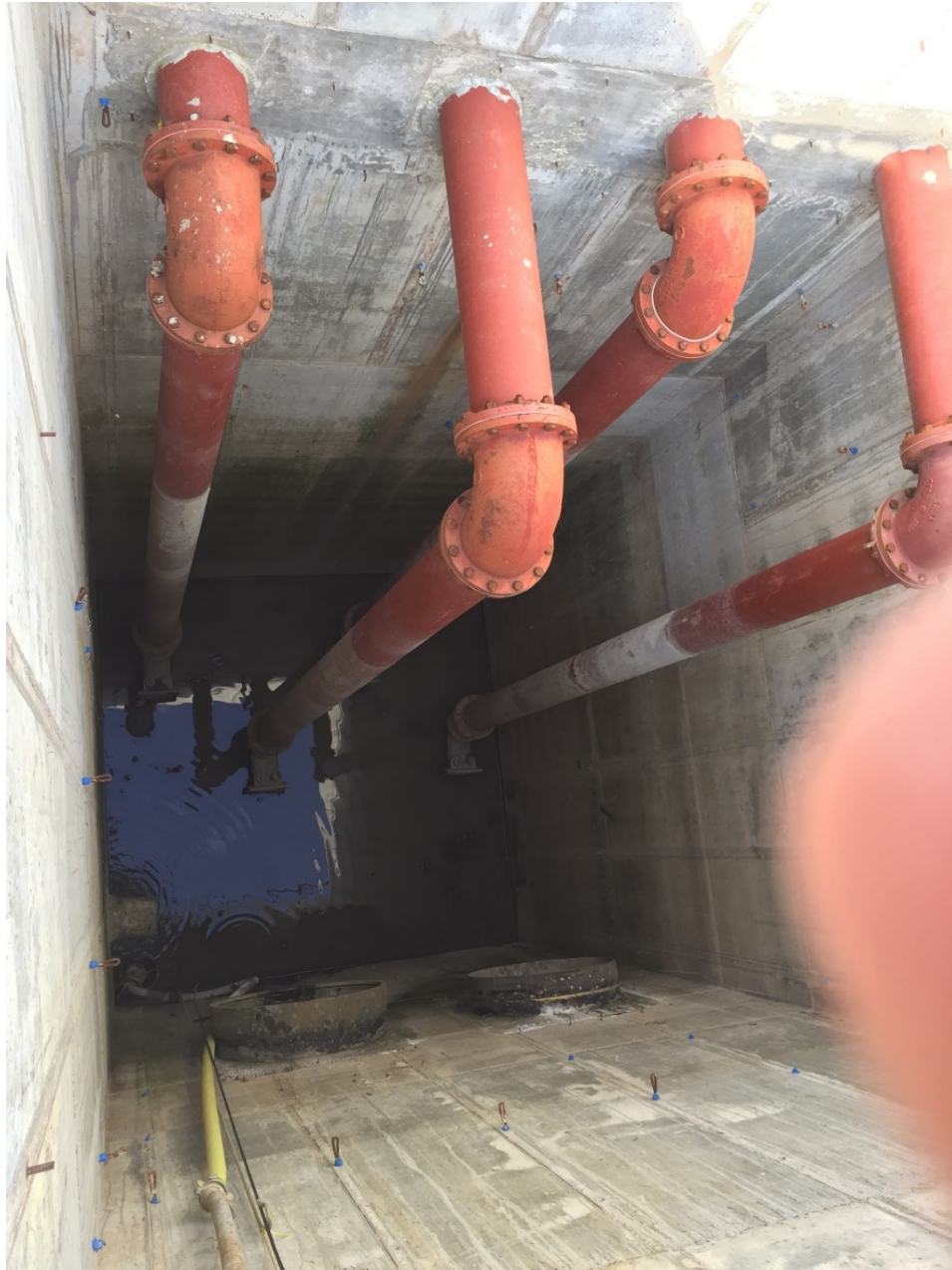
Figure 4 – View of the Influent Lift Station showing no slide rails, no pump controllers, and no pumps installed. Photo taken during IDEM's September 24, 2019 inspection. The grey coloring on the red discharge piping may show the high wastewater mark.
