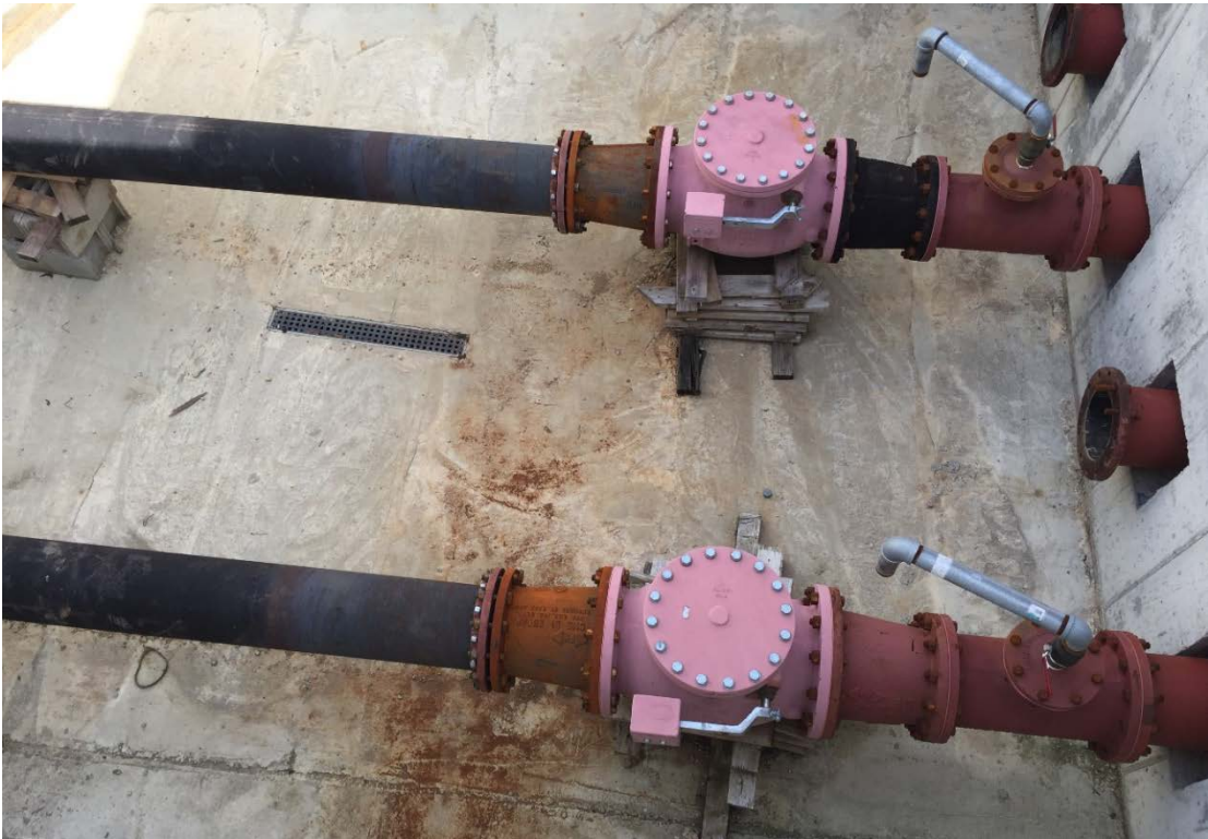
Figure 5 – View showing the incomplete Valve Pit for the Influent Lift Station (missing air release valves, the 6” D.I. Tee bypass pumping connections, the influent flow meters, and the 6” Ball Centric valves) Photo taken during IDEM September 24, 2019 inspection.
