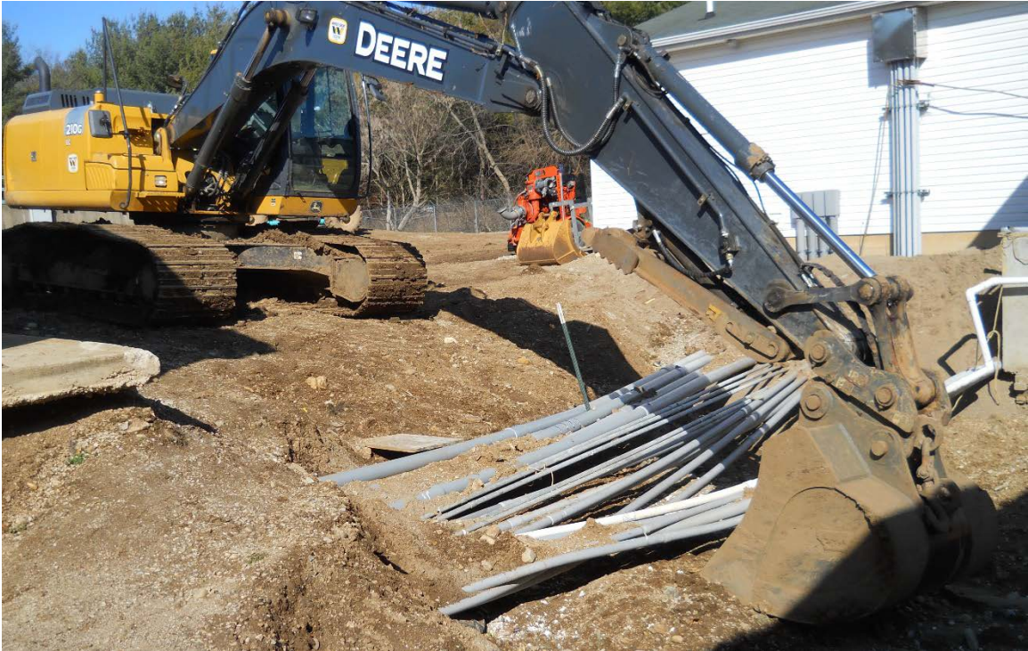
Figure 10 – View of electrical lines from the Control Building which are not in a duct bank.
