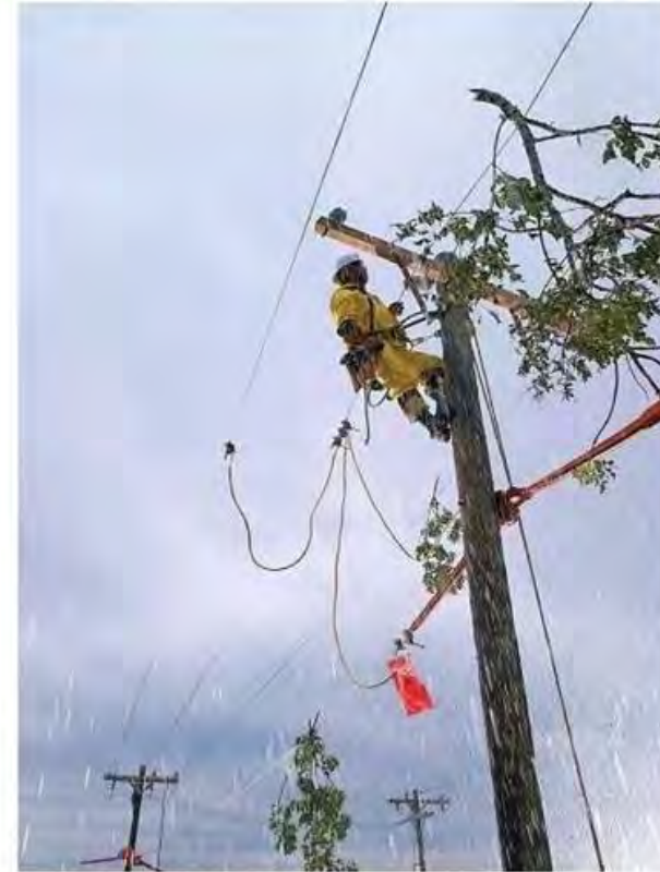
LINEMAN IN RAIN IN AREAS INACCESSIBLE BY BUCKET TRUCK, LINEMEN HAVE TO CLIMB POLES TO MAKE REPAIR.
