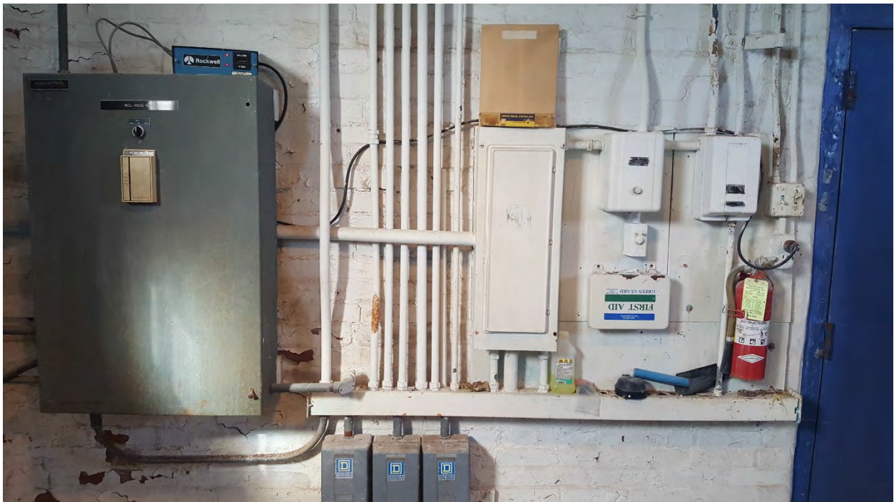
Bloomfield Wellfield Treatment Plant Interior (3)
