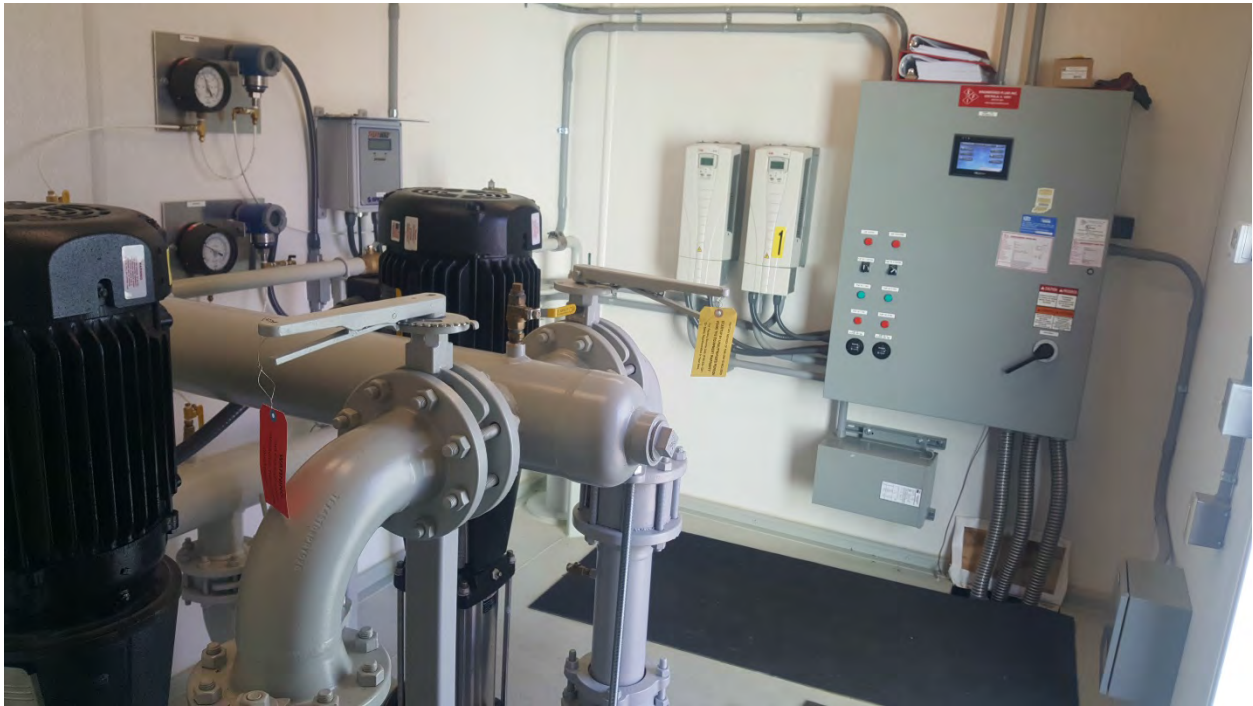
Booster Station #1 Interior
