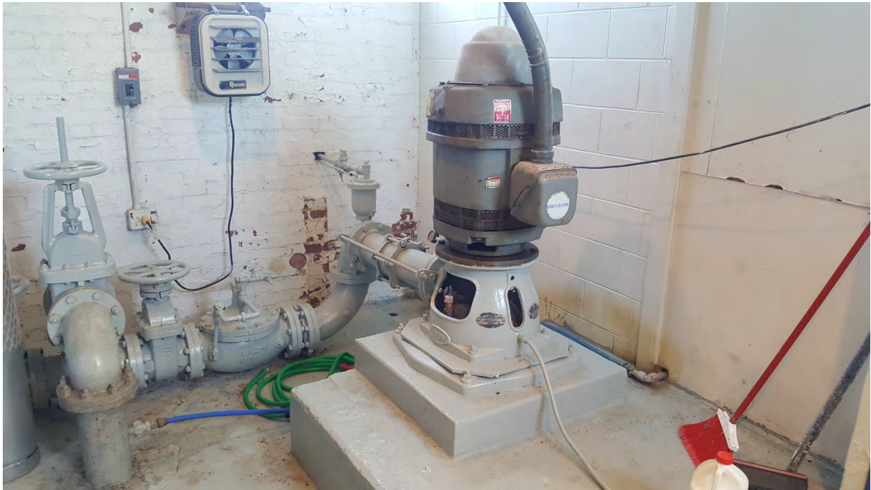
Bloomfield Wellfield Treatment Plant Interior (2)
