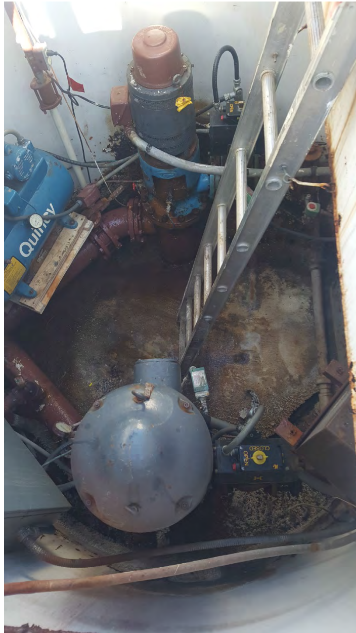
Booster Station #2 Interior
