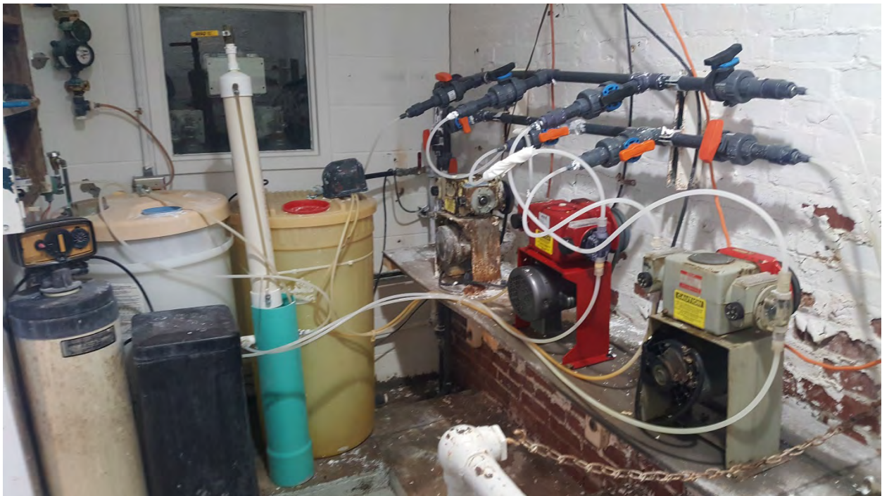
Bloomfield Wellfield Treatment Plant Interior (1)
