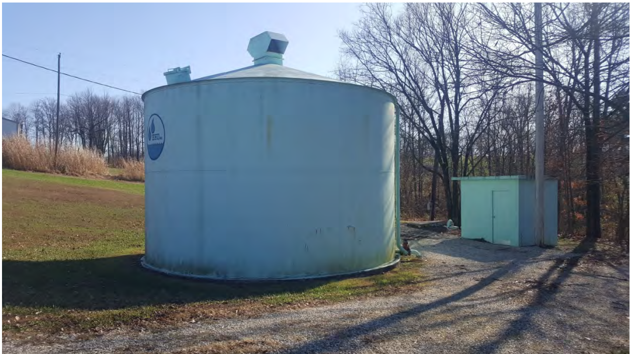
Booster Station #1 Storage Tank - 50,000 gal.
