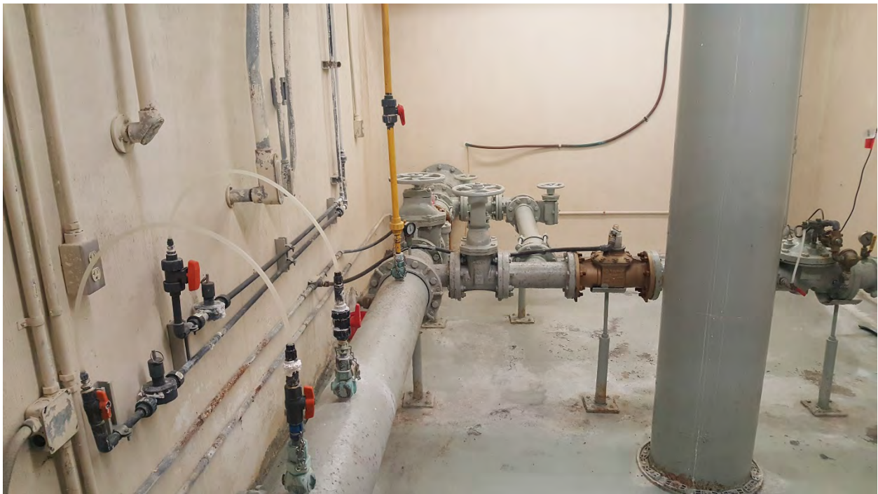
Worthington Wellfield Treatment Plant Interior (2)
