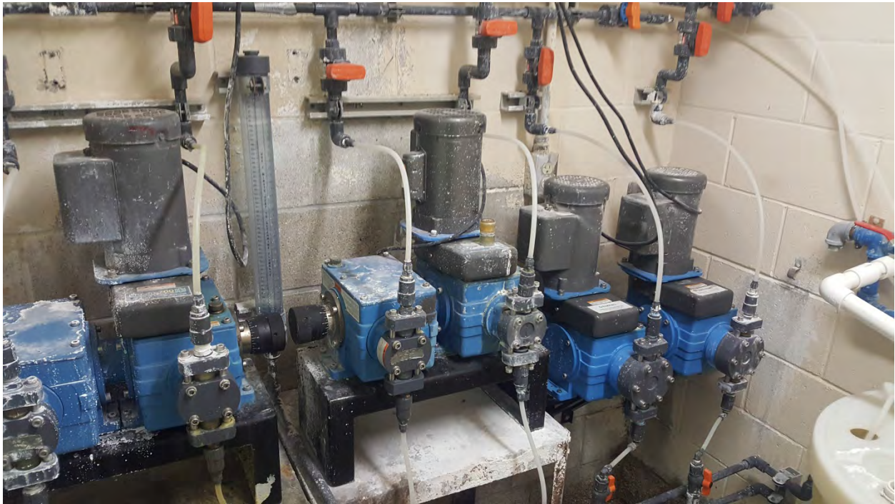
Worthington Wellfield Treatment Plant Interior (1)
