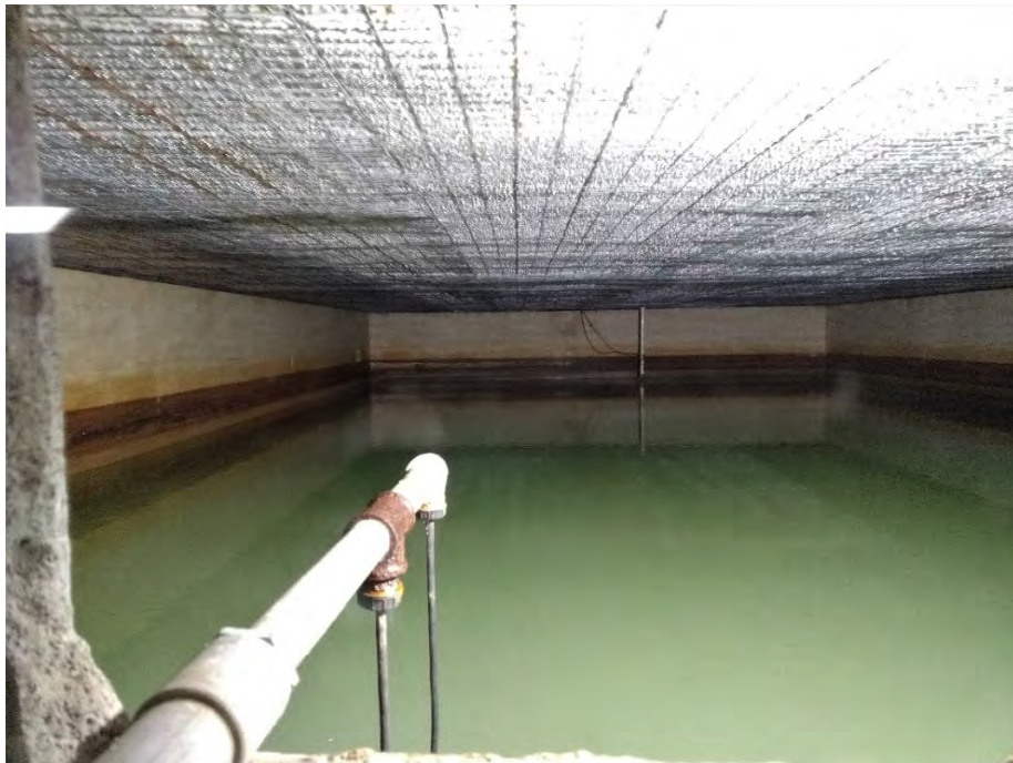
70,000 gallon concrete storage tank in plant
