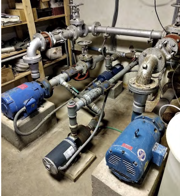
High service pumps, unit in rear is single-phase for generator
