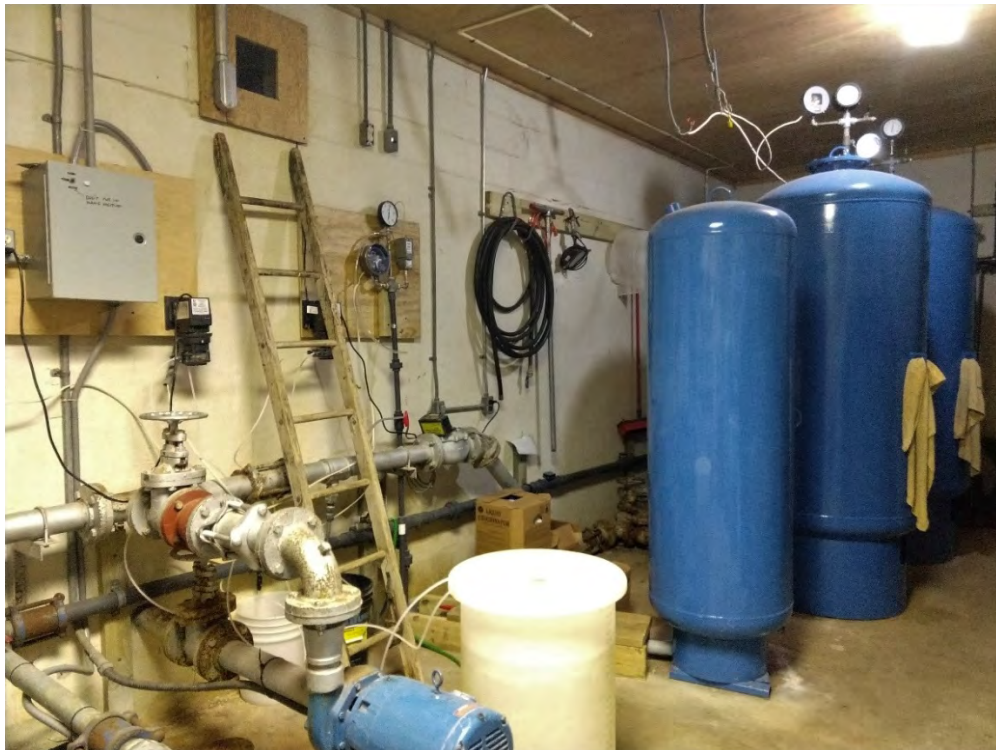
Plant interior showing high service pumps (lower left) and pressure tanks (right)
