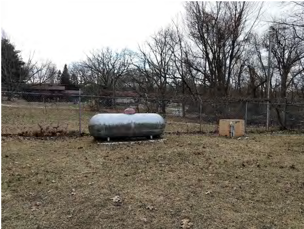
Backup generator and propane storage tank
