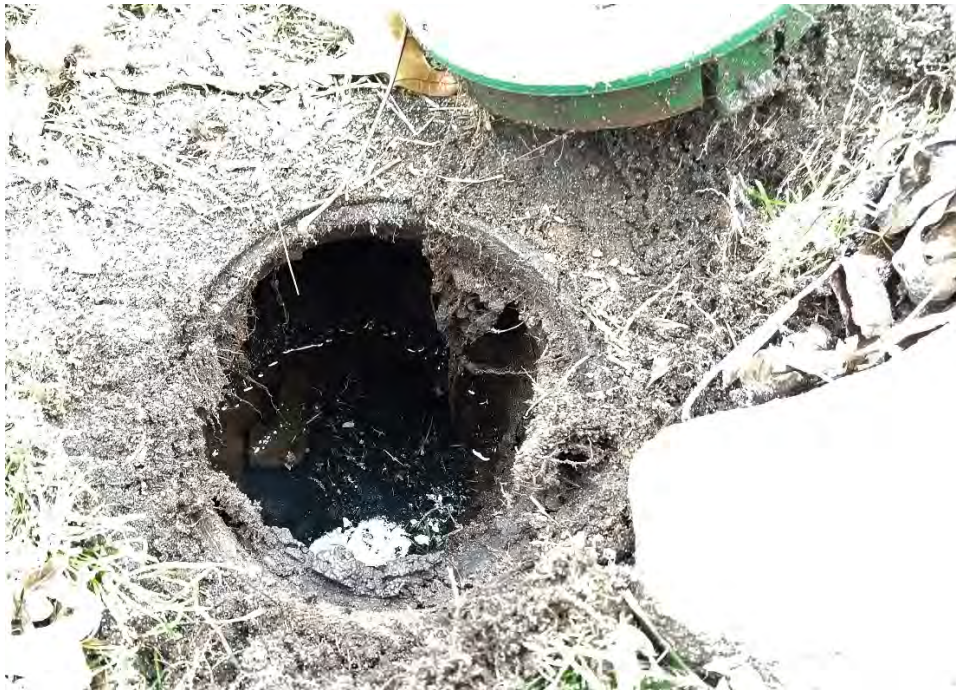
First leaking valve, note water in riser
