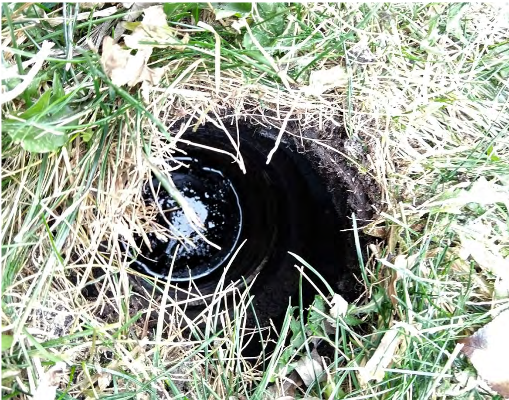
Third leaking valve identified
