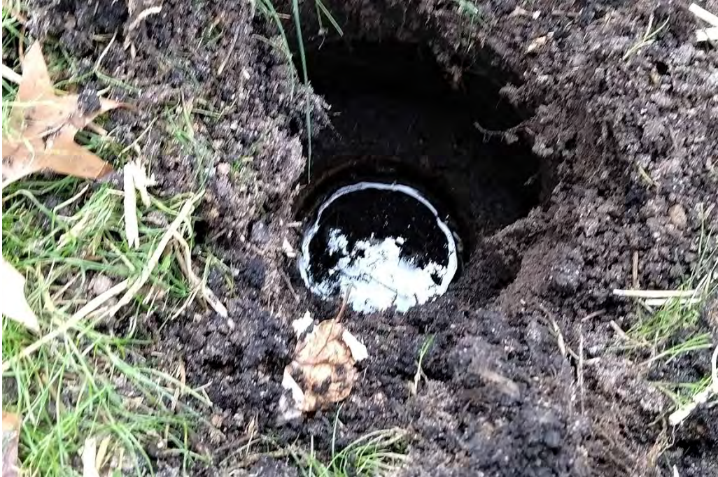
Second leaking valve uncovered
