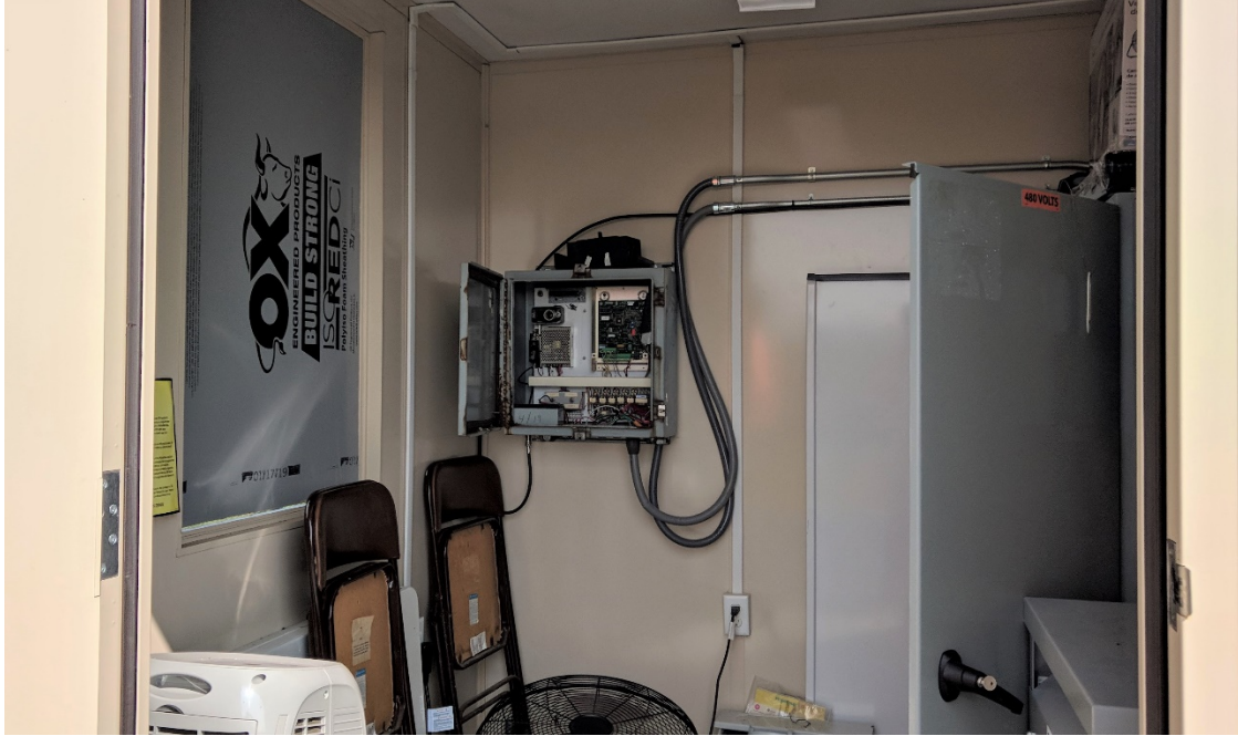
New well control building interior
