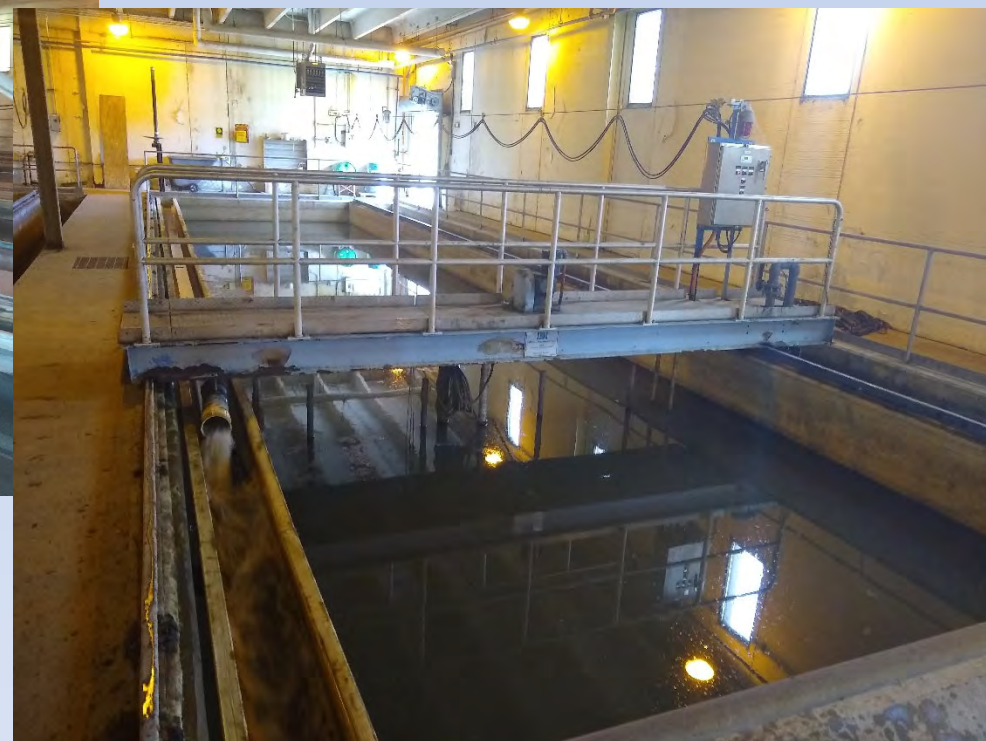
6 Automatic backwash filters with traveling bridges
