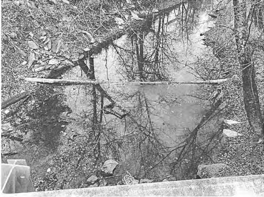
Exposed 8" PVC Water Main at Creek Crossing to be Addressed by Alternative 8
